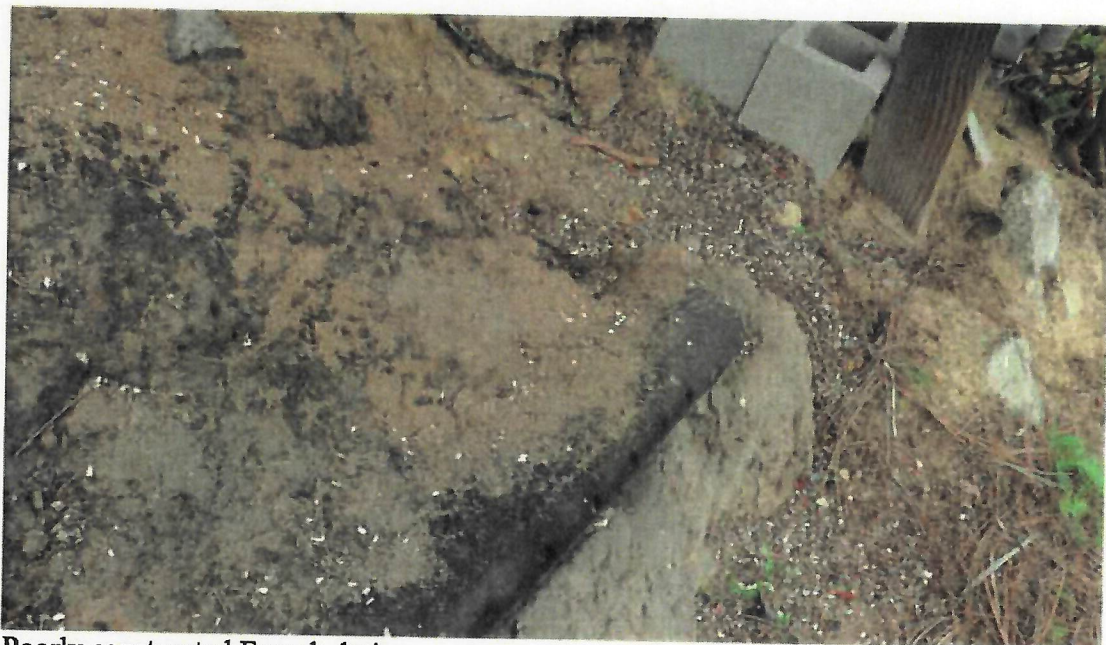
Poorly constructed French drain
