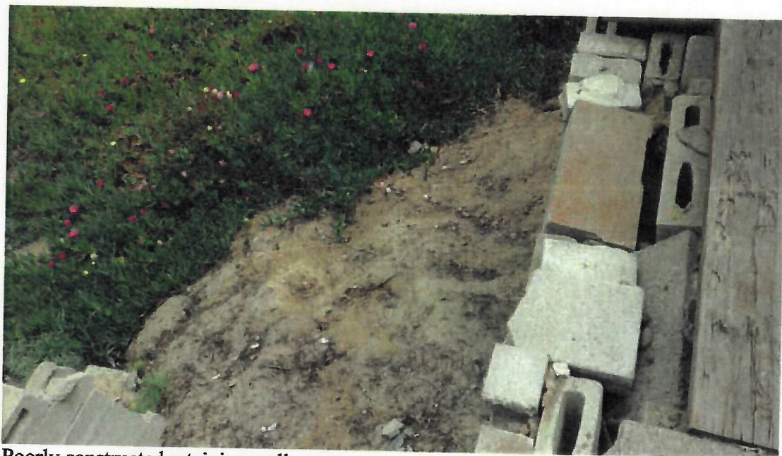
Poorly constructed retaining wall
