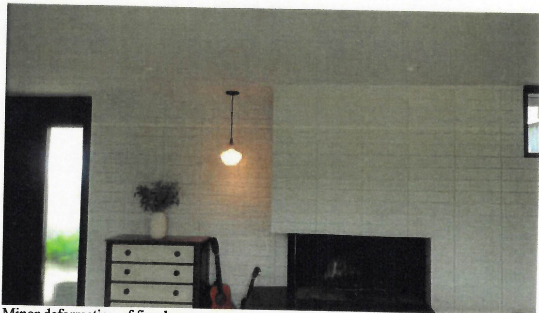
Minor deformation of fireplace area
