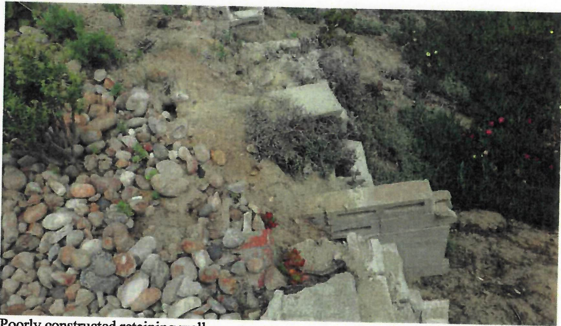
Poorly constructed retaining wall
