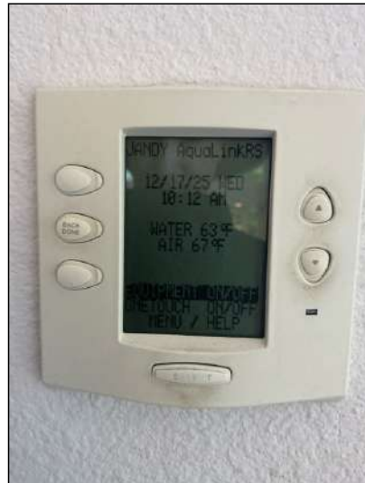
Pool equipment was tested with wall control, located on dining room wall.
