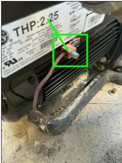
Pool pump is electrically bonded/grounded.
