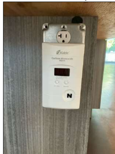
First floor carbon monoxide detector
