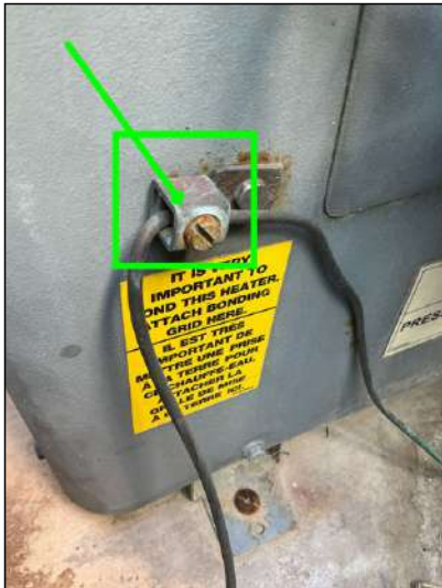
Pool heater is electrically bonded/grounded.
