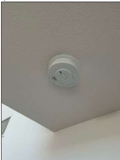
First floor smoke detector
