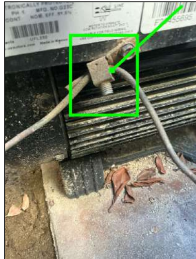
Pool pump is electrically bonded/grounded.
