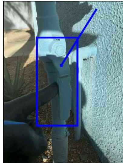
Main water shut of valve. Location: south exterior garage wall
