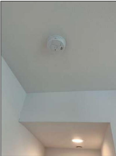
Second floor smoke detector
