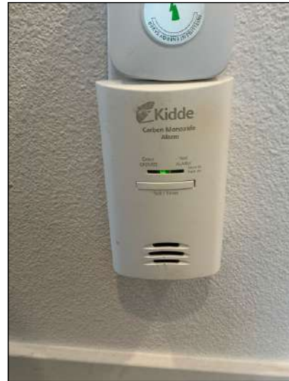
Second floor carbon monoxide detector
