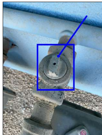
Main gas shut off valve. Location: west exterior wall
