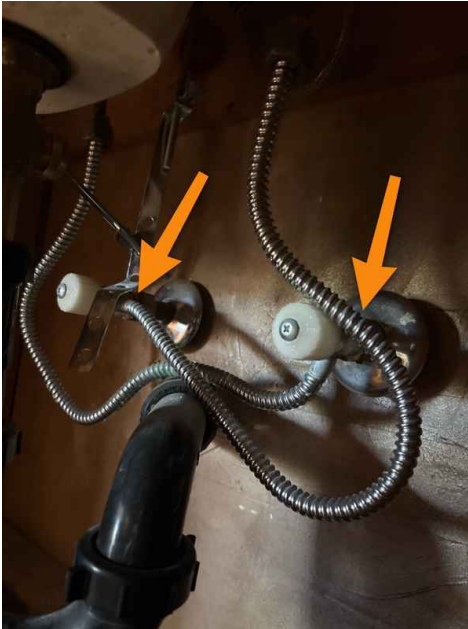
Example Primary Bathroom
