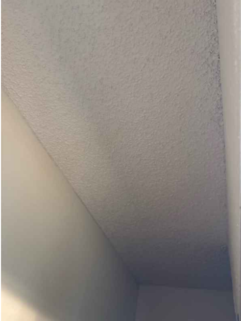
Example Primary Bathroom
