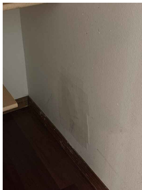
Example Primary Bathroom
