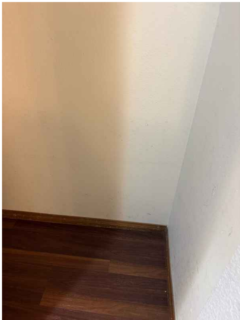
Example Primary Bathroom
