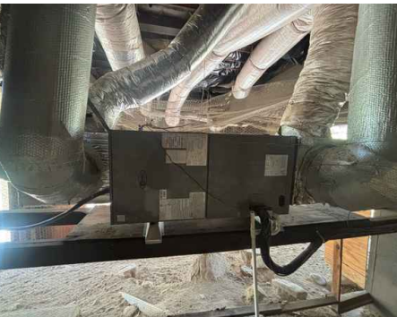
Photo of heat pump
