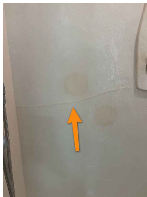
Example Primary Bathroom
