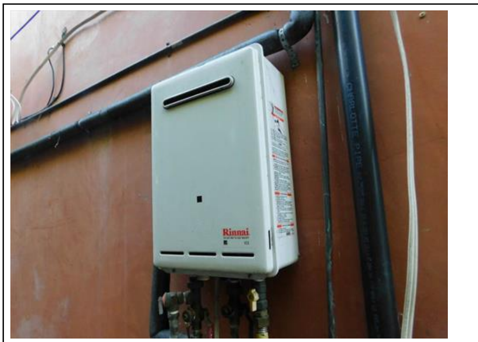
TANKLESS WATER HEATER FOR GUEST HOUSE
