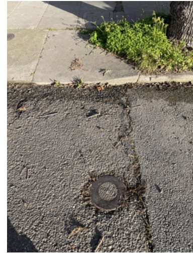
Valve at street before meter
