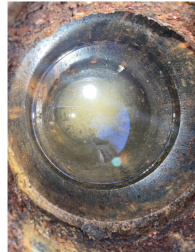
Street valve looks to be buried and cover with water.
