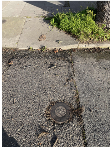
Valve at street before meter
