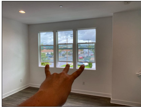
Missing screens - all
