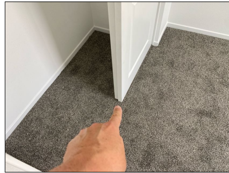
Bypass door guides missing at base - needs to be serviced - both guest bedrooms
