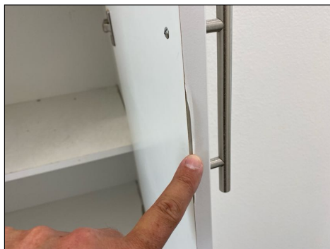
Delamination present on Cabinet doors – service needed
