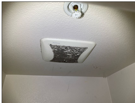
Extremely Dirty/dusty unit - recommend cleaning
