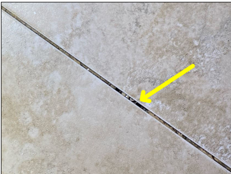
Cracked/loose/missing grout in areas - recommend grout and sealer maintenance
