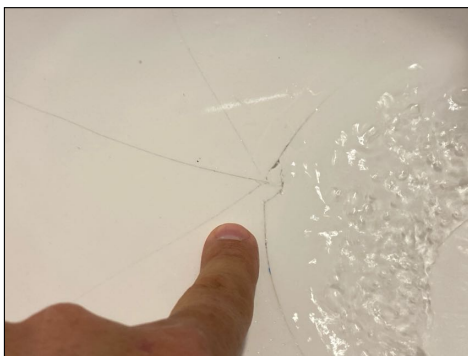
Cracked sink - needs to be serviced - bathroom off kitchen
