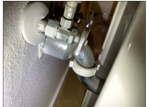
Older style metal traps present - traps can leak at any time due to corrosion
