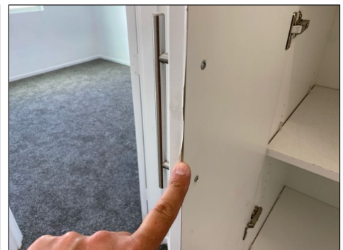
Delamination present on Cabinet doors – service needed
