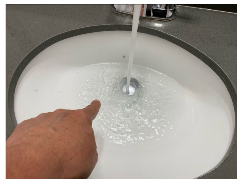
Drain operated slowly - needs to be serviced - bottom floor
