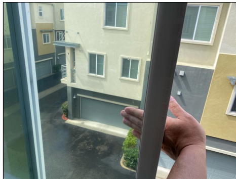
Missing screens - ALL - recommend installation of an appropriate screen
