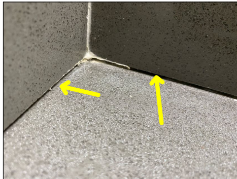
Gap at backsplash to countertop joint - needs to be serviced - top floor hallway bathroom
