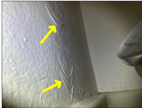
Peeling/blistered/cracking paint in areas - top floor hallway bathroom
