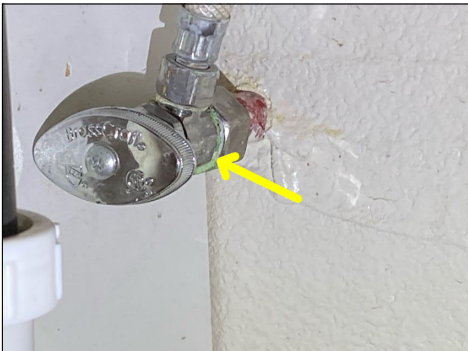
Shutoffs under sink corroded - needs to be serviced - this will be an ongoing maintenance issue for ALL plumbing valves
