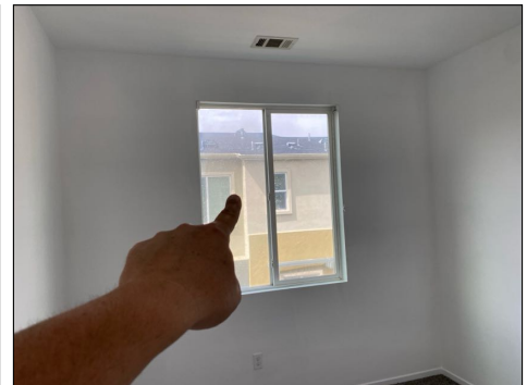
Visible internal condensation or hazy glass inside window - needs to be serviced/evaluated by a window contractor - recommend all windows be checked as others may exist
