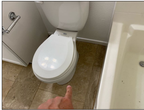
Toilet loose at floor - needs to be serviced - all toilets except ground floor
