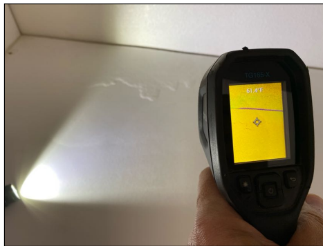
Stained areas below sink - dry at time of inspection
