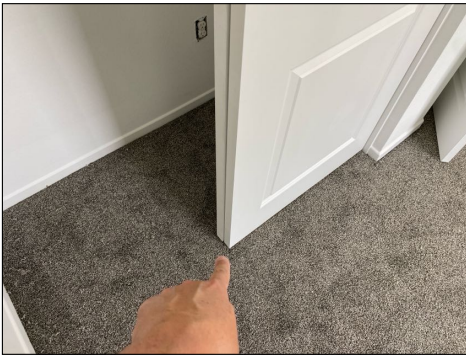
Bypass door guides missing at base - needs to be serviced - both guest bedrooms
