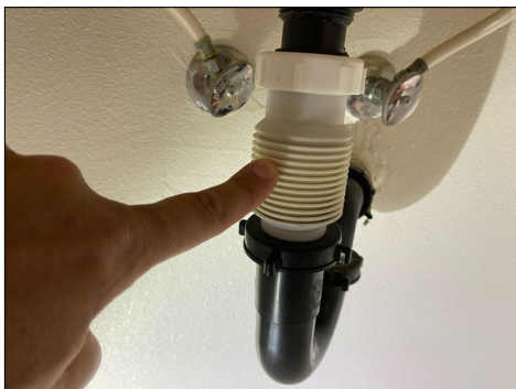
Plastic flex line used on bathroom sink drain - this material is considered weak and should be upgraded for optimum long term drainage
