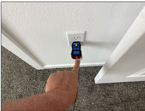
Three prong outlet(s) not grounded - needs to be serviced - master
