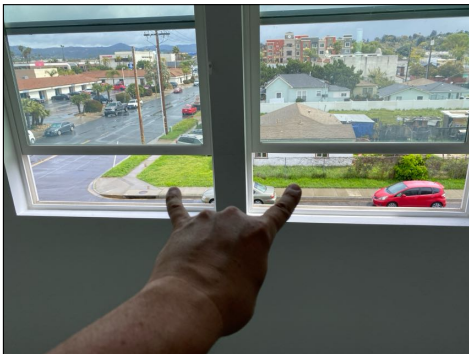
Missing screens - ALL - recommend installation of an appropriate screen
