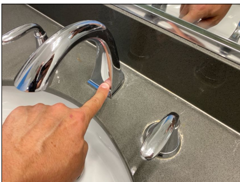
Loose fixture/handles - needs to be serviced - bottom floor bathroom and master
