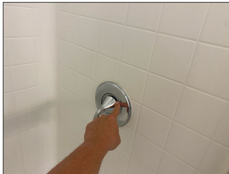
Plumbing loose in wall - needs to be serviced - master
