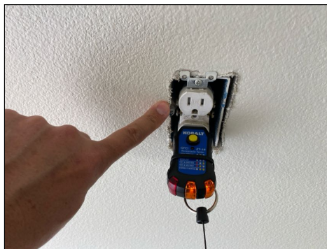
Outlet cover missing - needs to be serviced
