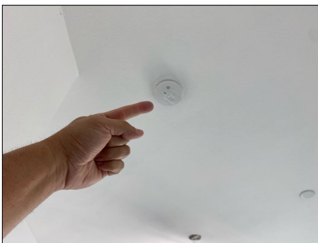
Worn/older model suggest replacement with modern devices - ALL
