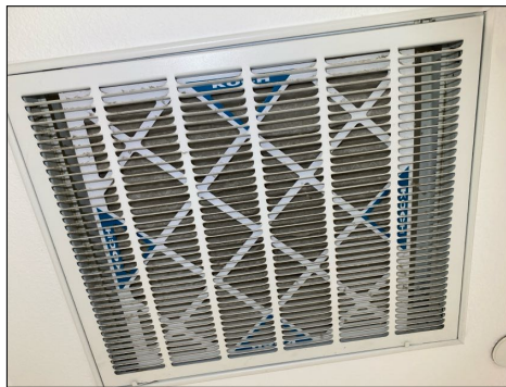
Filter is worn/dirty and will likely need changing soon
