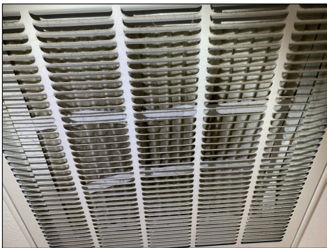
Filter is worn/dirty and will likely need changing soon
