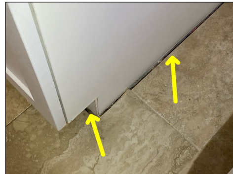
Open seams/gaps in areas - recommend sealing any cracks or voids in flooring
