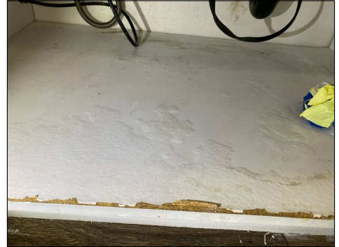
Stained/blistered area(s) - tested dry at time of inspection - monitor area for moisture
