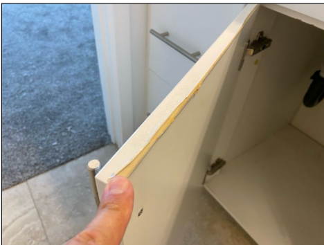
Delamination/moisture damage in some areas - needs to be serviced
