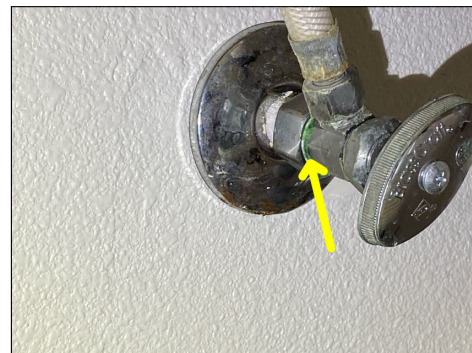
Shutoffs under sink corroded - needs to be serviced - this will be an ongoing maintenance issue for ALL plumbing valves
