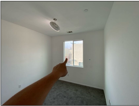
Visible internal condensation or hazy glass inside window - needs to be serviced/evaluated by a window contractor - recommend all windows be checked as others may exist
