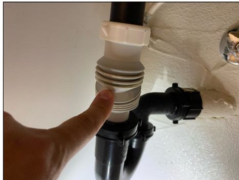
Plastic flex line used on bathroom sink drain - this material is considered weak and should be upgraded for optimum long term drainage
