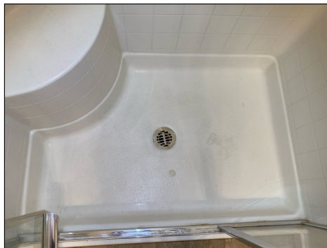
Shower pan is in a worn/stained/older condition - typical for the age
