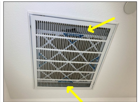
Wrong size - needs to be replaced
