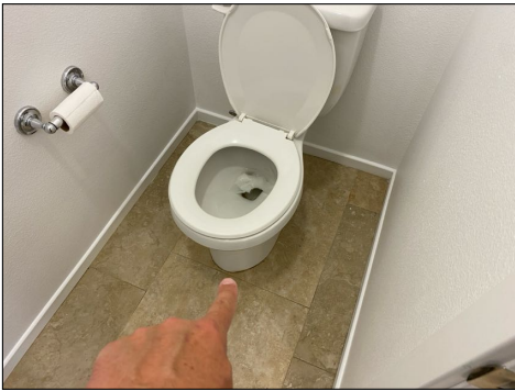
Toilet loose at floor - needs to be serviced - all toilets except ground floor
