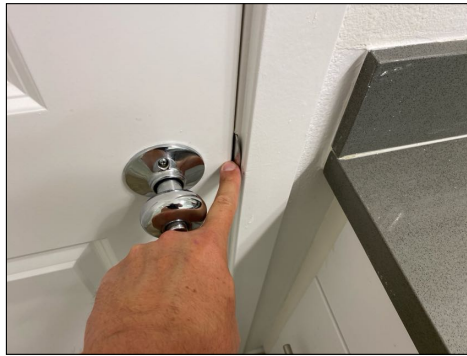
Did not latch properly - needs to be serviced - master
