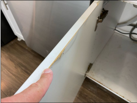
Delamination occurring in multiple areas – service needed
