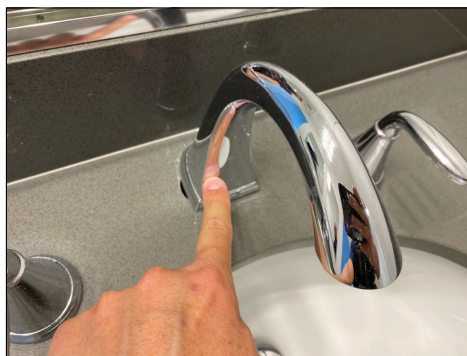
Loose fixture/handles - needs to be serviced - bottom floor bathroom and master
