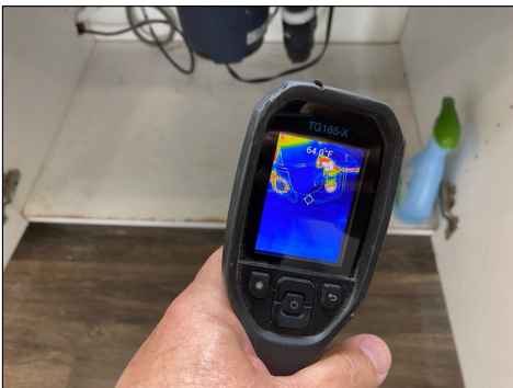
Stained/blistered area(s) - tested dry at time of inspection - monitor area for moisture
