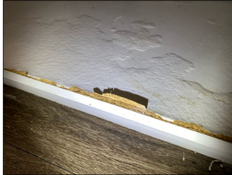
Delamination occurring in multiple areas – service needed
