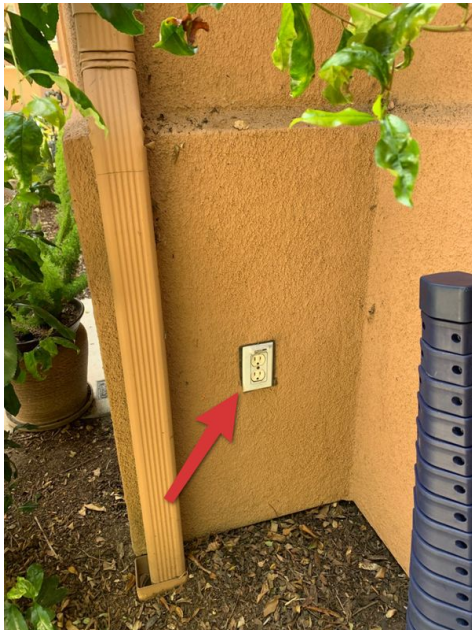
Example Noted at front door
