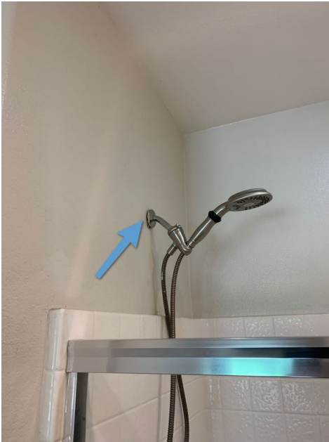
Example Noted at Master Bathroom
