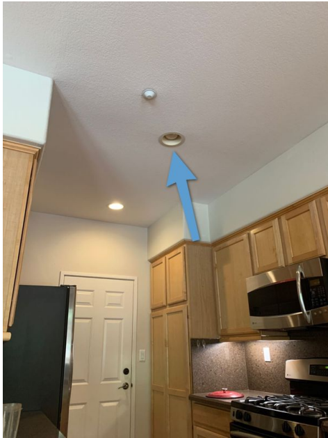
Example Noted at Kitchen
