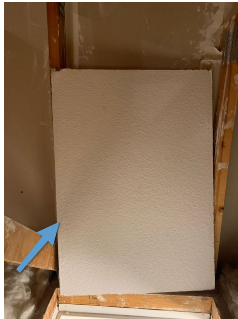
Example Noted at Attic
