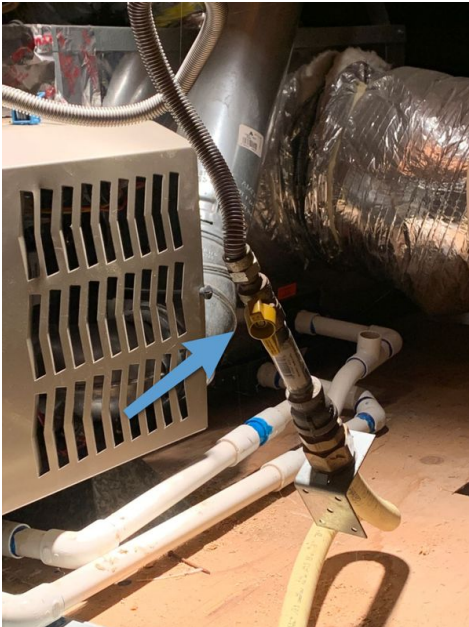
Example Noted at Furnace
