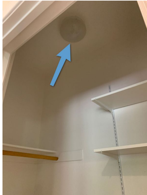
Example Noted at coat closet
