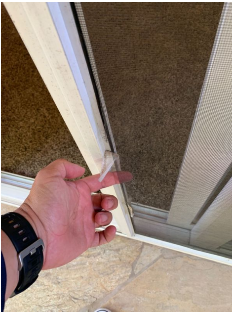
Example Noted at Patio
