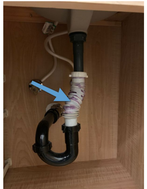
Example Noted at Master Bathroom
