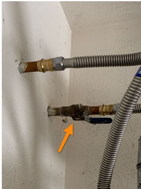
Example Noted at Water Heater
