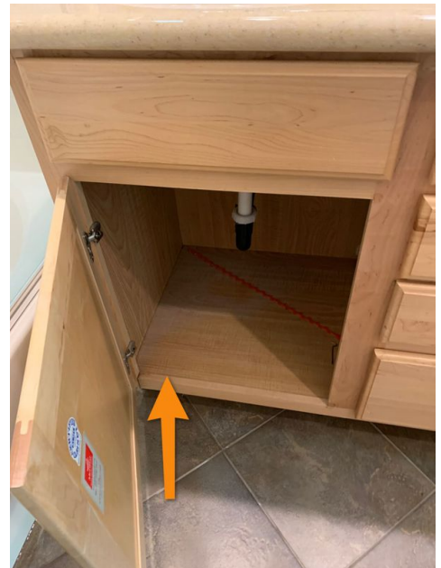
Example Noted at Master Bathroom
