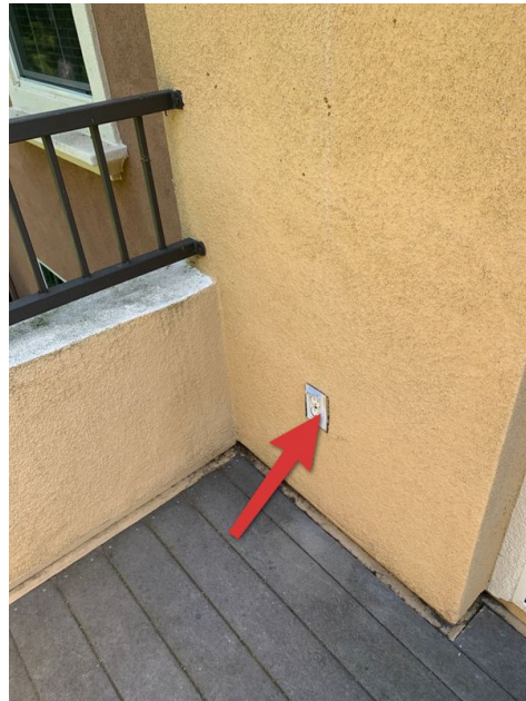
Example Noted at Balcony
