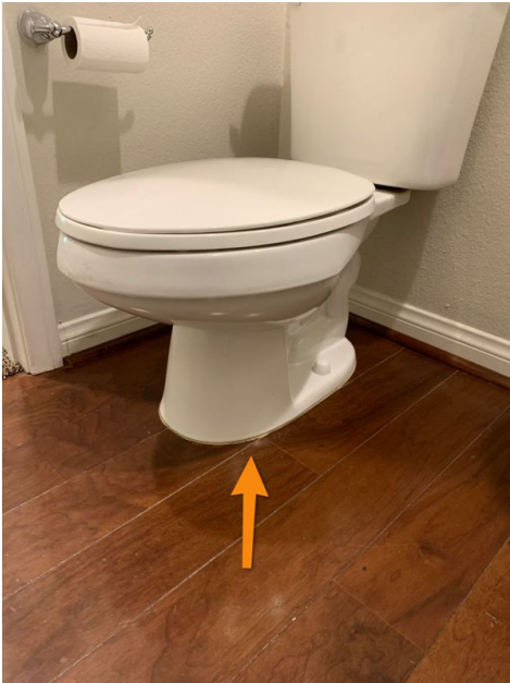
Example Noted at Half Bathroom
