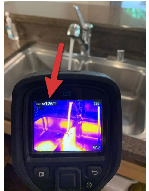
Example Noted at Kitchen
