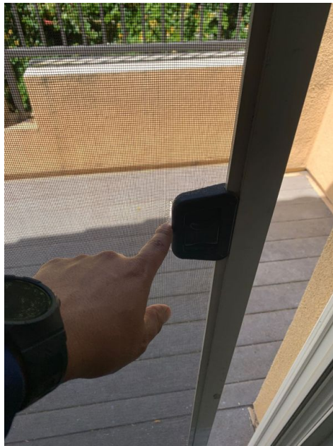
Example Noted at Master Bedroom
