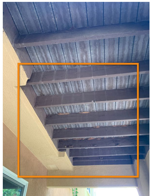
Example Noted at Balcony
