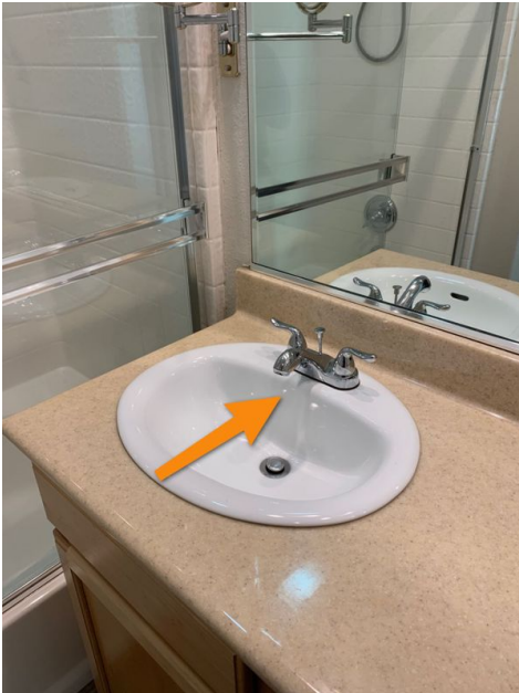
Example Noted at Master Bathroom
