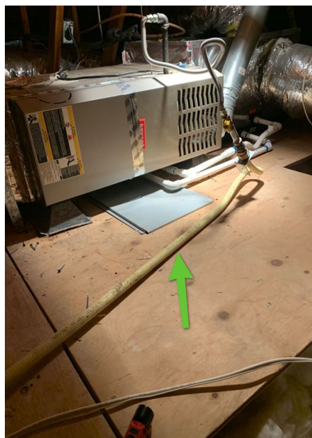
Example Noted at Attic
