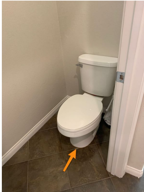
Example Noted at Master Bathroom
