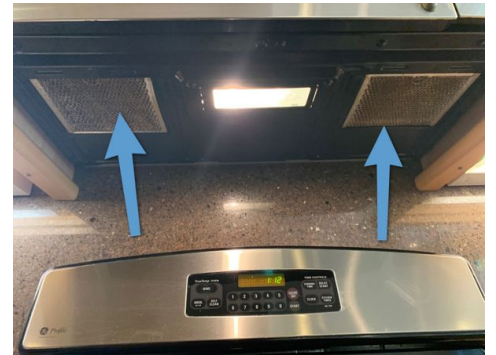
Example Noted at Kitchen
