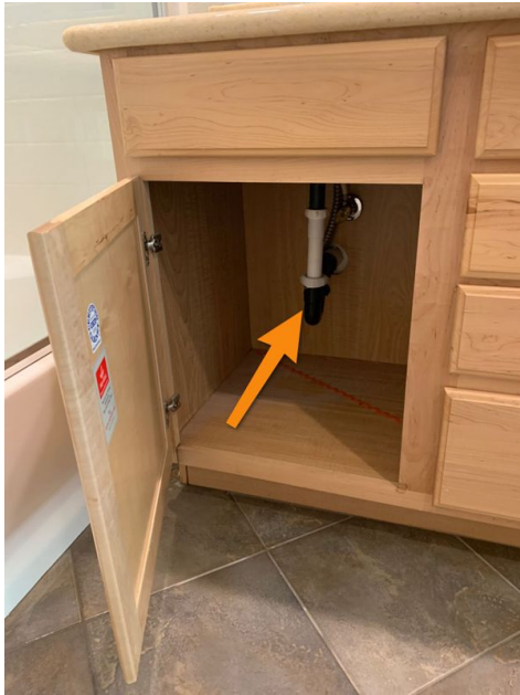
Example Noted at Master Bathroom
