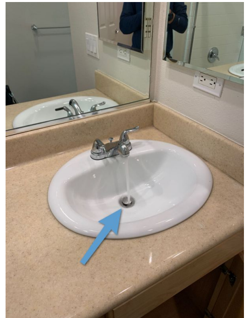
Example Noted at Master Bathroom
