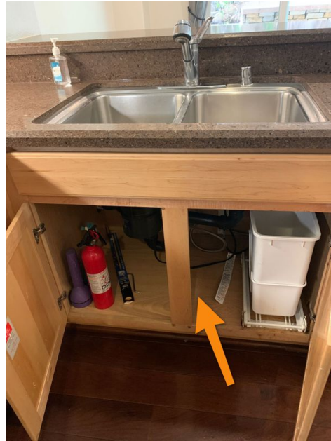
Example Noted at Kitchen
