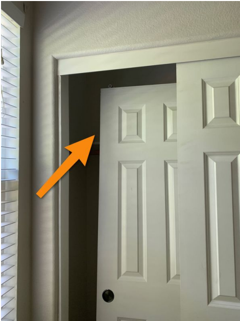
Example Noted at Bedroom #2
