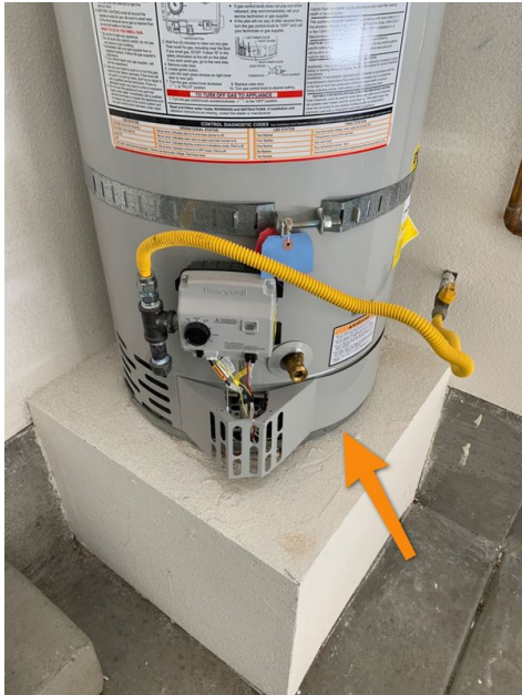
Example Noted at Water Heater
