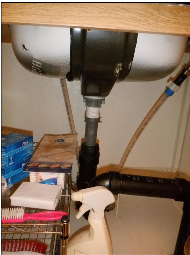
5.6 Item 5(Picture) Hallway bath sink plumbing
