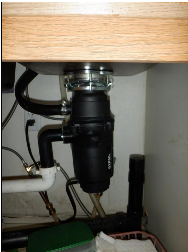
3.11 Item 1(Picture) Garbage disposal
