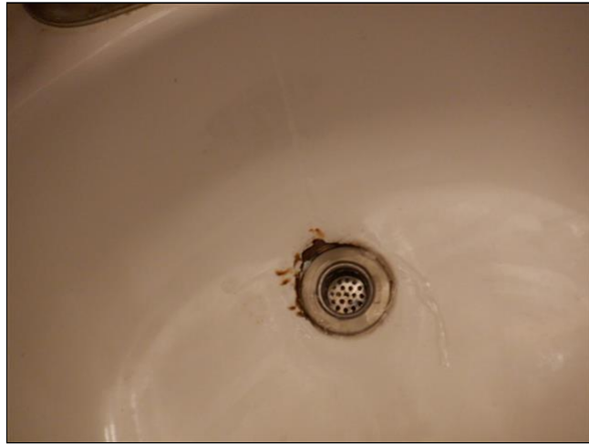
5.6 Item 4(Picture) Damaged hallway bath sink drain
