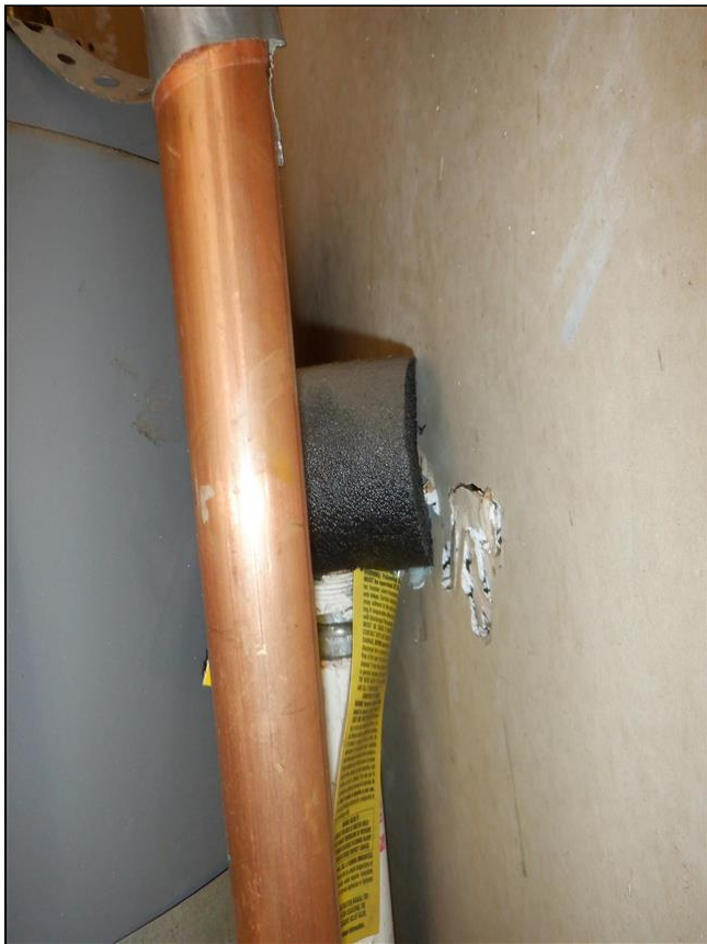
7.1 Item 5(Picture) T&P plumbing
