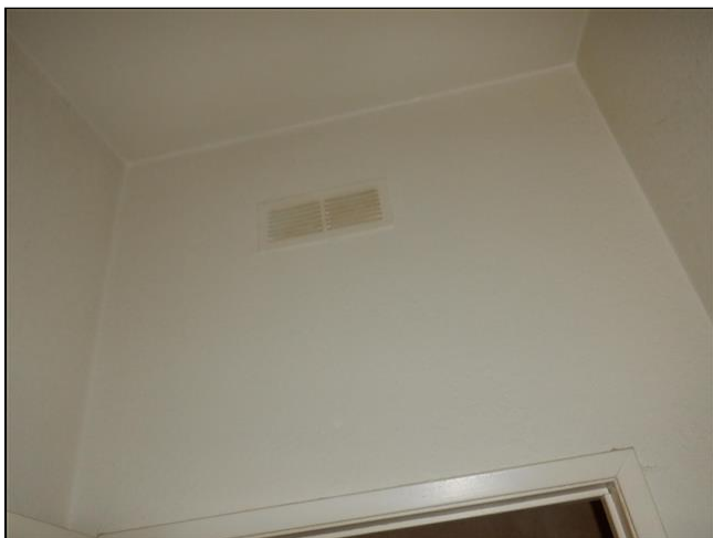
8.5 Item 1(Picture) Missing bedroom smoke detectors
