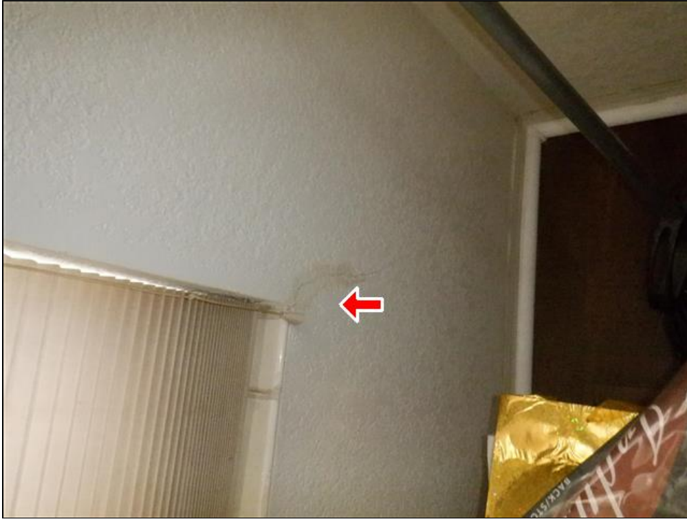
4.1 Item 1(Picture) Settling cracks
