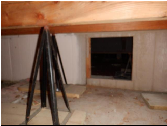
6.2 Item 3(Picture) Steel jacks
