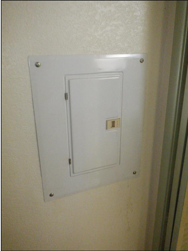
8.0 Item 1(Picture) Electrical panel
