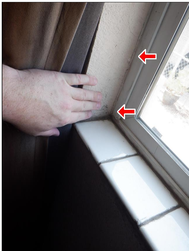
4.4 Item 1(Picture) Windows not sealed
