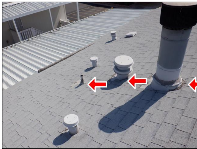
1.1 Item 2(Picture) Worn sealant
