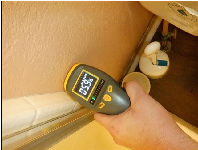
5.1 Item 3(Picture) Moisture test around hallway bath plumbing
