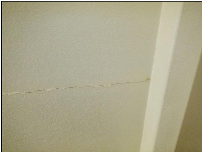
4.0 Item 1(Picture) Settling crack in living room ceiling
