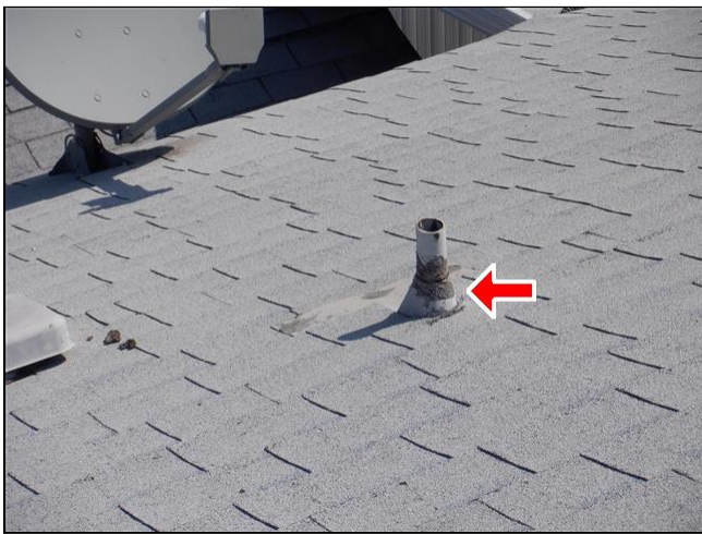
1.1 Item 1(Picture) Worn sealant
