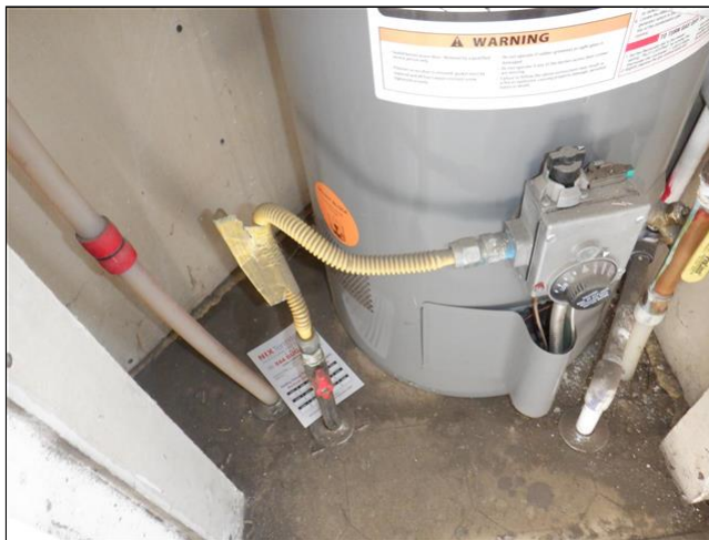
7.1 Item 8(Picture) Missing sediment trap
