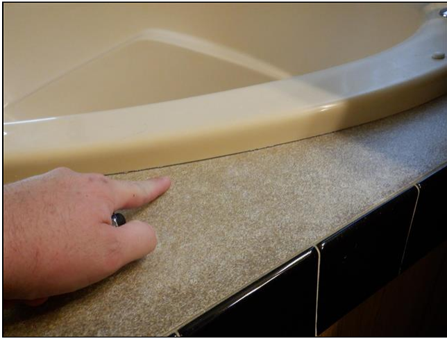
5.7 Item 5(Picture) Tub not sealed
