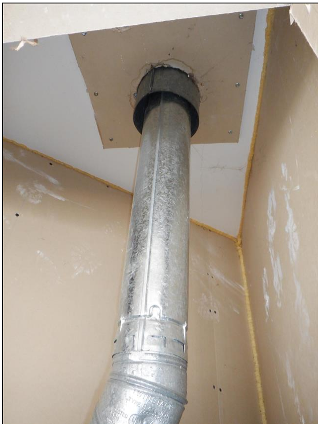
7.1 Item 7(Picture) Flue venting
