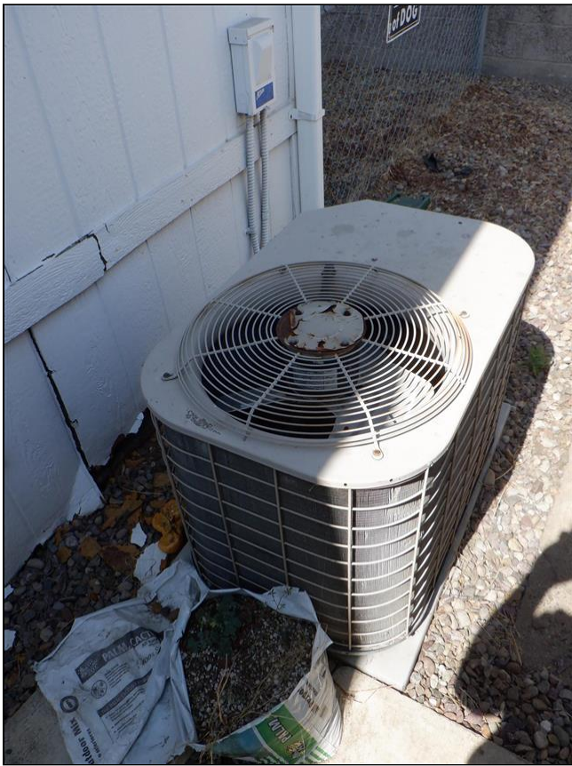
9.6 Item 1(Picture) Condenser
