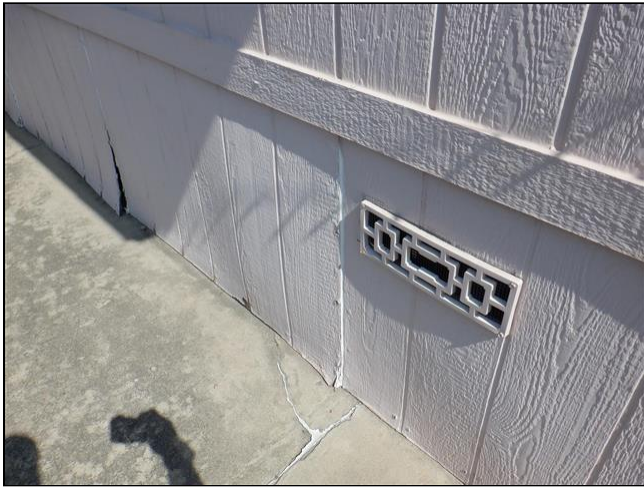
6.0 Item 3(Picture) Damaged skirting
