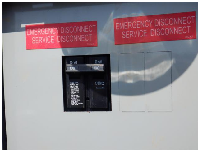
8.4 Item 2(Picture) Main 100 amp breaker
