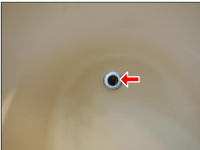
5.6 Item 1(Picture) Missing primary tub stopper
