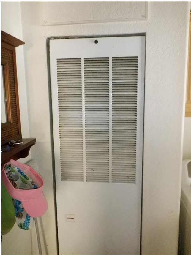
9.0 Item 1(Picture) Furnace
