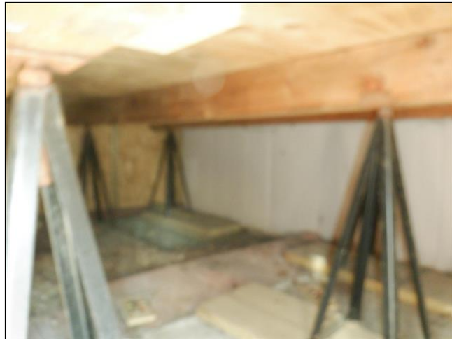
6.2 Item 2(Picture) Steel jacks
