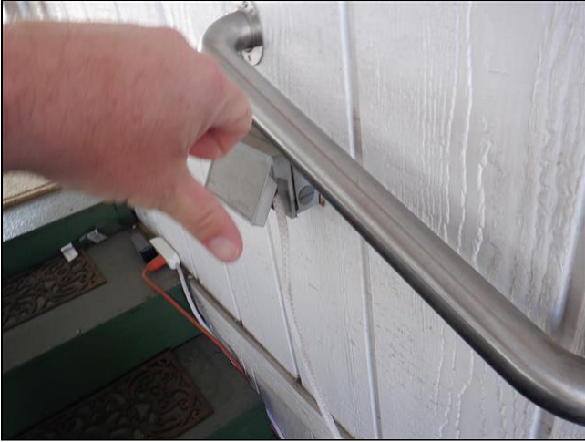
2.7 Item 1(Picture) Not GFCI
