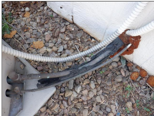
9.6 Item 2(Picture) Missing insulation
