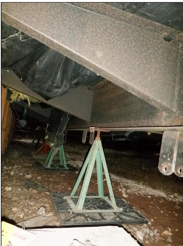
6.2 Item 5(Picture) Steel jacks
