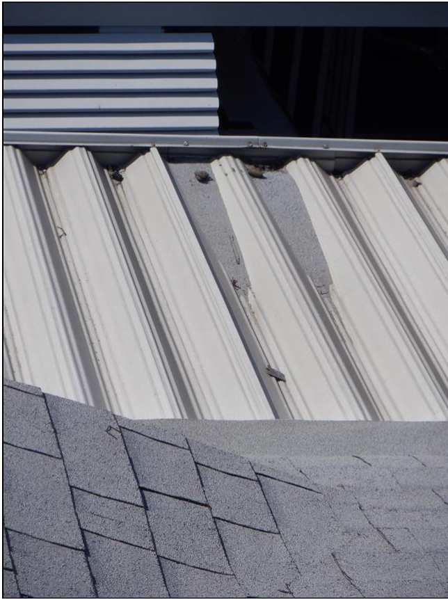
1.0 Item 13(Picture) Debris in carport cover
