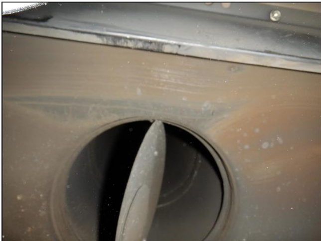
9.5 Item 3(Picture) Flue damper
