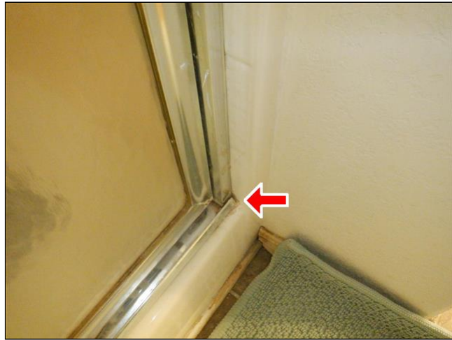
5.7 Item 2(Picture) Worn caulking on shower door
