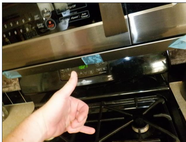
3.12 Item 2(Picture) Microwave too close to cook top
