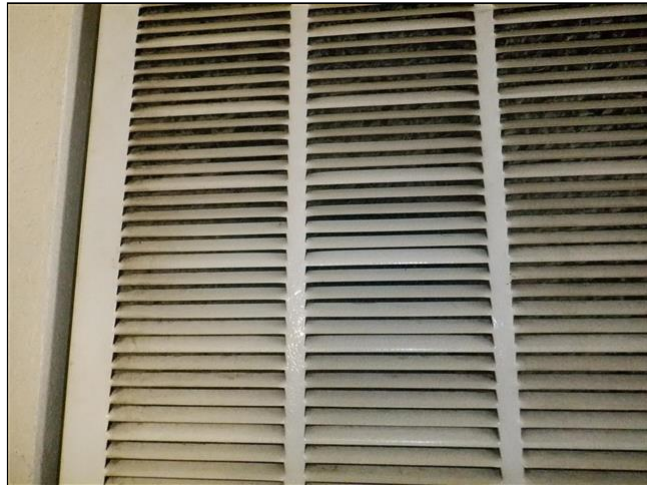
9.0 Item 2(Picture) Dirty filter
