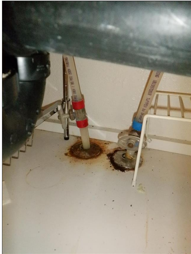
5.7 Item 6(Picture) Corrosion
