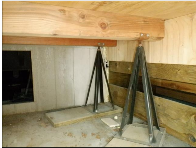
6.2 Item 4(Picture) Steel jacks
