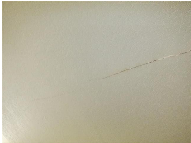
4.0 Item 2(Picture) Settling crack in living room ceiling
