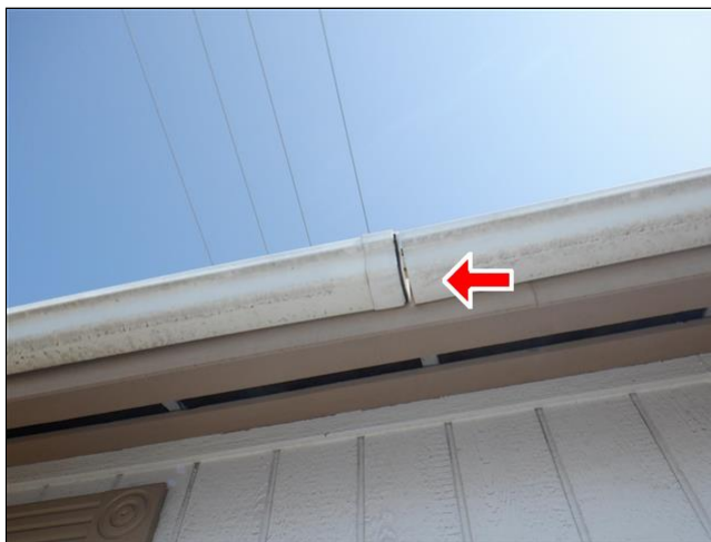
1.3 Item 2(Picture) Separated gutters
