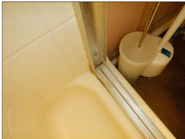
5.7 Item 8(Picture) Worn caulking at hallway bath shower door
