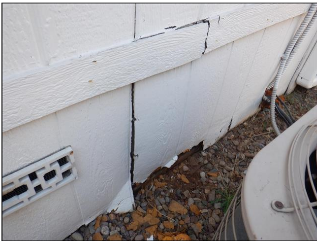
6.0 Item 1(Picture) Damaged skirting
