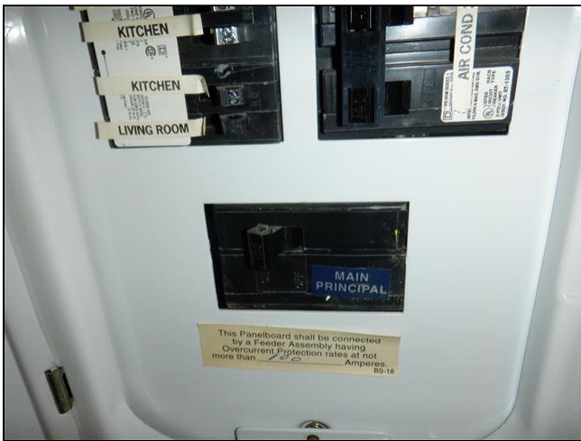
8.0 Item 3(Picture) Circuit breakers
