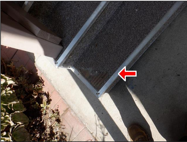
2.3 Item 1(Picture) Loose step
