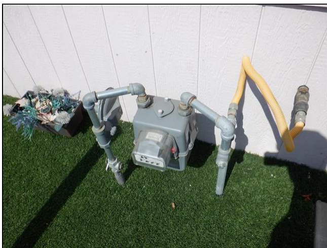
7.4 Item 1(Picture) Gas meter and shut off
