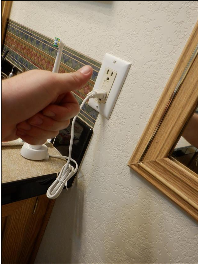
5.8 Item 1(Picture) Good GFCI (master for both bathrooms)
