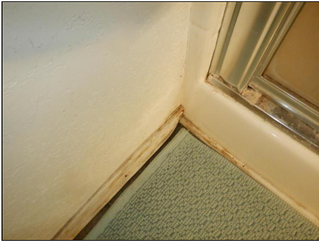
5.7 Item 1(Picture) Damaged trim by shower
