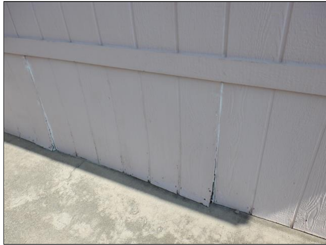
6.0 Item 4(Picture) Damaged skirting
