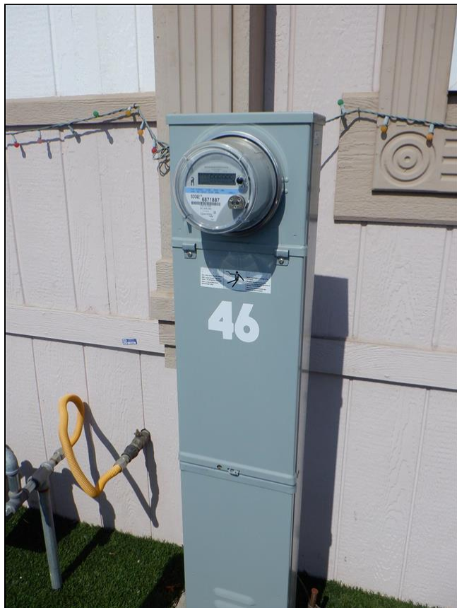
8.4 Item 1(Picture) Electric meter
