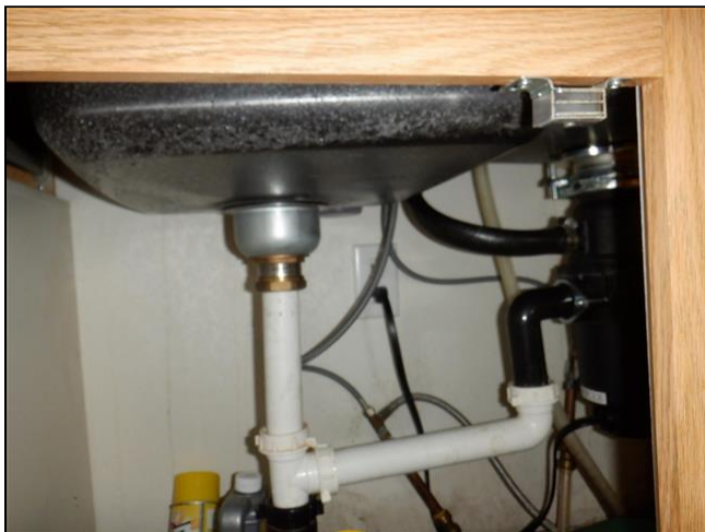
3.5 Item 1(Picture) Kitchen sink plumbing
