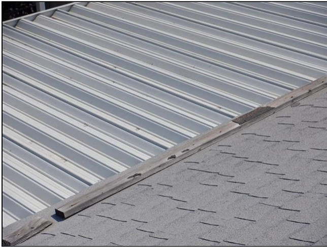
1.0 Item 7(Picture) Roof covering / improper flashing
