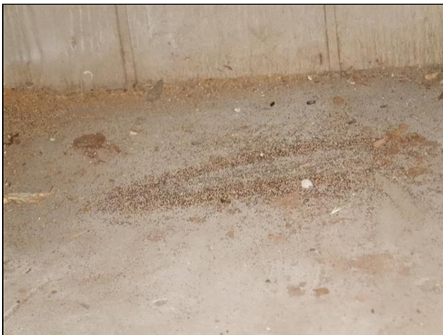
6.0 Item 5(Picture) Termite droppings under deck
