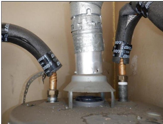
7.1 Item 6(Picture) Flue venting and water lines
