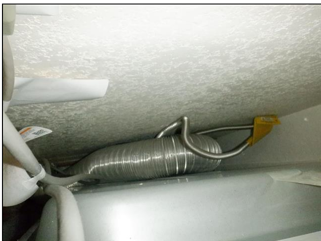
3.13 Item 3(Picture) Gas connection for dryer
