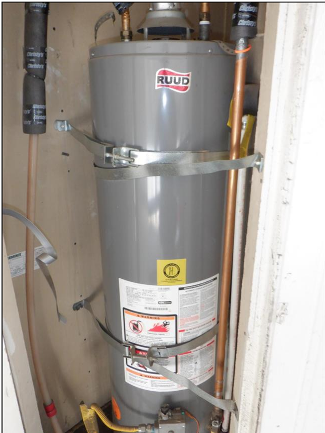
7.1 Item 1(Picture) Water heater
