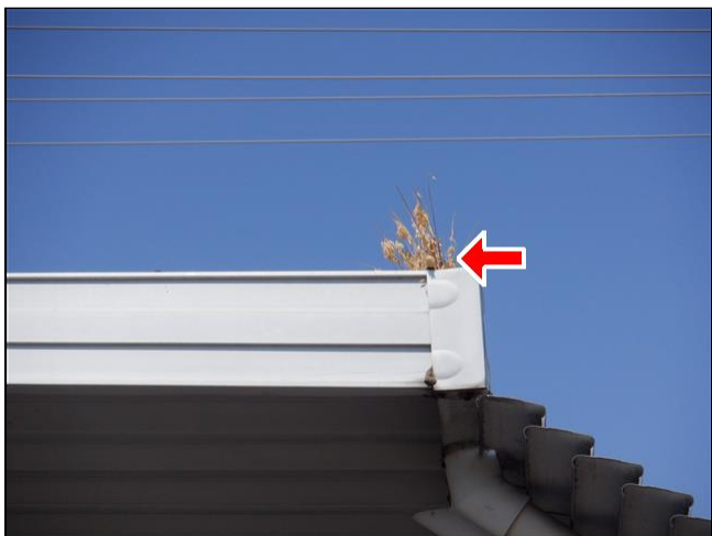
1.3 Item 1(Picture) Debris in gutters
