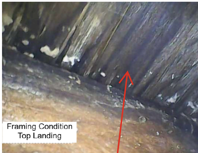
Evidence of Moisture
