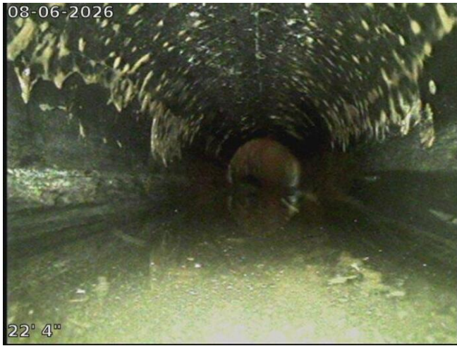
2026-08-06-13-49-19 Damaged ABS to Cast Iron connection
