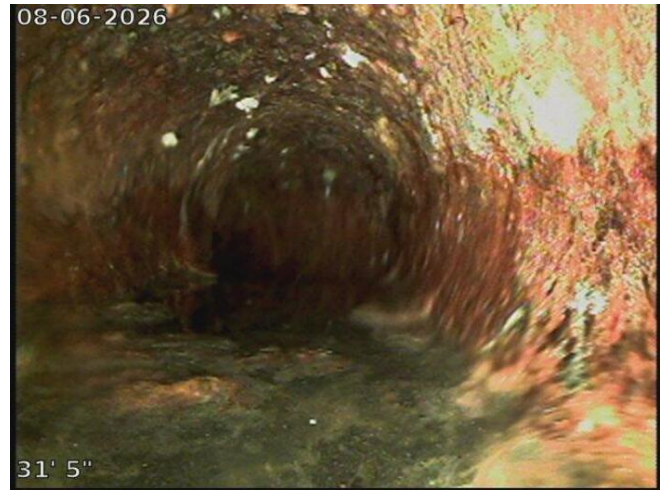
2026-08-06-13-46-34 Heavy buildup in the Cast Iron
