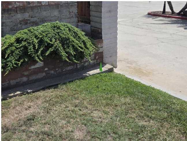
No title Flag marking an area of the damaged ABS (about 4' deep)
