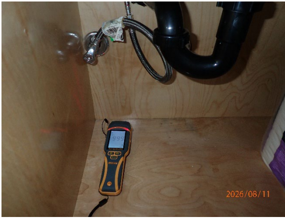
Elevated moisture readings on base shelf of cabinet below guest bathroom sink
