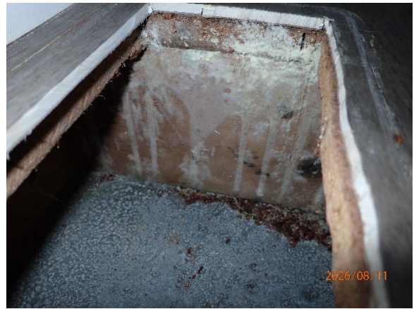
Mold growth on subfloor and floor joist
