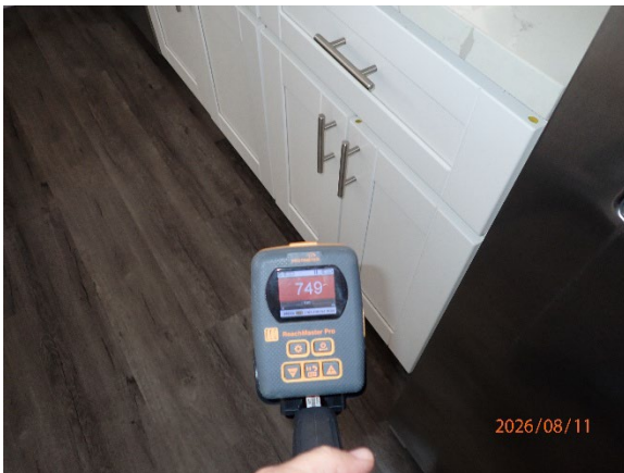
Elevated moisture readings on floor in kitchen
