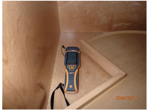
Elevated moisture readings on base shelf of corner cabinet in kitchen
