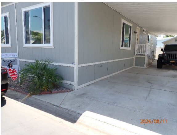
No perimeter vents at east or north side of home below living room, laundry, guest bathroom, and guest bedroom
