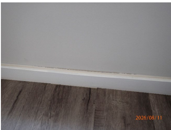
Baseboard separating from east wall of living room
