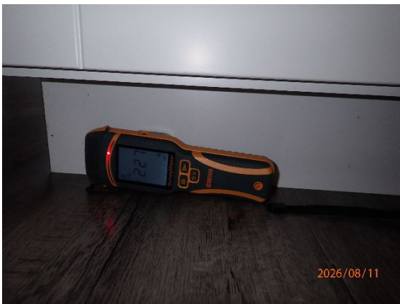
Elevated moisture readings on toe kick of peninsula in kitchen
