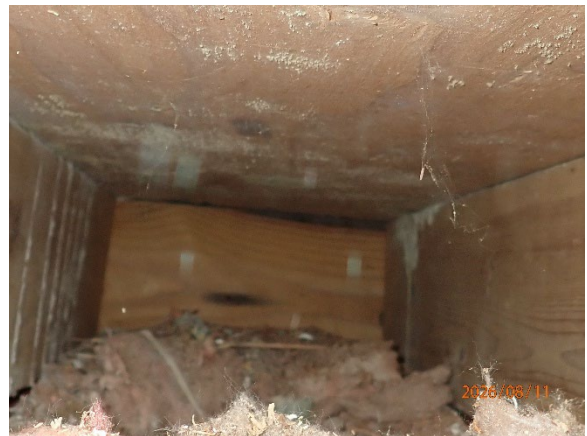
Mold growth on underside of subfloor
