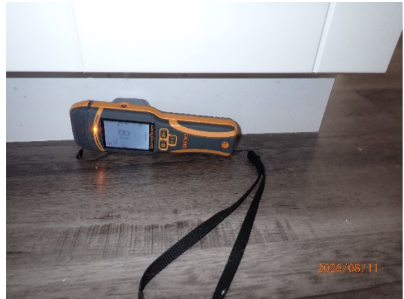
Elevated moisture readings on toe kick of kitchen island
