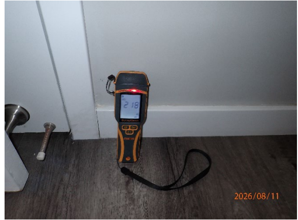
Elevated moisture readings on west wall of guest bathroom next to bedroom door
