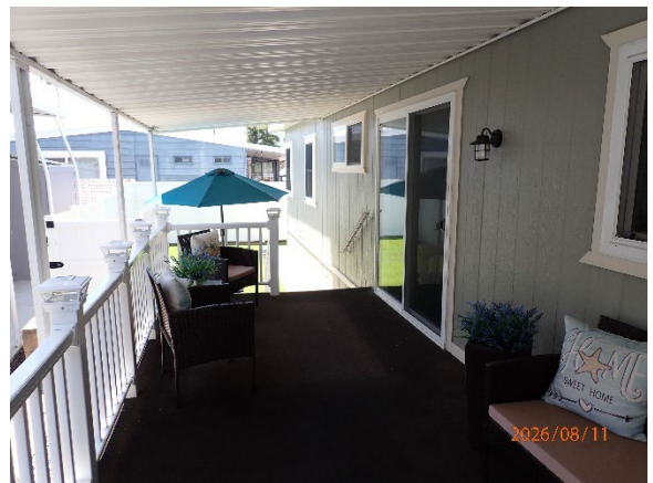
No perimeter vents at south side of home outside of living room, kitchen, and family room
