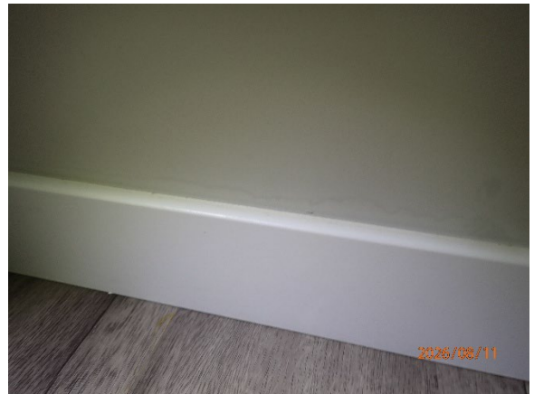
Stain at base of west wall in family room
