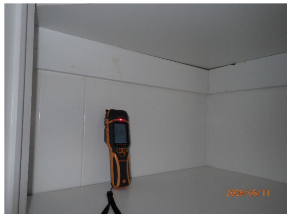
Elevated moisture readings in linen closet adjacent to guest bathroom
