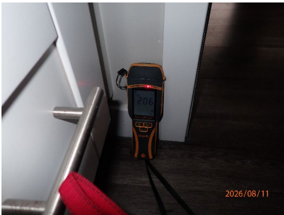
Elevated moisture readings on south wall right of vanity cabinet in guest bathroom
