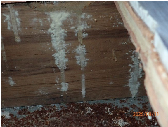
Mold growth on floor joist
