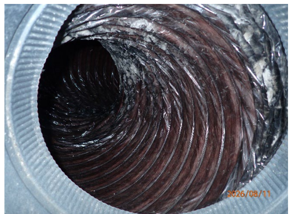
Mold growth in return duct
