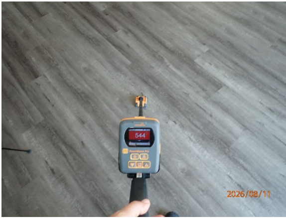
Elevated moisture readings on floor in living room
