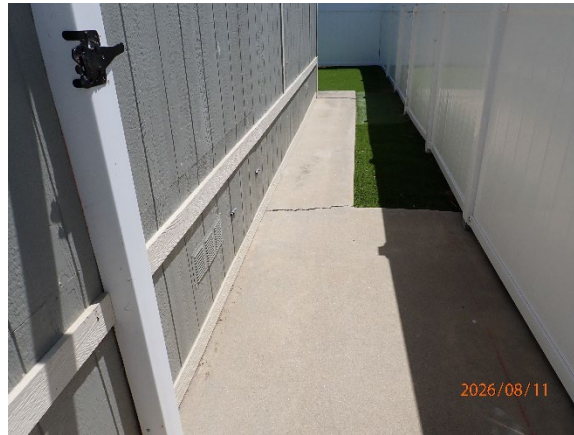
Perimeter vents at west side of home below primary bedroom
