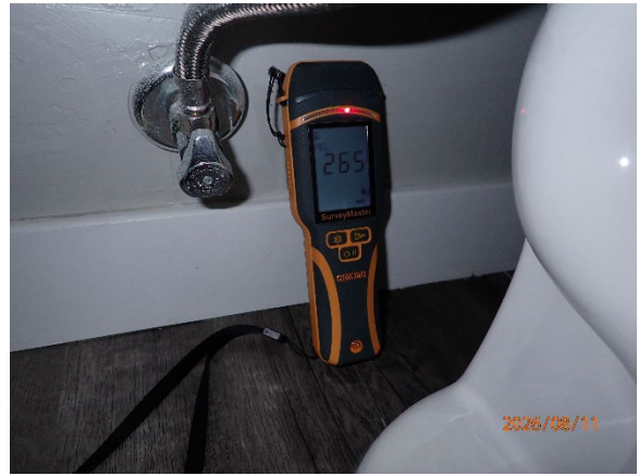
Elevated moisture readings on east wall behind toilet in guest bathroom
