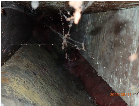
Mold growth below flooring at east side of living room
