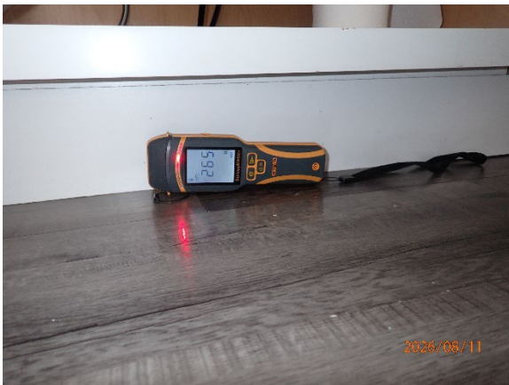
Elevated moisture readings on toe kick below kitchen sink
