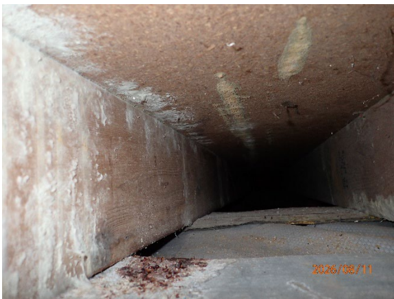
Mold growth on underside of subfloor and floor joist
