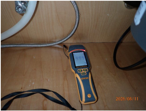
Elevated moisture readings on base shelf below kitchen sink
