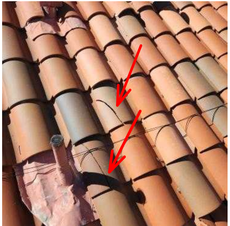
(6-8) broken roof tiles in areas
