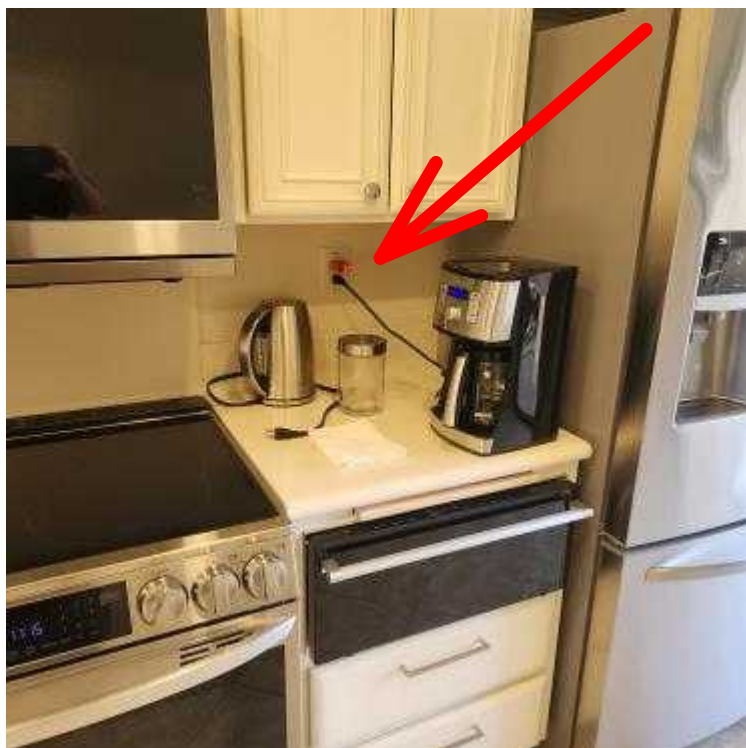
North outlet on west wall in kitchen not GFCI protected-NTBS
