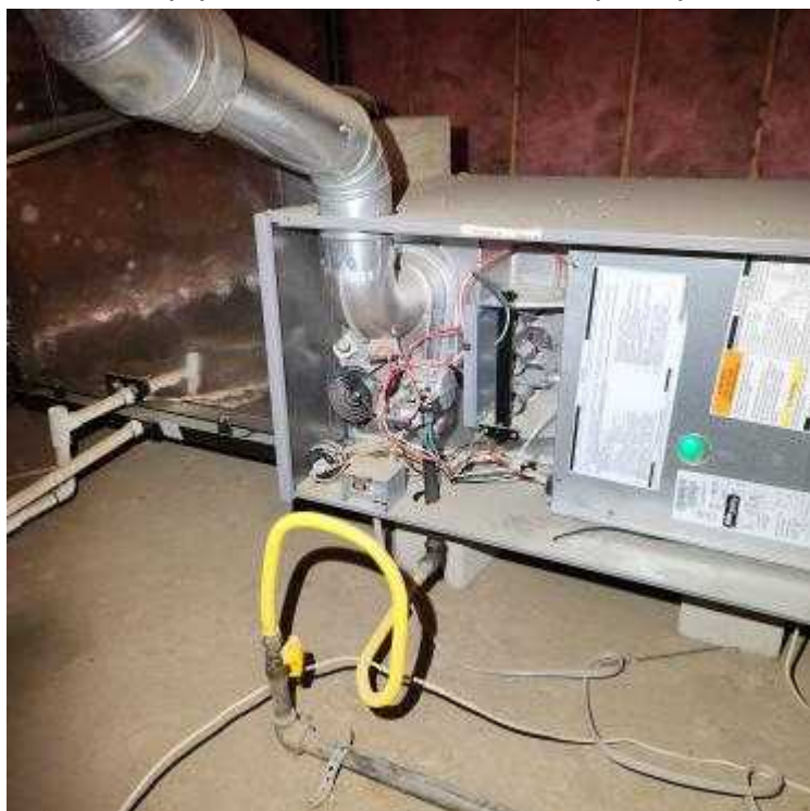
Heater operated properly (70k BTU 2011 model located in attic)
