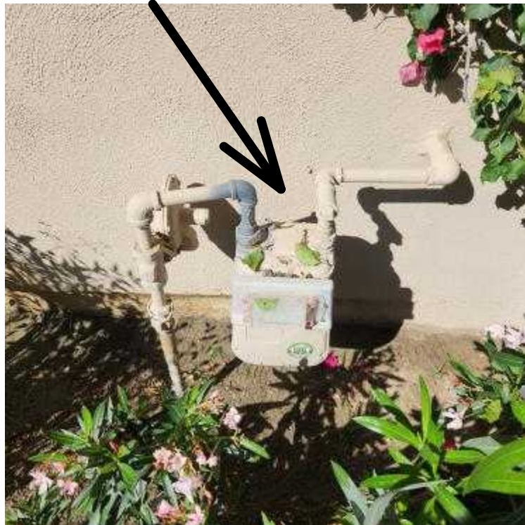
Gas Meter to proprty GV (Located on east side of garage)
