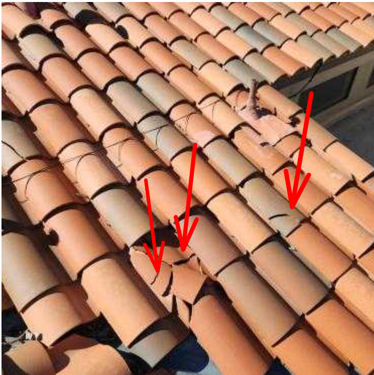
(6-8) broken roof tiles in areas
