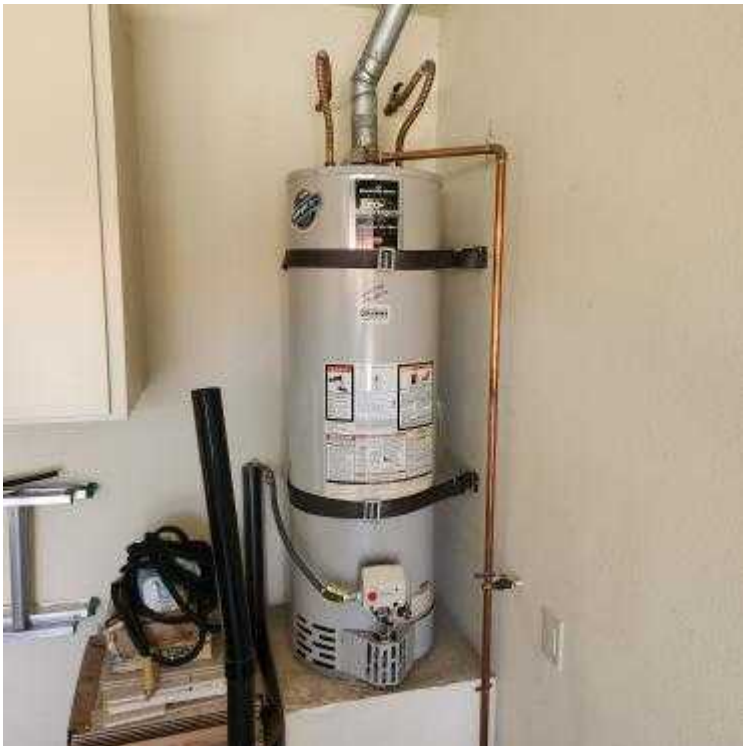
Water Heater operated & strapped properly (40 gallon 2011 model located in garage)
