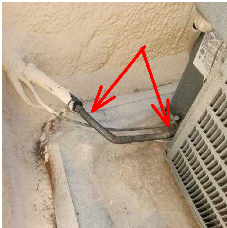
Torn insulation/Exposed copper on refrigerant pipe to AC Condenser
