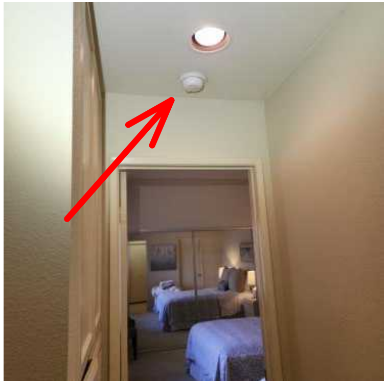
Missing carbon monoxide alarm in north hall outside bedroom-NTBS
