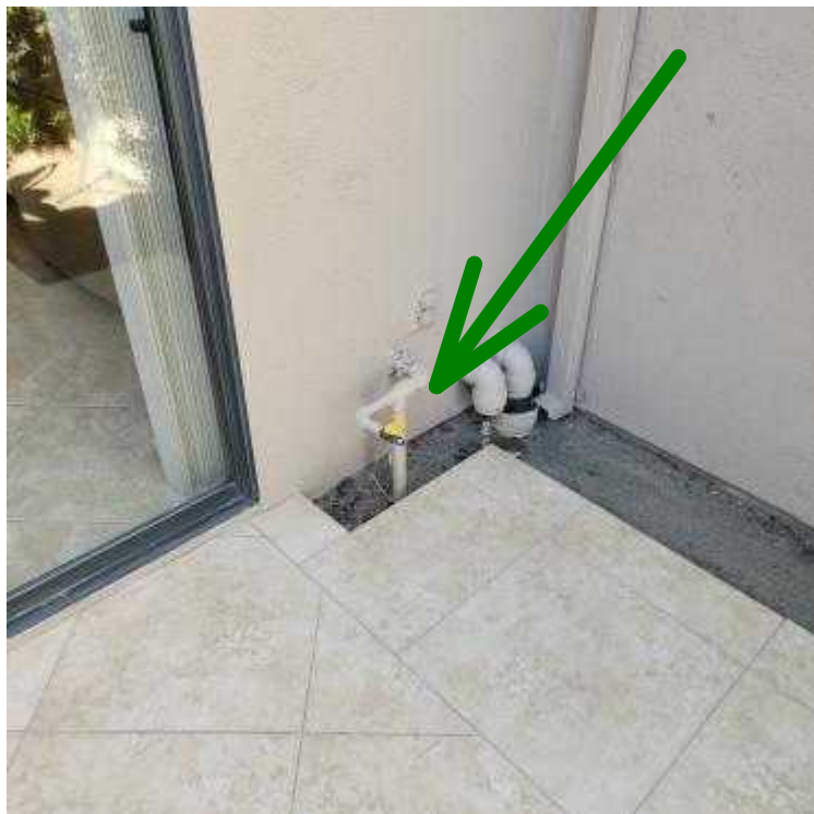
Gas valve on north wall of house operated at time of inspection
