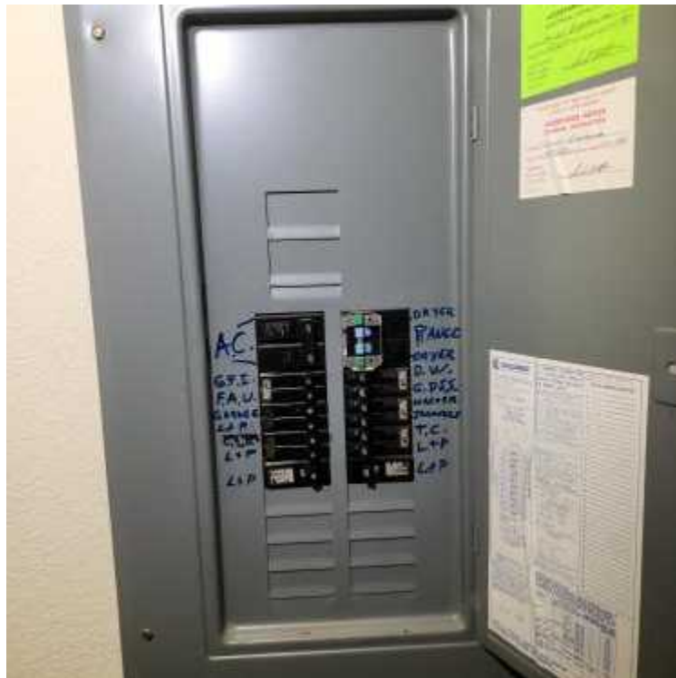
Main electrical panel GV (200 amp panel located in north bedroom closet)
