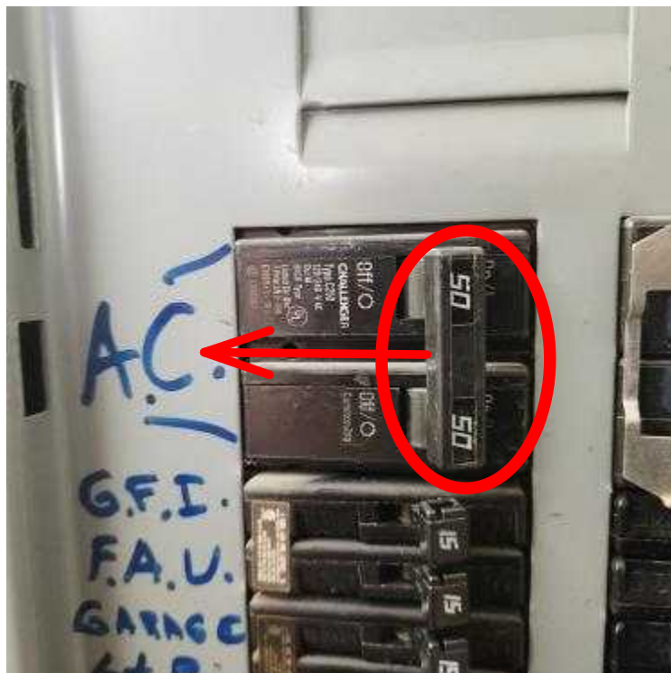
Breaker amperage to AC Condenser overcurrent exceeds unit requirement (40 amp max required-50 amp present in main electrical panel)
