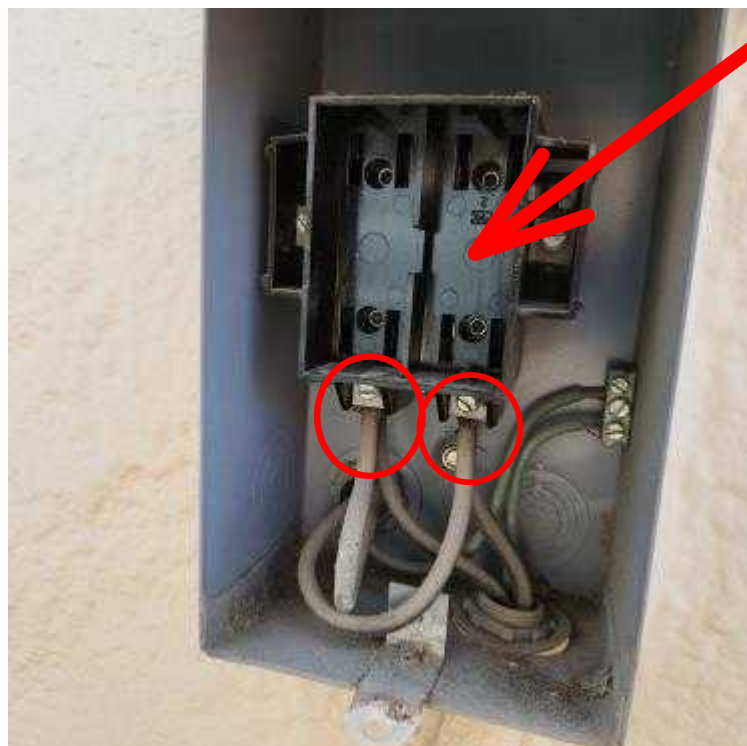
Missing fuses/carriage inside AC disconnect box & Unit wired hot-NTBS
