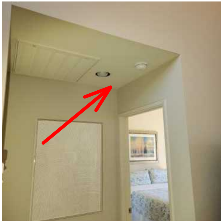
Missing carbon monoxide alarm in south hall outside bedroom-NTBS
