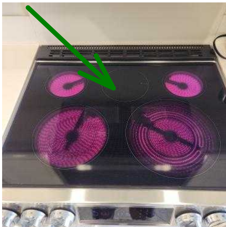
Electric range in kitchen operated at time of inspection (LG)
