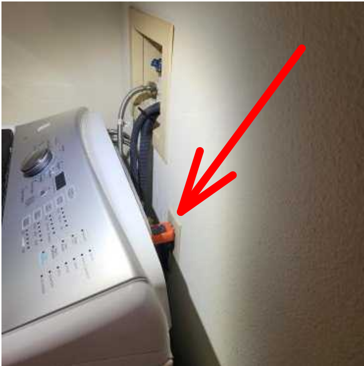
Outlet on wall in laundry closet not GFCI protected-NTBS-Required to be readily accessible to reset when replaced
