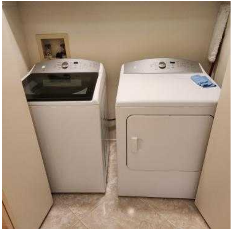
Washer & Dryer operated at time of inspection (Kenmore)
