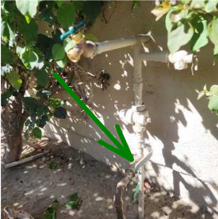
Water shut off to house operated (Located on east side of garage)
