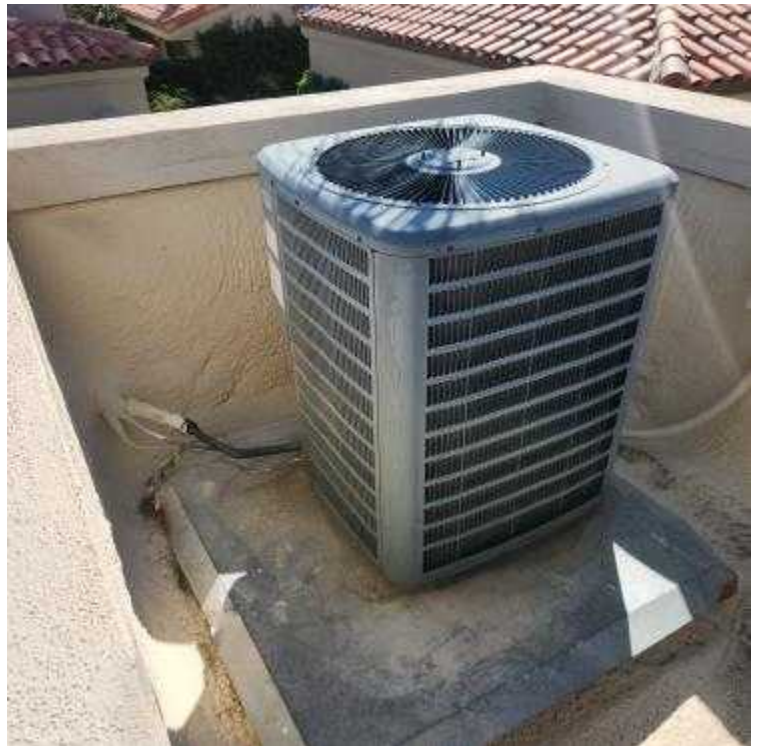
AC Condenser operated properly (4 ton 2011 model located on garage roof-East unit)
