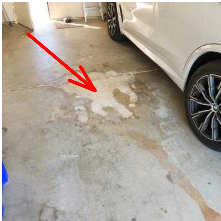
Acid stained concrete in garage
