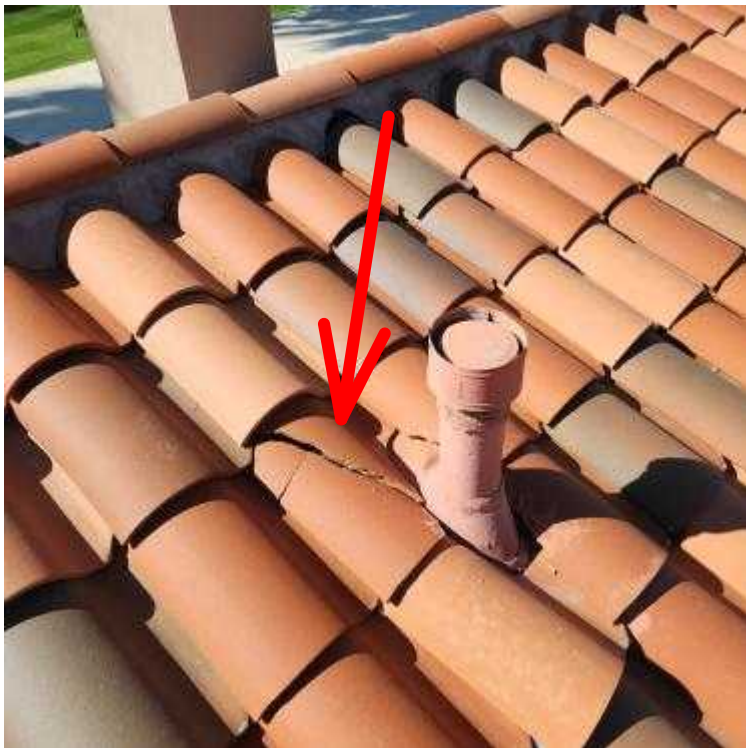
(6-8) broken roof tiles in areas
