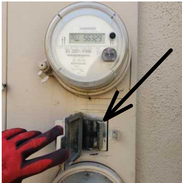
Main electrical disconnect breaker to house located on west side of 76647
