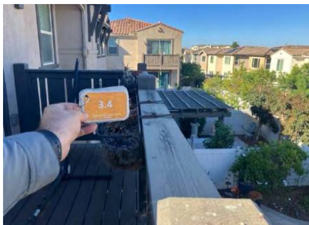
1218 Via Lucero, Balcony, North 3.4 Guardrail - Loose or Missing Hardware
