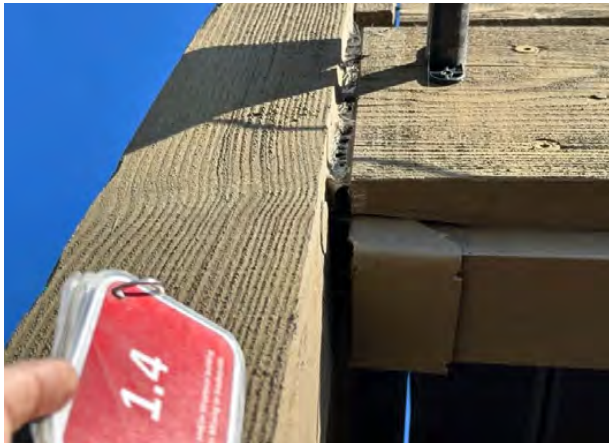
1127 Via Lucero, Balcony, West 1.4 Hardware and/or Structural Building Component Issues
