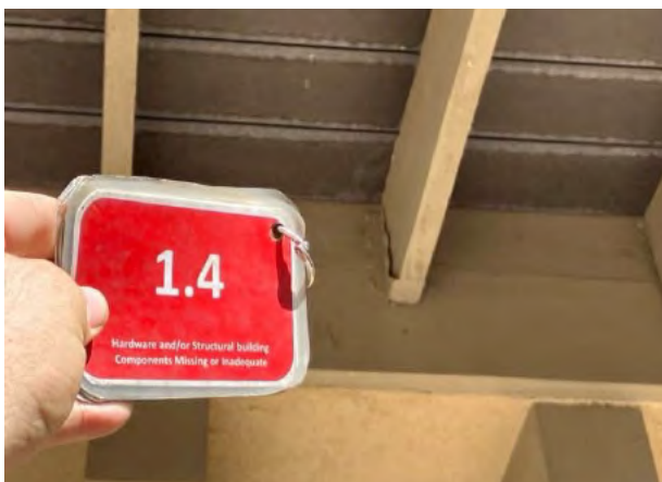
1195 Via Candelas, Balcony, South 1.4 Hardware and/or Structural Building Component Issues
