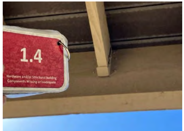
1191 Via Candelas, Balcony, South 1.4 Hardware and/or Structural Building Component Issues
