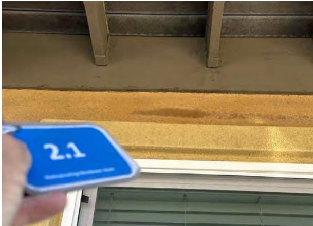
1151 Via Lucero, Balcony, West 2.1 Waterproofing Membrane Issues
