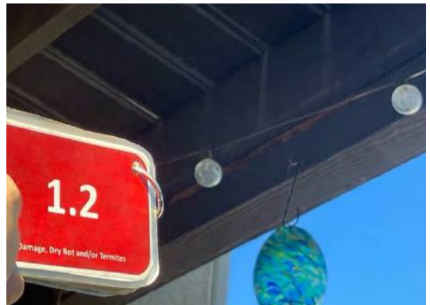
1208 Via Lucero, Balcony, East 1.2 Damage, Dry Rot and/or Termites
