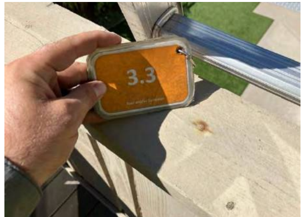
1191 Via Candelas, Balcony, South 3.3 Guardrail - Rust/Corrosion
