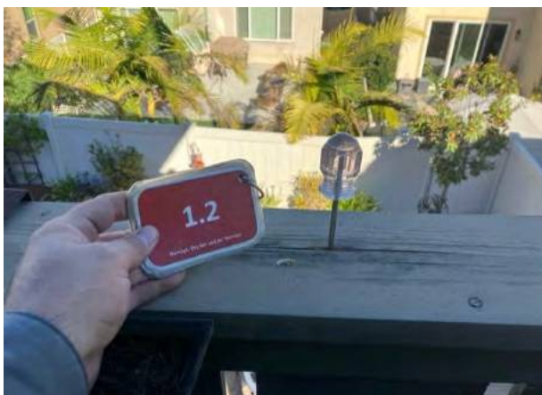
1218 Via Lucero, Balcony, North 1.2 Damage, Dry Rot and/or Termites
