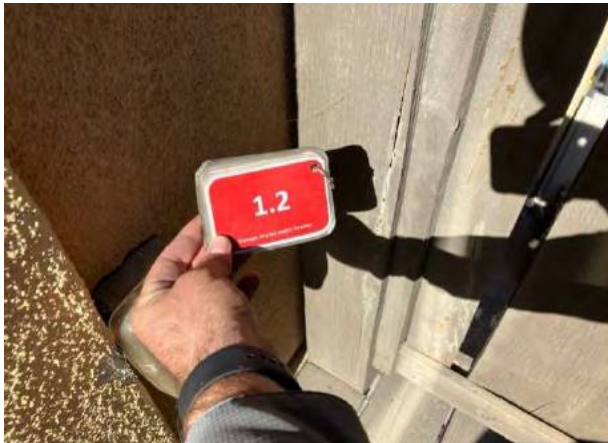
1278 Via Fanal, Balcony, East 1.2 Damage, Dry Rot and/or Termites
