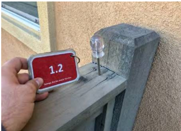
1202 Via Lucero, Balcony, West 1.2 Damage, Dry Rot and/or Termites
