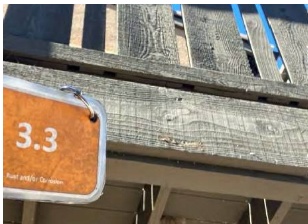
1278 Via Fanal, Balcony, East 3.3 Guardrail - Rust/Corrosion
