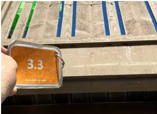
1136 Via Candelas, Balcony, East 3.3 Guardrail - Rust/Corrosion
