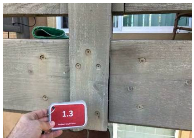
1202 Via Lucero, Balcony, West 1.3 Hardware Rust/Corrosion
