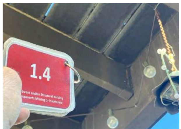
1208 Via Lucero, Balcony, East 1.4 Hardware and/or Structural Building Component Issues
