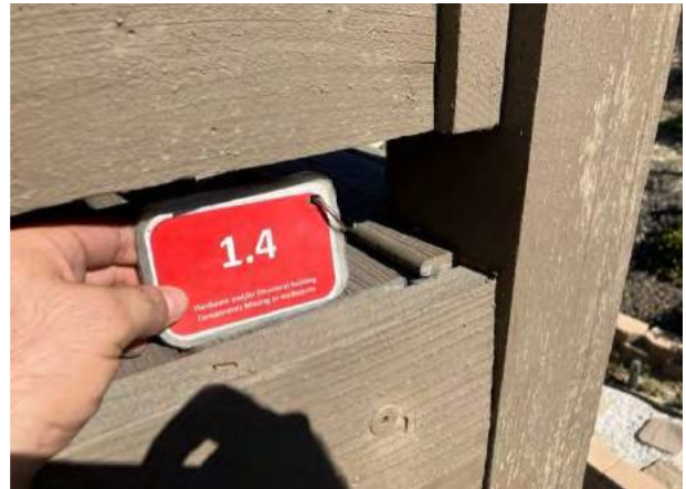
1132 Via Cuesta, Balcony, East 1.4 Hardware and/or Structural Building Component Issues
