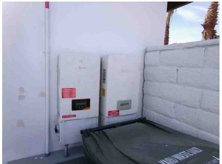
SOLAR PANEL SYSTEMS
