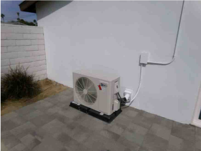
OTHER HEATING/COOLING UNIT
