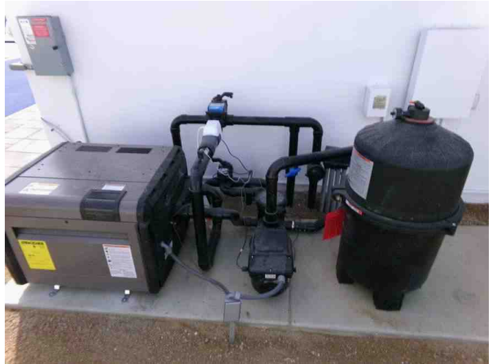
NEW POOL/SPA EQUIPMENT
