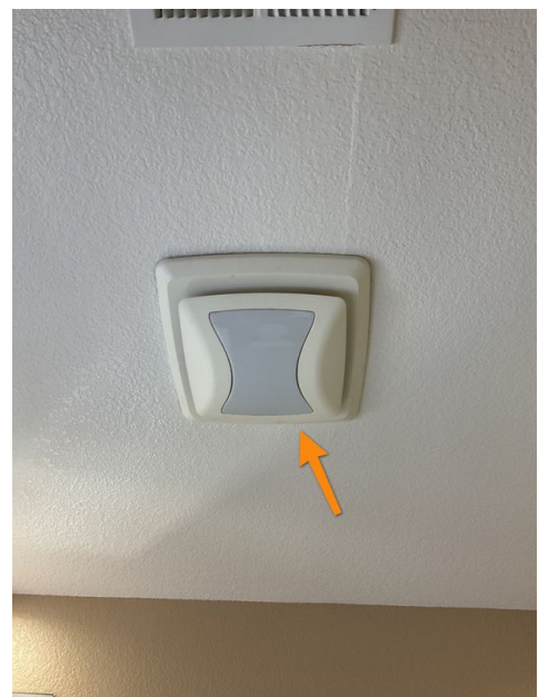
Light Bulb Need Replacement
