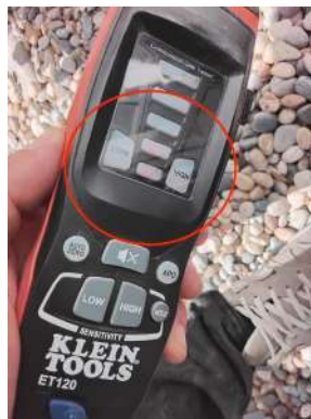
Gas Leak Detected
