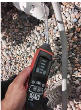
Gas Leak Detected
