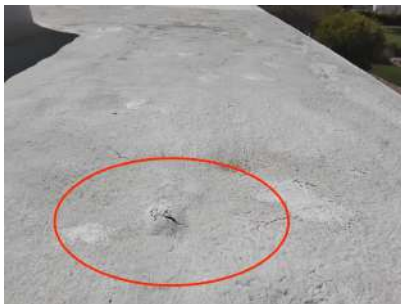
Blistering + Holes In Foam
