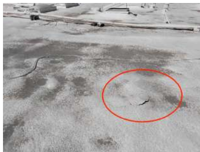
Blistering + Holes In Foam
