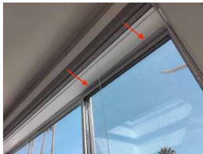
Evidence Of Leakage - Dining Room
