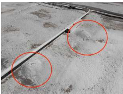
Blistering + Holes In Foam
