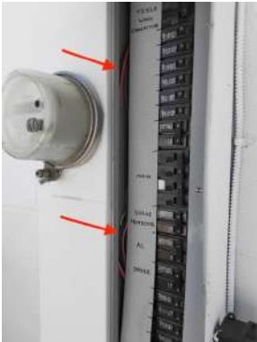
Inadequate Dead Front Cover
