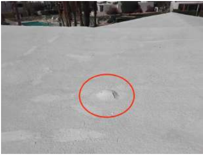
Blistering + Holes In Foam
