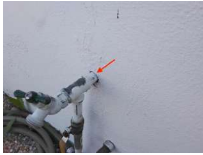
Unsealed Wall Penetration - North
