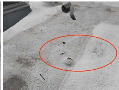
Blistering + Holes In Foam
