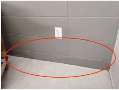
Water Damage - Living Room (East Wall)
