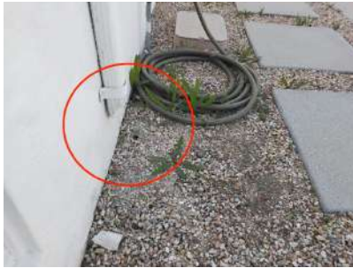
Inadequate Downspout Termination - North
