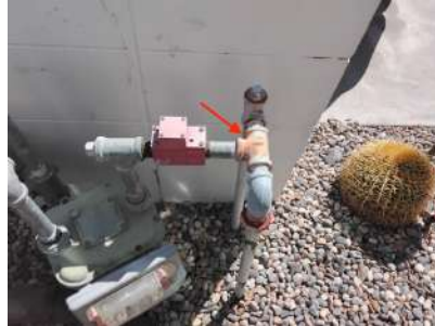
Rust On Pipes and Fittings
