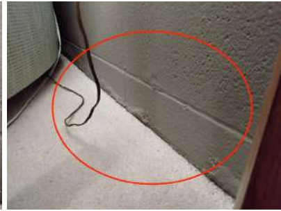
Water Damage - Living Room (East Wall)
