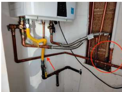
Inadequate TPR Valve Extension
