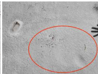
Elastomeric Deterioration + Exposed Foam
