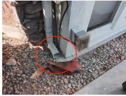
Inadequate Downspout Termination - South
