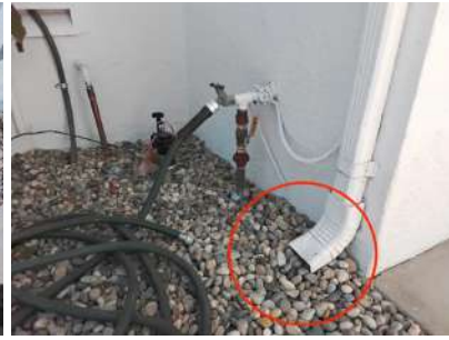
Inadequate Downspout Termination - South
