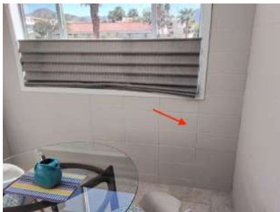
Evidence Of Leakage - Dining Room
