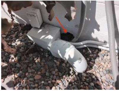
Unsealed Hole - South
