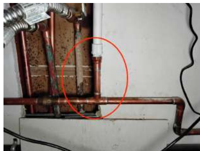
Inadequate TPR Valve Extension
