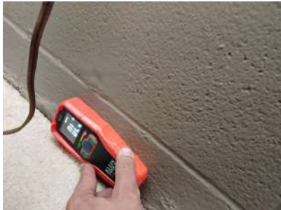
High Moisture Levels - Living Room (East Wall)
