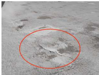
Blistering + Holes In Foam
