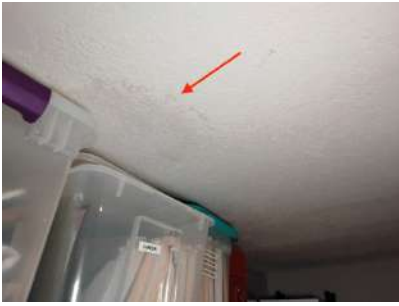
Water Stains - Guest Bedroom Closet
