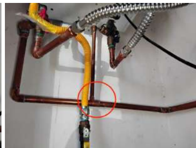
Inadequate TPR Valve Extension
