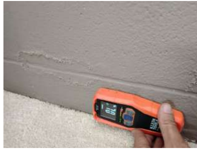
High Moisture Levels - Living Room (East Wall)
