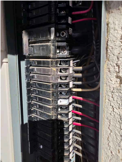
Panel: Main Amp Breaker Rating 100
