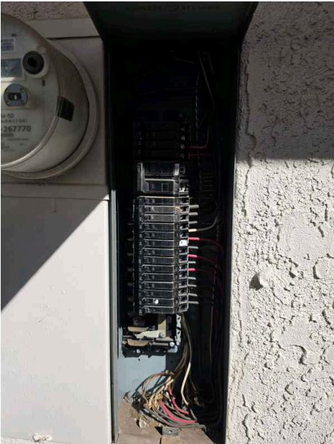
Panel: Panel Brand General Electric
