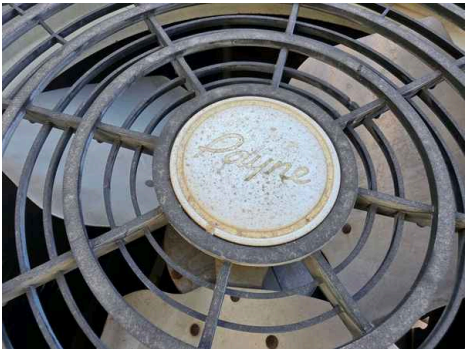
AC Compress Condition: AC Date of Manufacture
