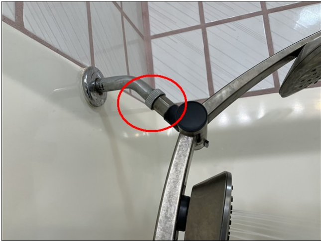
6.5 Item 3(Picture) shower valve leaked during testing
