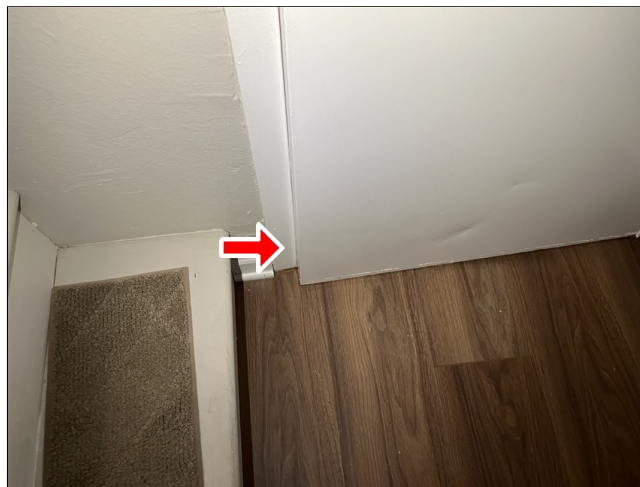
4.3 Item 2(Picture) garage door rubs against the jamb
