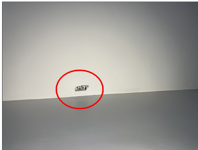
7.5 Item 5(Picture) bedroom ceiling: missing box cover
