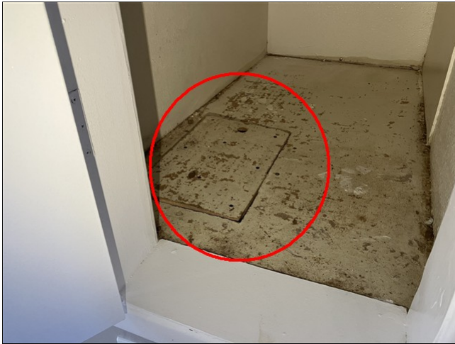
4.4 Item 1(Picture) possible evidence of repair or modification observed / recommend further evaluation
