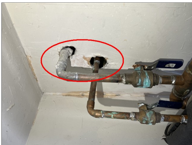
3.1 Item 3(Picture) unsealed penetrations observed in garage firewalls
