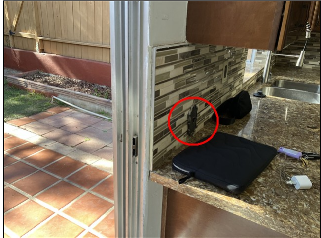
7.5 Item 2(Picture) switch and corresponding fixture or outlet were not identified
