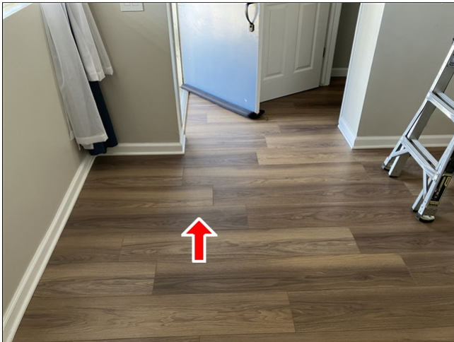
4.8 Item 1(Picture) possible slope or hump observed / recommend further evaluation
