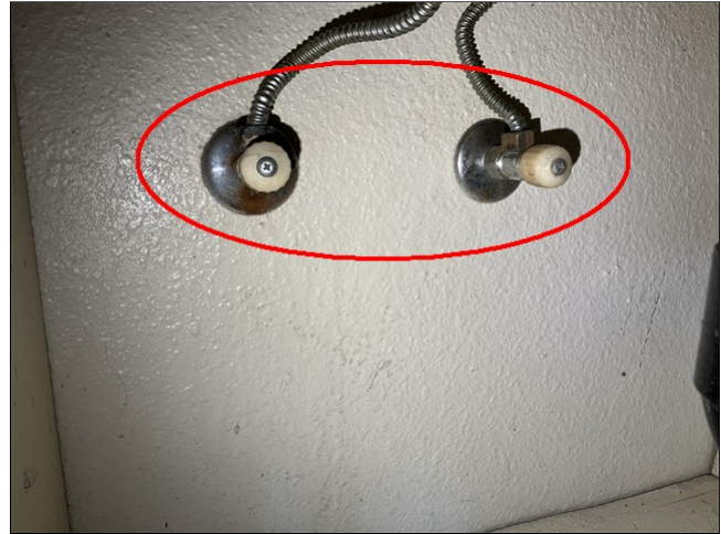
6.4 Item 2(Picture) bathrooms: aged water supply valves/hoses observed
