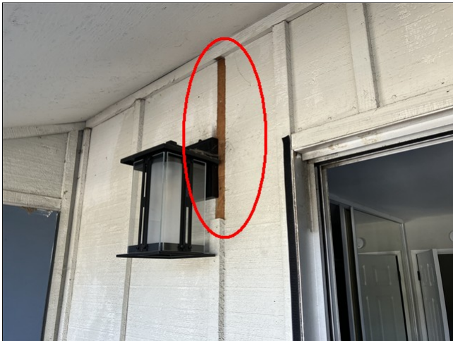
2.6 Item 9(Picture) siding trim maintenance/repairs needed
