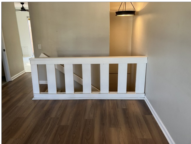
4.2 Item 3(Picture) railing safety upgrades recommended
