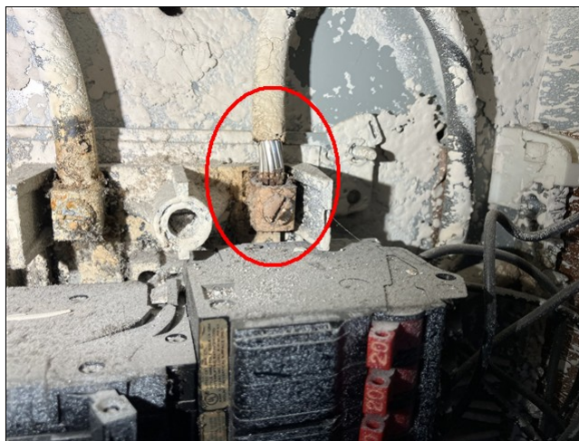
7.3 Item 2(Picture) panel wiring: a performance and safety inspection by a qualified person is recommended
