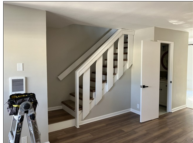
4.2 Item 2(Picture) railing safety upgrades recommended
