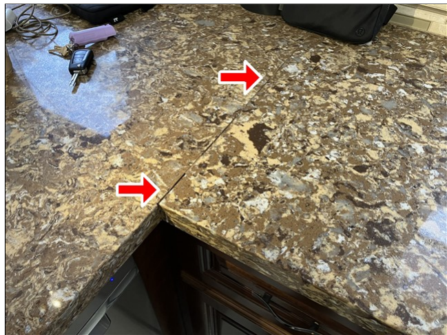
4.4 Item 4(Picture) kitchen countertop: epoxy sealant maintenance/repairs needed
