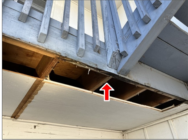
2.6 Item 8(Picture) decks/stairs: possible WDO evidence or damage observed / recommend further evaluation and correction as needed
