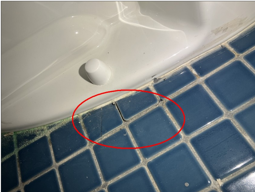
4.1 Item 2(Picture) bathroom: tile defects observed around toilet / recommend further evaluation and correction as needed
