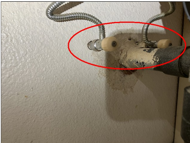
6.4 Item 5(Picture) bathrooms: aged water supply valves/hoses observed
