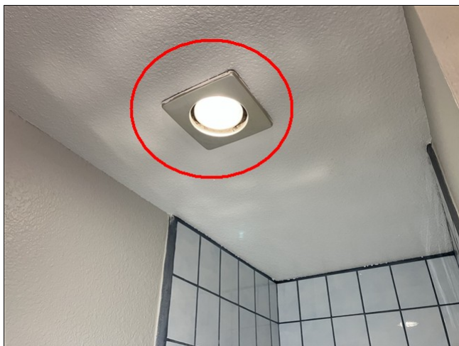
9.1 Item 2(Picture) aged bath exhaust fan
