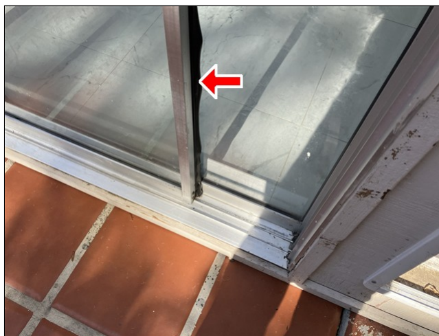
2.1 Item 4(Picture) main floor slider: weather stripping maintenance/repairs needed
