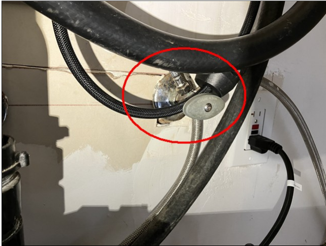
6.4 Item 1(Picture) kitchen: aged water supply valves/hoses observed
