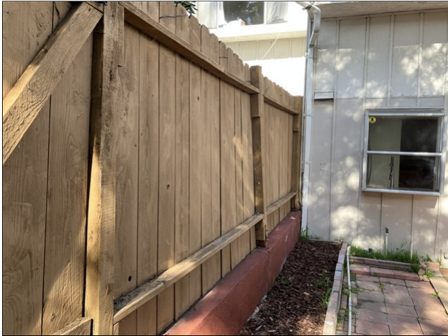
2.6 Item 11(Picture) leaning fence
