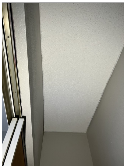
4.8 Item 4(Picture) popcorn texture: materials installed around or before 1978 may contain asbestos
