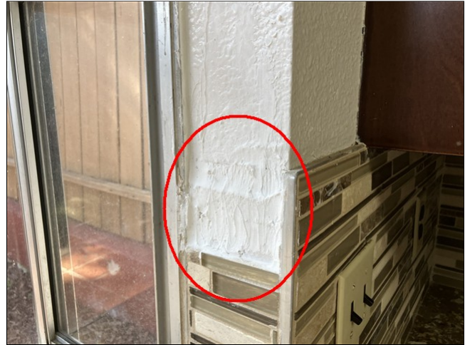
4.8 Item 6(Picture) kitchen wall surface: recommend further evaluation and correction as needed
