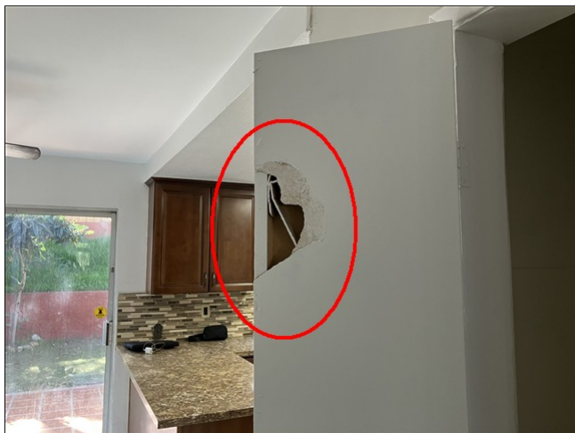
4.3 Item 1(Picture) pantry door near kitchen: maintenance / repairs / or replacement needed
