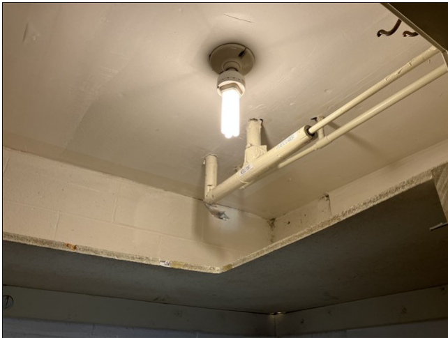
7.5 Item 3(Picture) closet bare-bulb light fixture upgrades recommended
