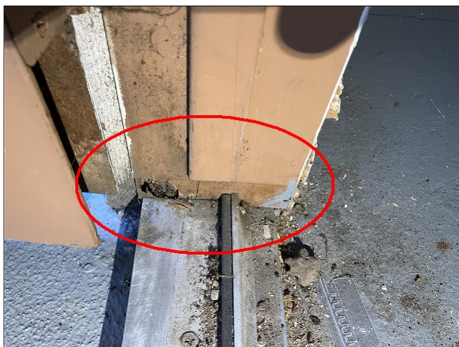
2.1 Item 3(Picture) deck closet door: possible WDO evidence or damage observed
