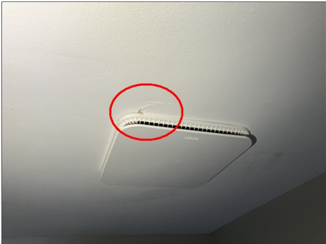
4.0 Item 3(Picture) top level: ceiling surface maintenance/repairs needed
