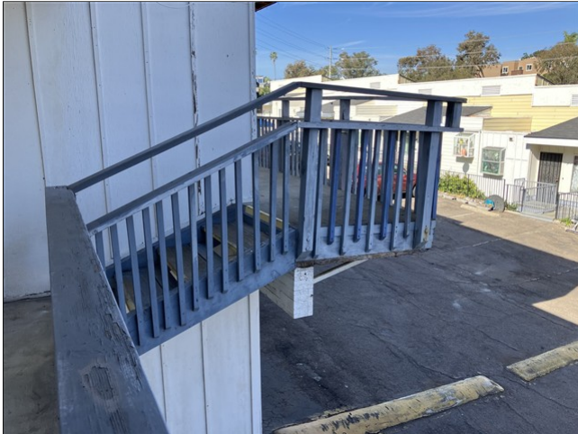
2.6 Item 1(Picture) decks/stairs: possible WDO evidence or damage observed / recommend further evaluation and correction as needed
