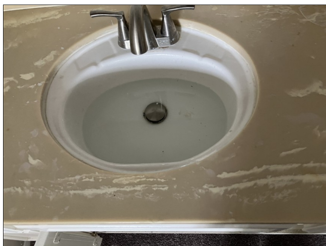
6.3 Item 1(Picture) bathroom: slow drainage observed at the sink
