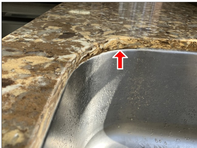
4.4 Item 5(Picture) kitchen: caulking or appropriate sealant maintenance/repairs needed
