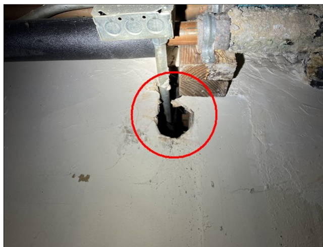
3.1 Item 4(Picture) unsealed penetrations observed in garage firewalls
