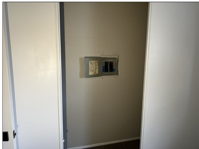
7.2 Item 1(Picture) electrical panel location upgrade recommended
