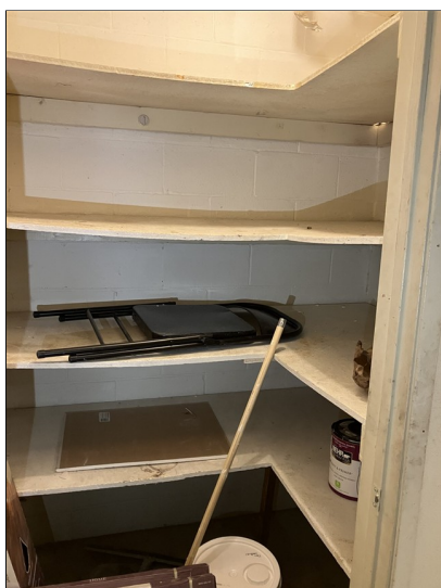
4.4 Item 11(Picture) garage: shelving sagging observed
