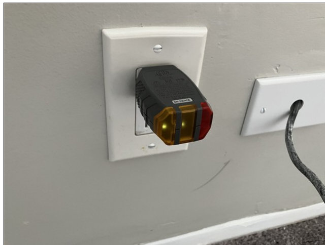
7.5 Item 7(Picture) bedrooms: outlet was still energized when the switch was turned off
