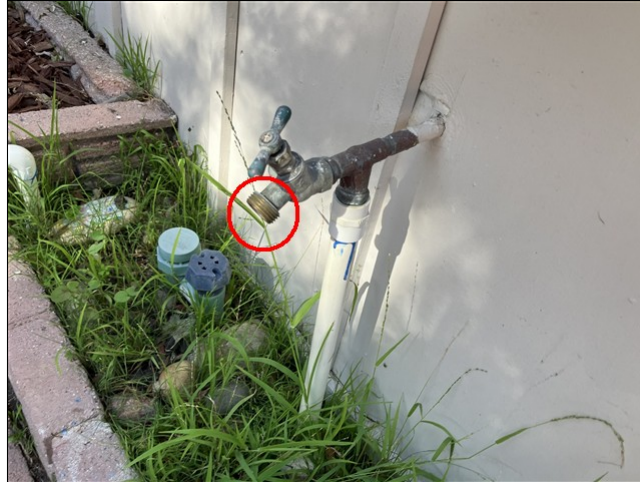
6.4 Item 8(Picture) missing vacuum breaker (anti-siphon device) at exterior spigot(s)
