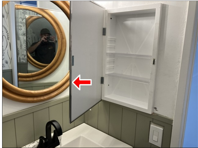
4.4 Item 2(Picture) main floor hall bath: vanity mirror trim was loose
