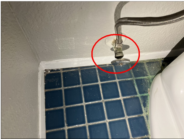
6.4 Item 3(Picture) bathrooms: aged water supply valves/hoses observed
