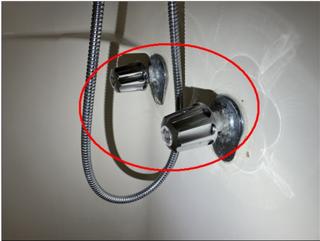
6.5 Item 4(Picture) shower: aged shower valves observed (note: hot and cold orientation are reserved)
