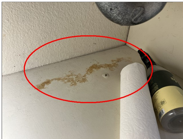
4.4 Item 10(Picture) bedroom bath: moisture stains or damage visible
