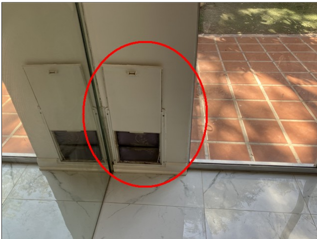
4.0 Item 6(Picture) pet access door observed / recommend further evaluation for removal and wall repair as needed
