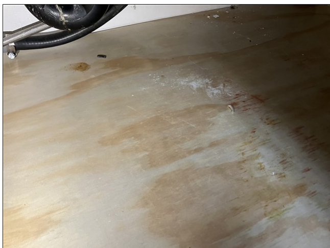
4.4 Item 7(Picture) kitchen cabinet: stains visible at cabinet base
