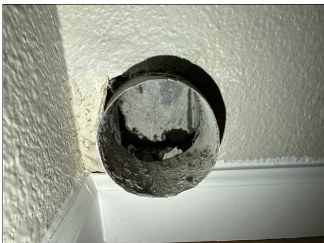
9.1 Item 1(Picture) dryer duct cleaning recommended
