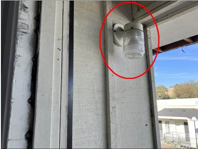
7.5 Item 1(Picture) front entry: switch and corresponding fixture or outlet were not identified
