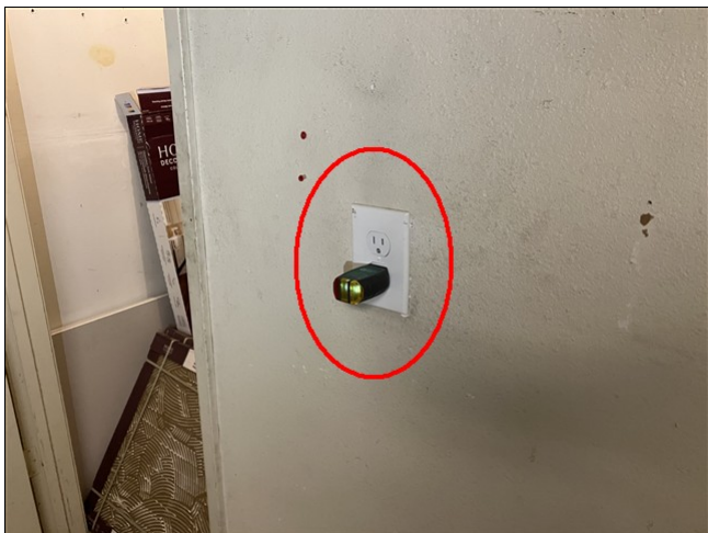
7.6 Item 2(Picture) garage: recommend evaluation and upgrade of any non-GFCI outlets
