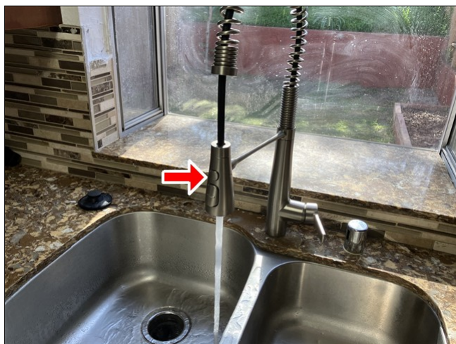
6.5 Item 1(Picture) kitchen faucet: control button did not operate properly when tested
