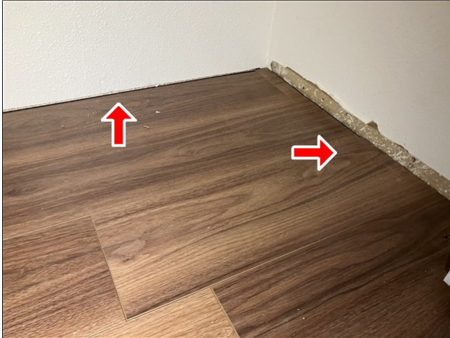
4.1 Item 1(Picture) top level closet: missing baseboard
