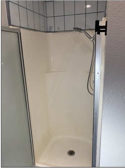
4.6 Item 1(Picture) aged shower enclosure
