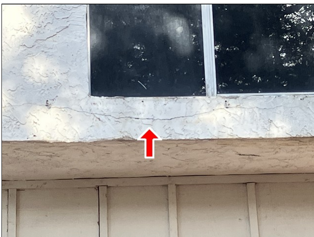
2.6 Item 5(Picture) cracks visible of the stucco
