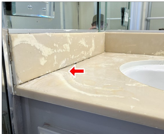
4.4 Item 6(Picture) bedroom bath: caulking or appropriate sealant maintenance/repairs needed
