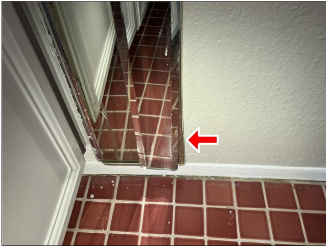
4.0 Item 5(Picture) bedroom bath: loose mirror trim piece
