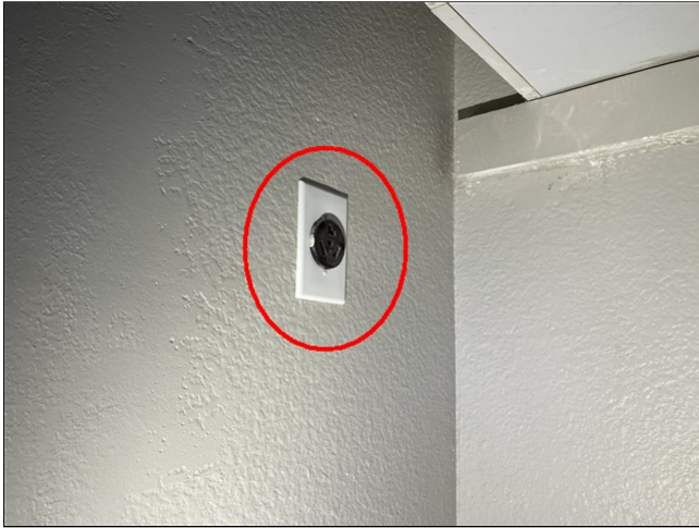
7.4 Item 1(Picture) dryer: outlet upgrade recommended
