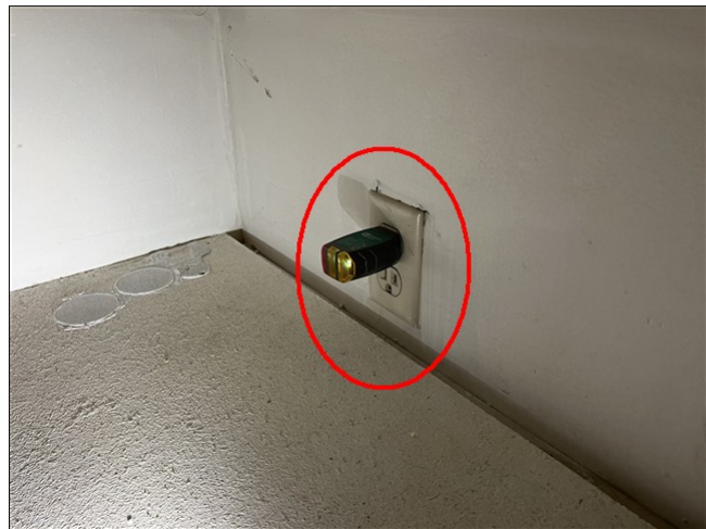
7.6 Item 3(Picture) garage: recommend evaluation and upgrade of any non-GFCI outlets
