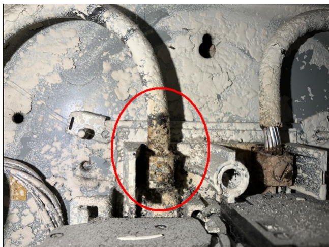
7.3 Item 1(Picture) panel wiring: a performance and safety inspection by a qualified person is recommended
