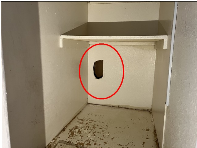
4.0 Item 1(Picture) pantry near kitchen: wall damage visible
