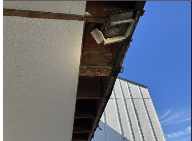
2.6 Item 2(Picture) fascia/soffits: possible WDO evidence or damage observed / recommend further evaluation and correction as needed
