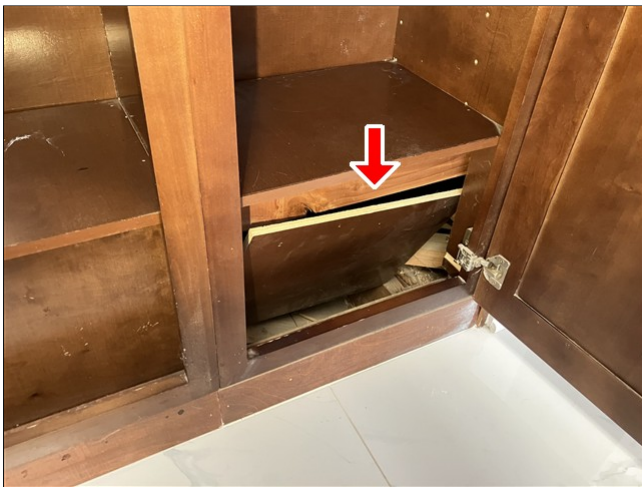
4.4 Item 3(Picture) kitchen: cabinetry maintenance/ repairs needed
