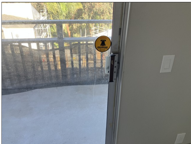
2.1 Item 1(Picture) bedroom slider did not latch properly when tested
