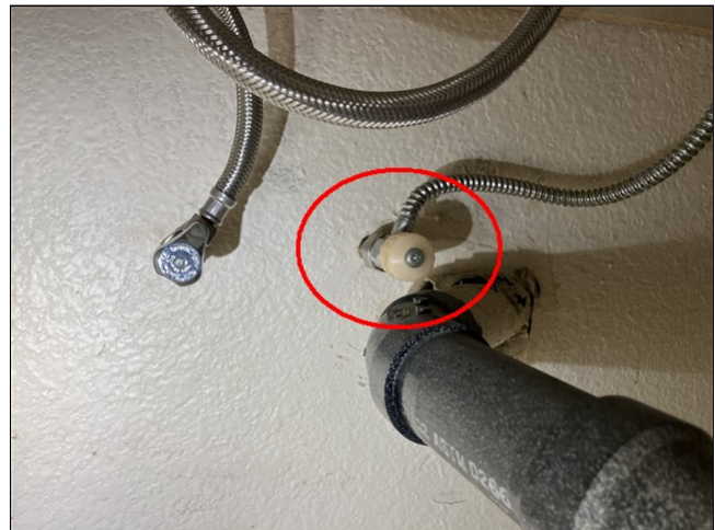
6.4 Item 6(Picture) bathrooms: aged water supply valves/hoses observed
