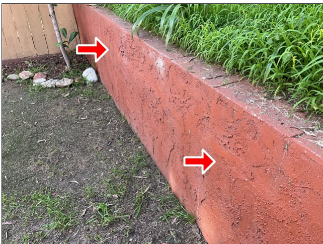
2.6 Item 10(Picture) retaining wall appeared to be leaning / recommend further evaluation and correction as needed
