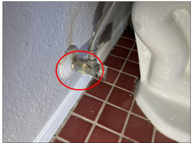
6.4 Item 4(Picture) bathrooms: aged water supply valves/hoses observed
