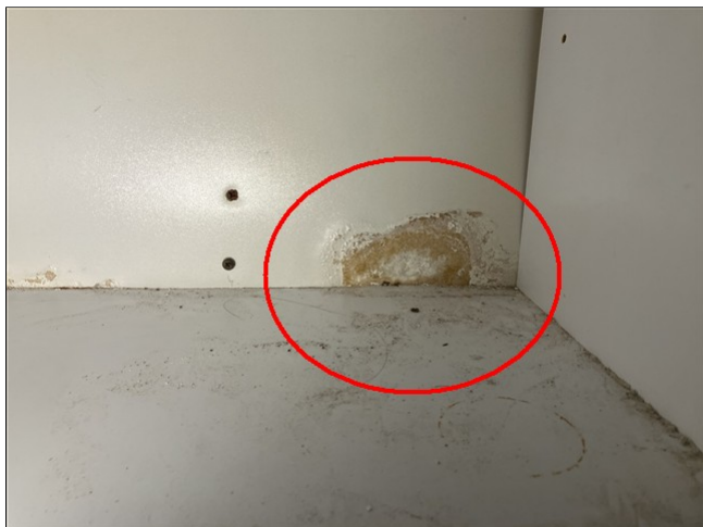
4.4 Item 9(Picture) laundry cabinet: moisture stains or damage visible
