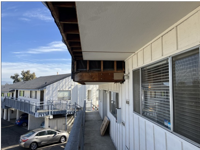
2.6 Item 3(Picture) possible WDO evidence or damage observed / recommend further evaluation and correction as needed
