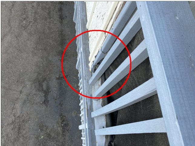
2.3 Item 2(Picture) deck railing: possible WDO evidence or damage observed
