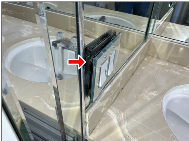
7.5 Item 4(Picture) bedroom bath: loose outlet
