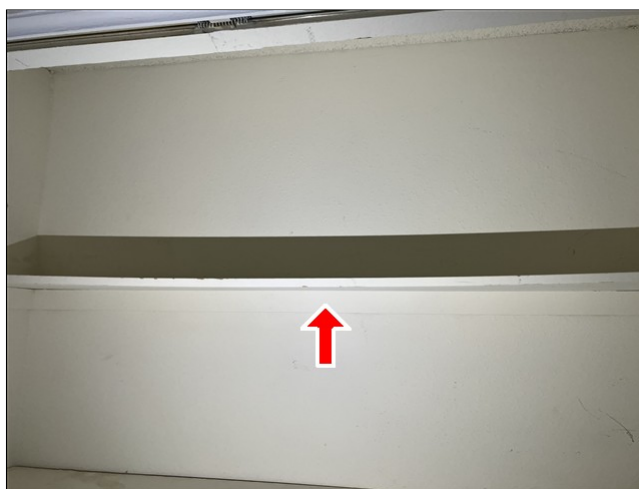
4.4 Item 12(Picture) bedroom: shelving sagging observed
