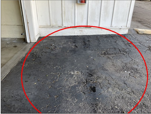
2.6 Item 7(Picture) asphalt maintenance/repairs needed
