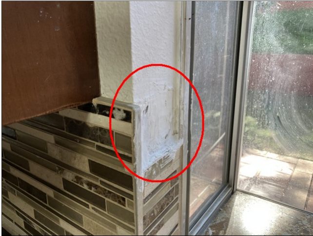
4.8 Item 5(Picture) kitchen wall surface: recommend further evaluation and correction as needed
