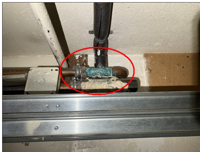
6.4 Item 11(Picture) garage: oxidation visible at water supply pipe
