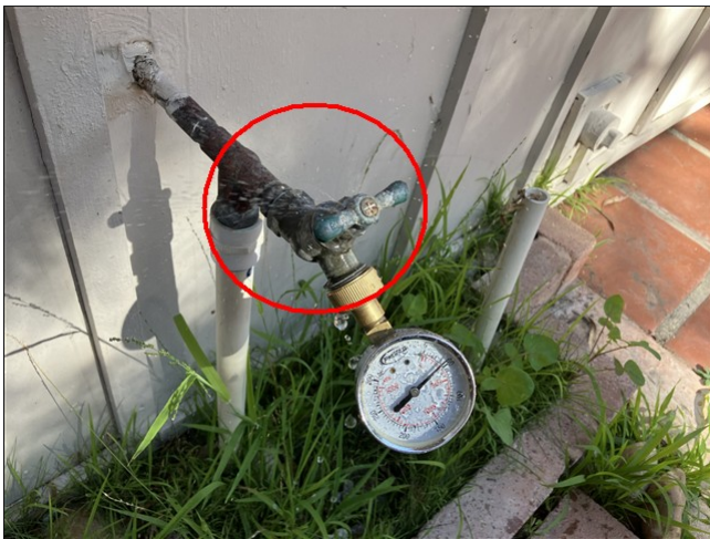
6.4 Item 9(Picture) spigot leaked during testing
