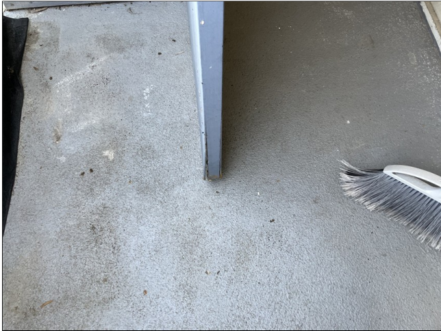
2.3 Item 1(Picture) deck waterproofing appeared aged / recommend further evaluation
