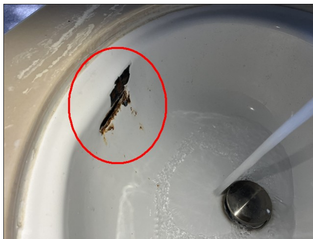
6.5 Item 2(Picture) bedroom sink: oxidation visible // maintenance / repairs / or replacement needed
