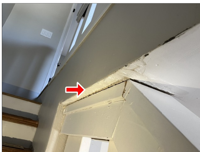
4.8 Item 2(Picture) popcorn texture: materials installed around or before 1978 may contain asbestos
