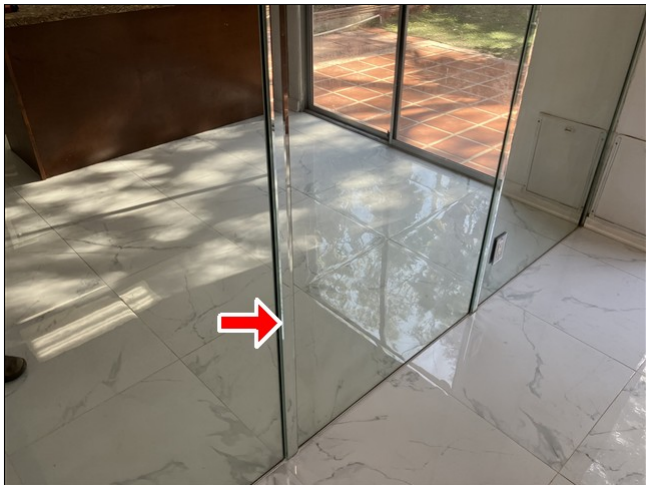
4.0 Item 2(Picture) main floor dining area: mirror trim piece was not properly adhered
