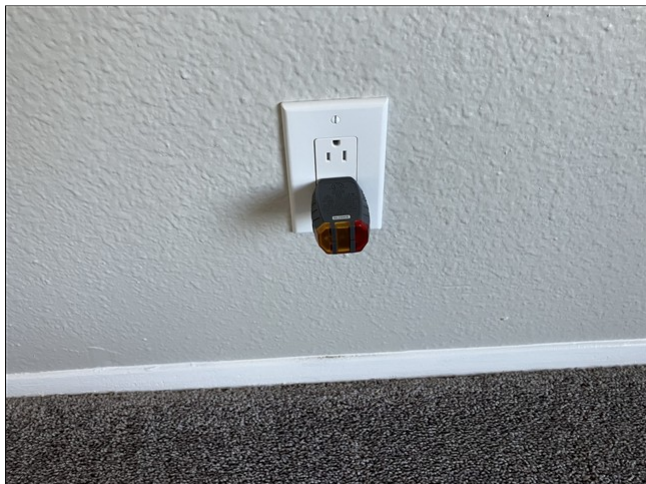
7.5 Item 6(Picture) bedrooms: outlet was still energized when the switch was turned off
