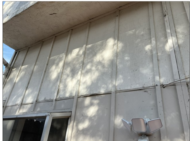
2.6 Item 4(Picture) siding defects observed /maintenance/repairs needed
