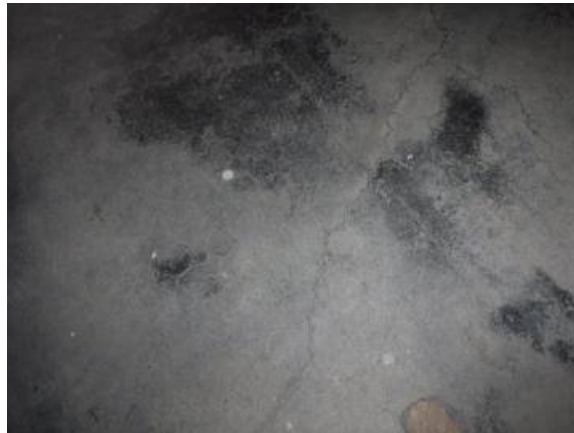
Functional - Hairline crack(s) noted in the floor slab.
