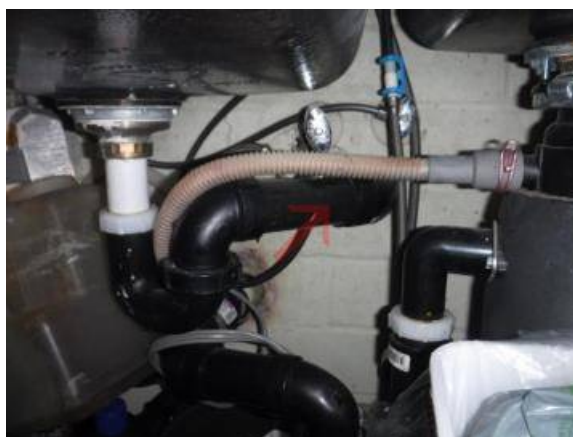
Maintenance - A slightly negative pitch was observed in the drain arm at the kitchen. This condition promotes clogging. Adjustment or repair is recommended to create a positive pitch for proper flow.
