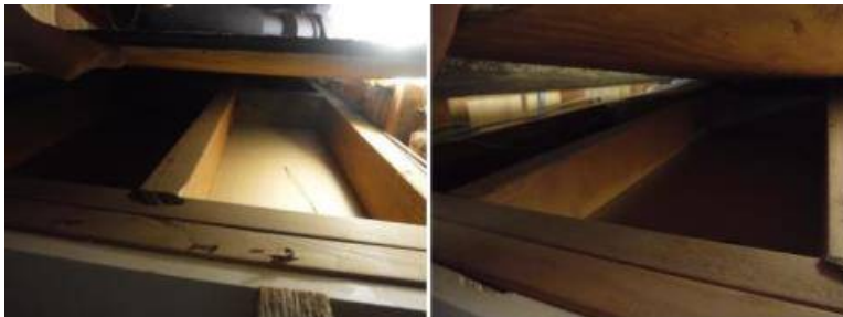
Upgrade - Insulation was not installed in much of the attic. Suggest upgrading by adding insulation in the attic.
