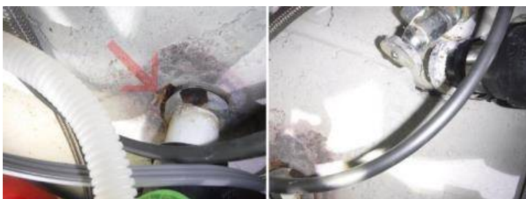
Marginal - The cast iron drain pipes were old. Corrosion was present. Ongoing repairs should be anticipated as this older system continues to age. Replacing the entire system will eventually need to be undertaken.
