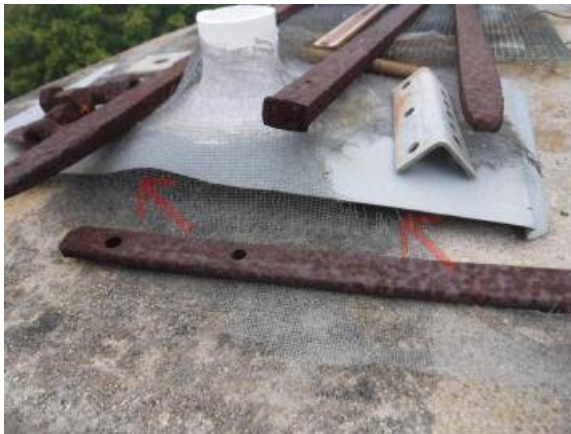
Repair - Metal flashing was improperly installed / was not sealed at the furnace vent.
