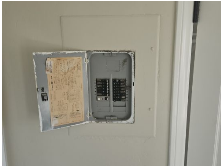
Sub panel location
