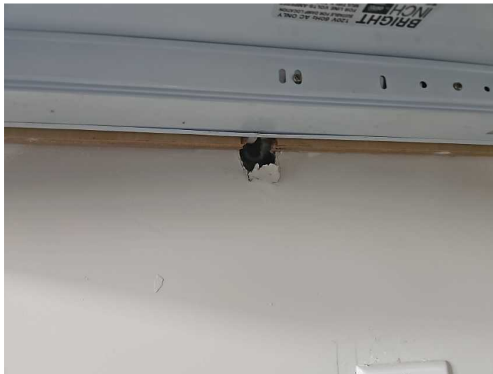
Hole under kitchen cabinet
