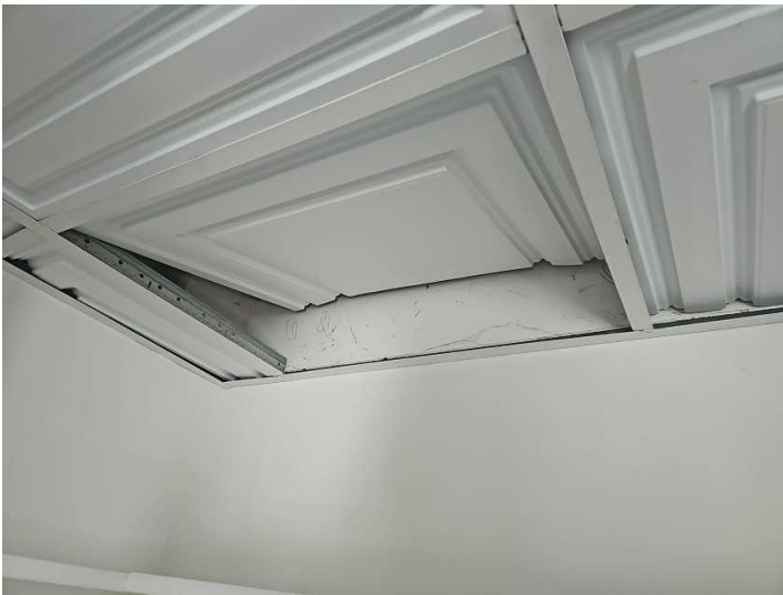
Return air being pulled in through drop down ceiling panel
