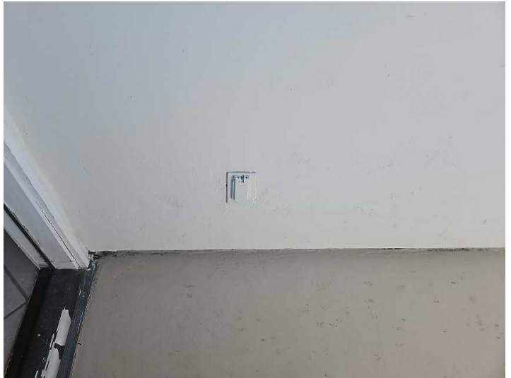
In-use cover not installed
