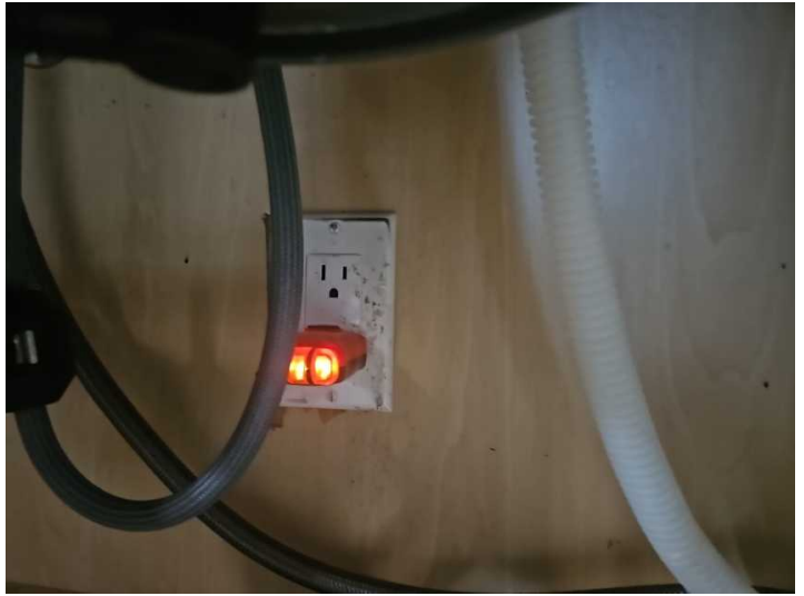
No GFCI present
