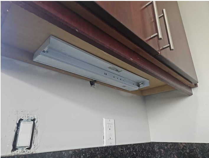
Missing bulb and cover
