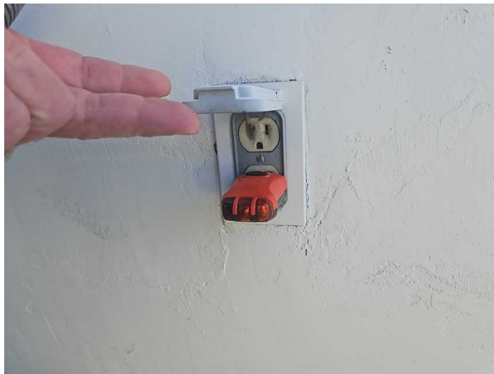
No GFCI present
