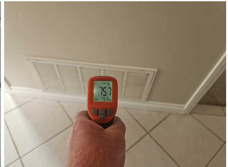
Room temperature at return
