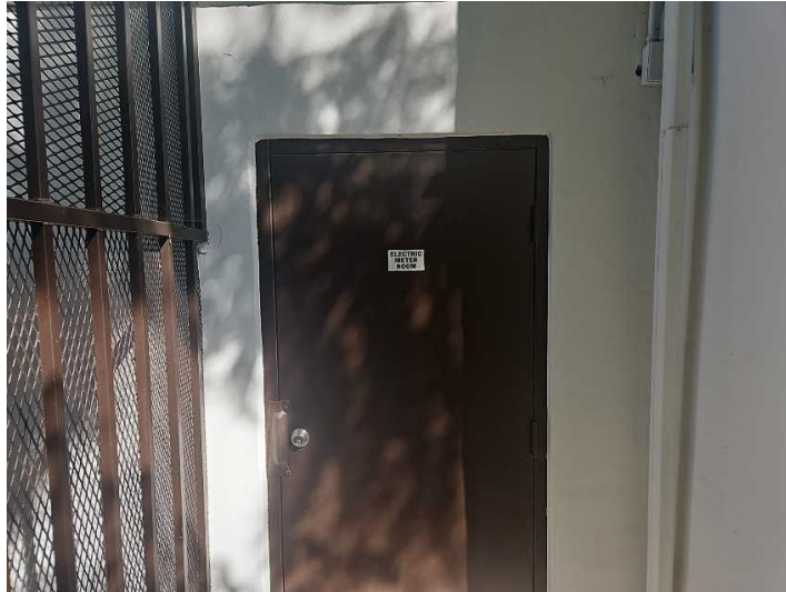
Main panel location
