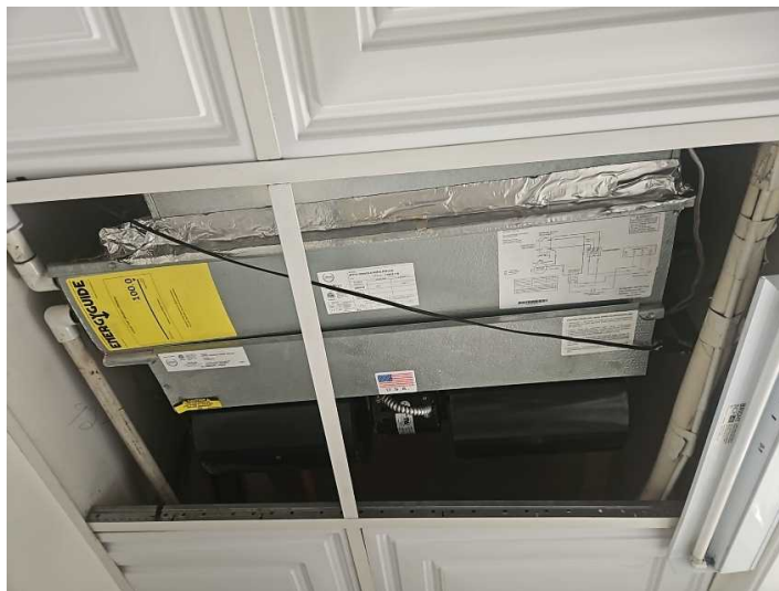
Air handler location
