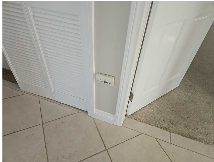
CO detector location
