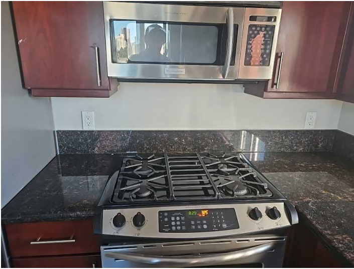
No GFCI present
