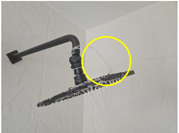
Shower head leaking
