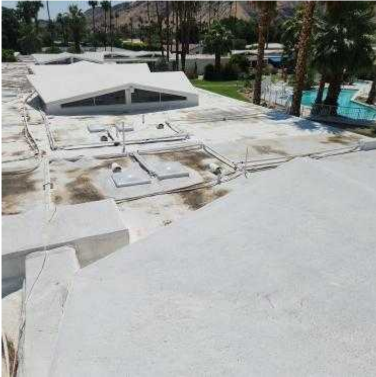
Roof GV-Standing water present (Rained overnight on 6-3-25)
