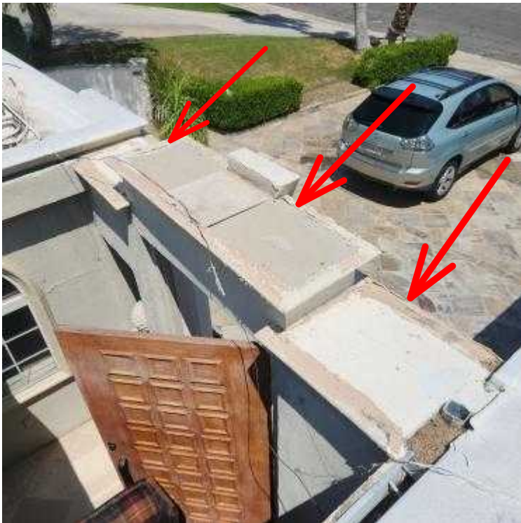
Missing roofing material/flashing cap-Exposed sheathing over portico
