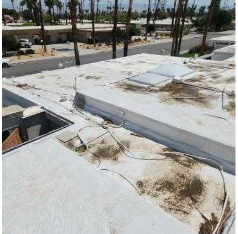
Roof GV-Standing water present (Rained overnight on 6-3-25)
