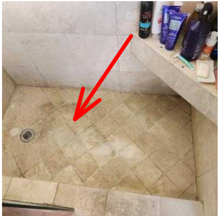
Stained tiles on north bathroom shower pan
