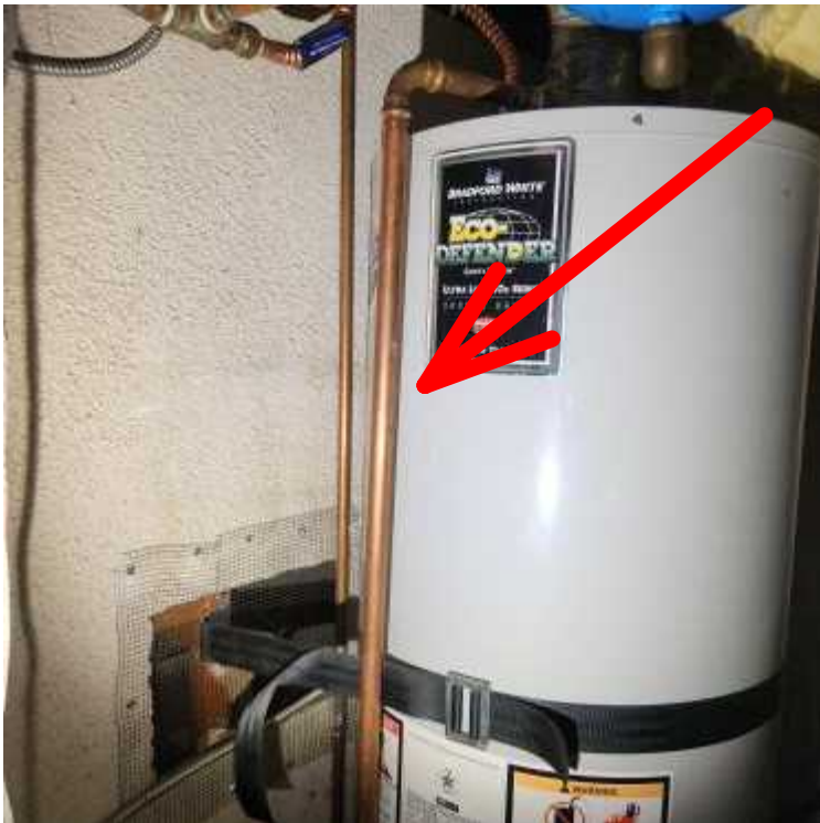
Water Heater TPRV drain tube opening does not extend to exterior-NTBS/Installation of a Watts 210 Valve required
