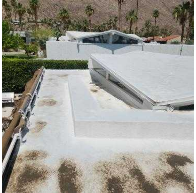
Roof GV-Standing water present (Rained overnight on 6-3-25)
