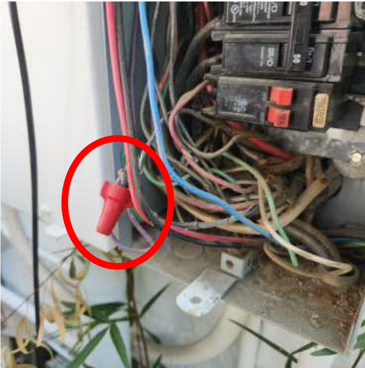
Double tap load wires present inside electrical panel-NTBS
