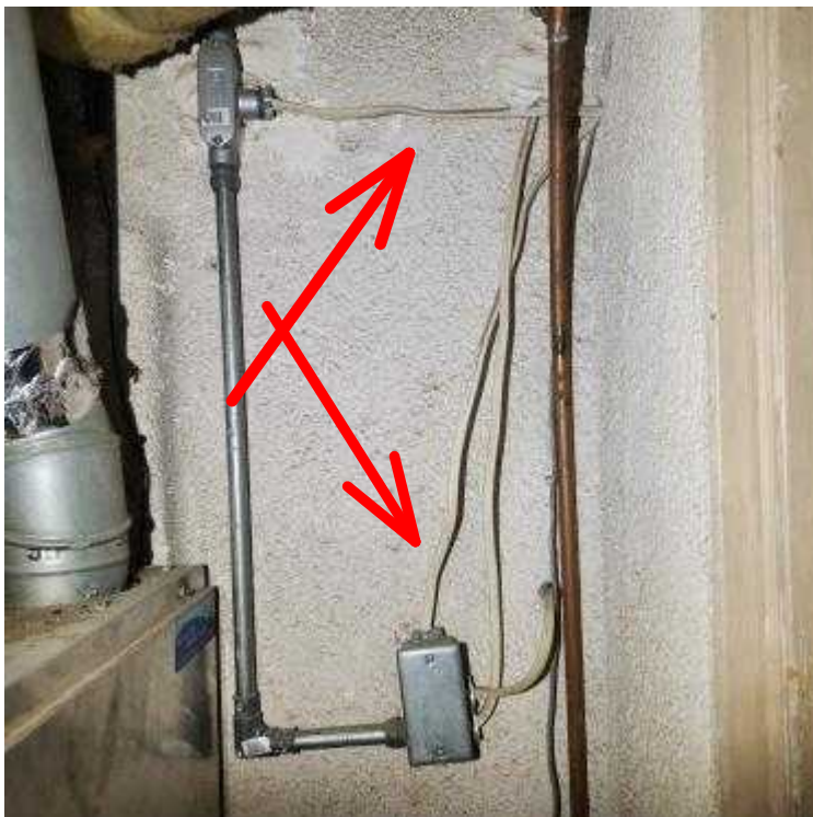
Outlet on south wall inside utility closet separated from box/missing cover plate
