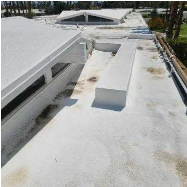
Roof GV-Standing water present (Rained overnight on 6-3-25)
