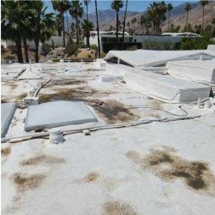
Roof GV-Standing water present (Rained overnight on 6-3-25)
