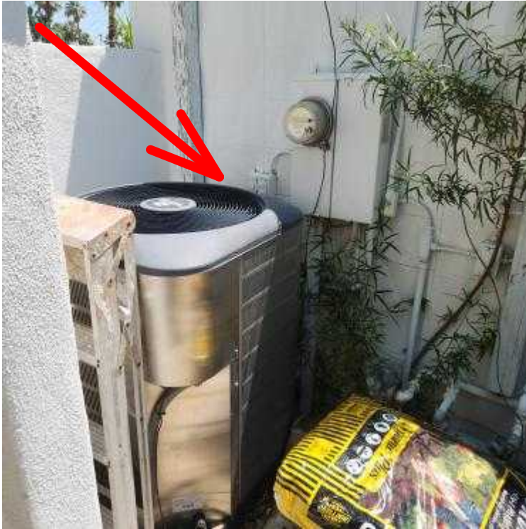
Main electrical panel/meter does not have required 36 inch out by 30 inch wide working space-NTBS
