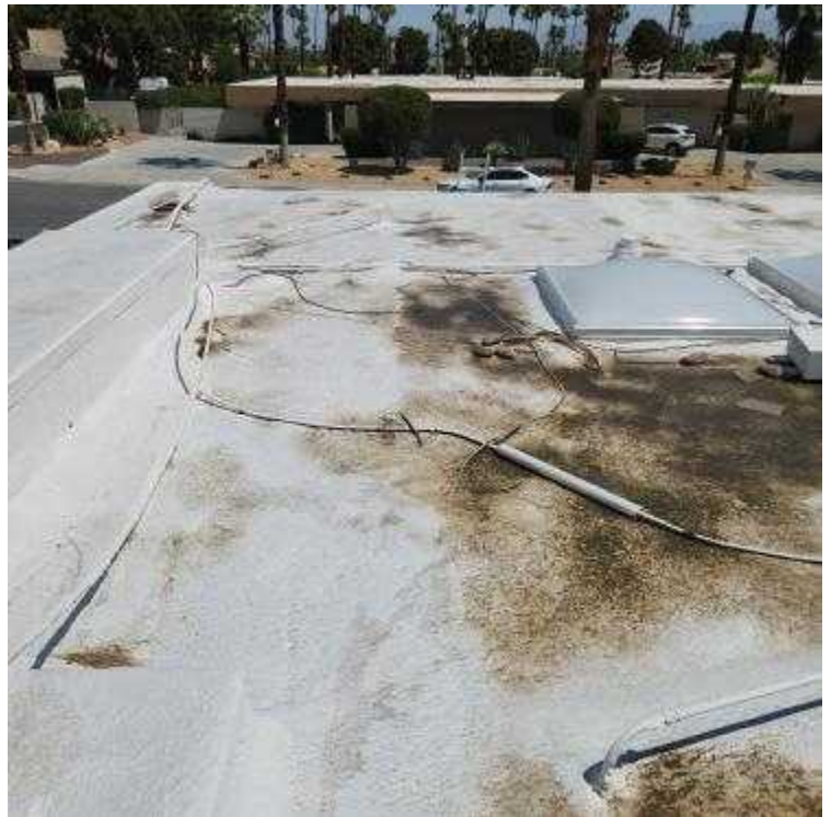
Roof GV-Standing water present (Rained overnight on 6-3-25)
