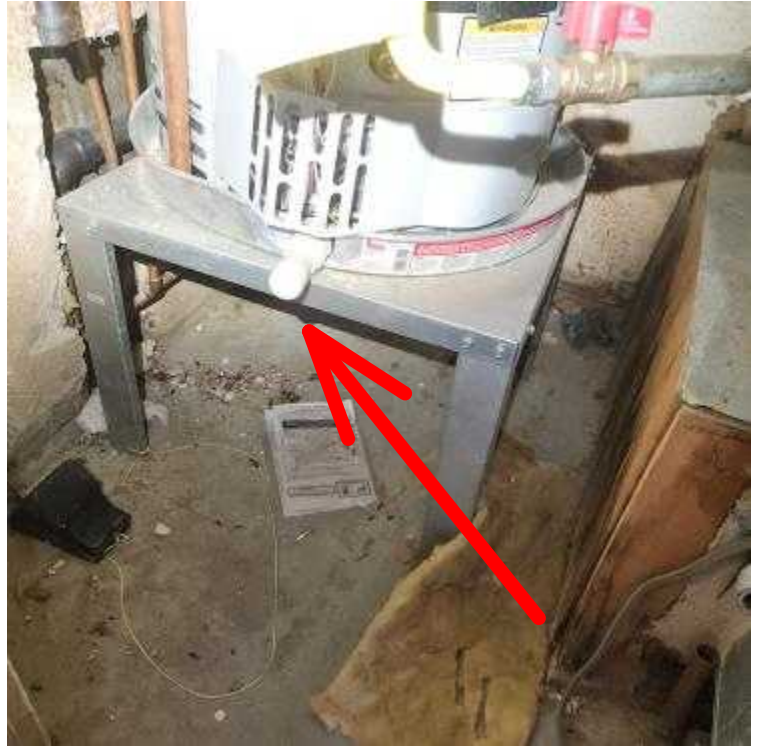
Missing drain pipe from catch pan under water heater-NTBS
