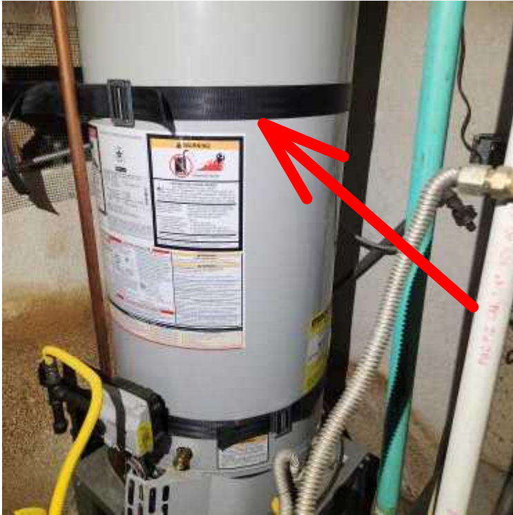
Improper strapping installation on water heater-Upper strap placed too low on casing-NTBS
