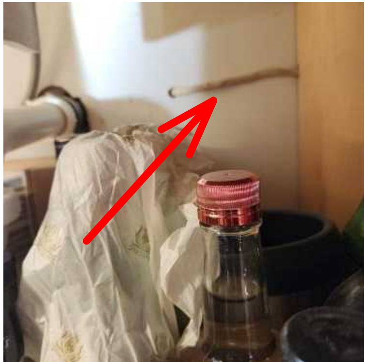
Exposed wiring on east wall inside cabinet below sink-NTBS
