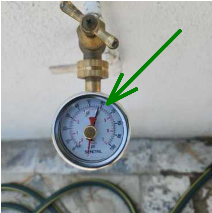
Water Pressure at house is 60 PSI
