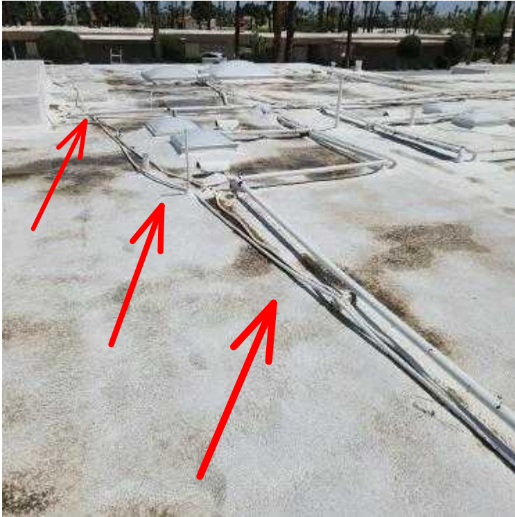
Multiple electrical conduit laying on roof surface-NTBS
