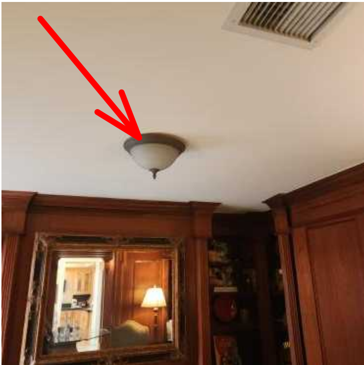
Inoperative fixture/bulb on ceiling in den
