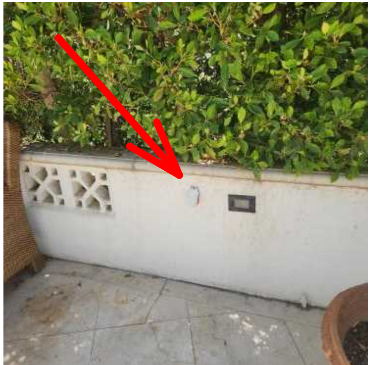
GFCI outlet on south wall on south patio did not trip-NTBS
