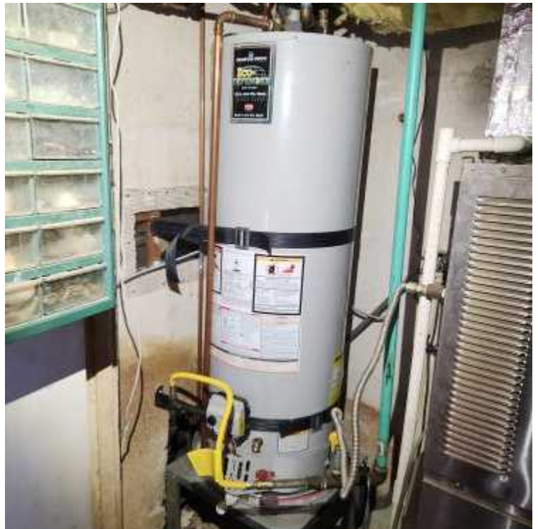
Water Heater operated properly (50 gallon 2023 model located in utility closet)
