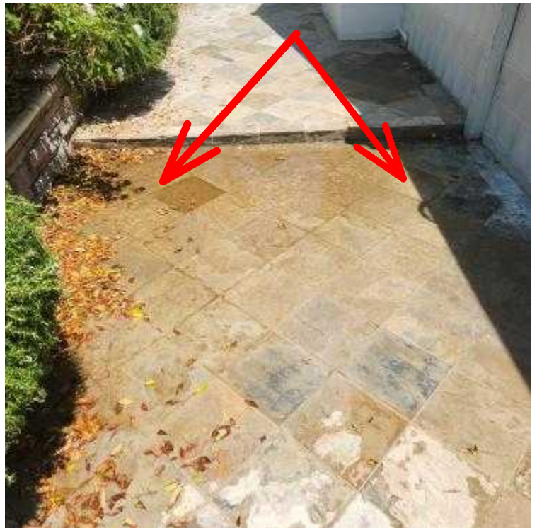
Standing water present on west side of house-Installation of drains recommend
