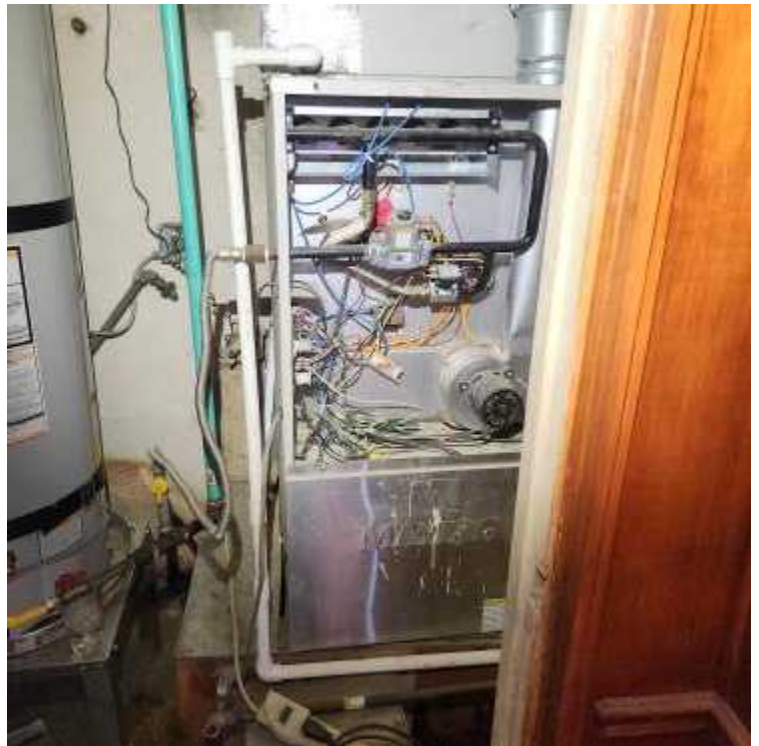
Heater operated properly (120k BTU 2011 model located in utility closet)
