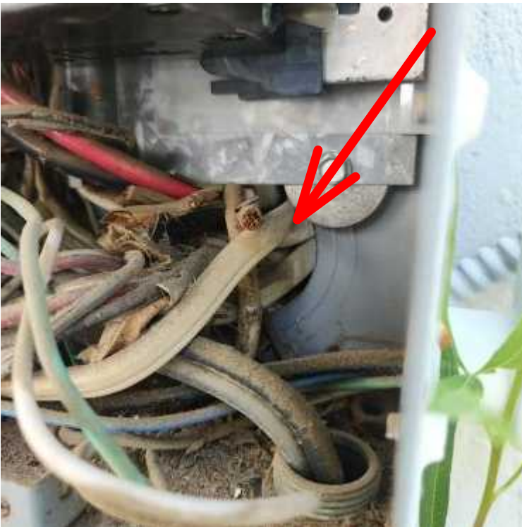
Missing anti-chafe bushing around wires inside electrical panel-NTBS
