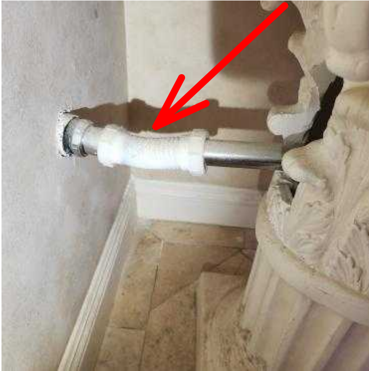
Improper material used for section of drain pipe below north sink in primary bathroom-NTBS/Accordion flexible type present
