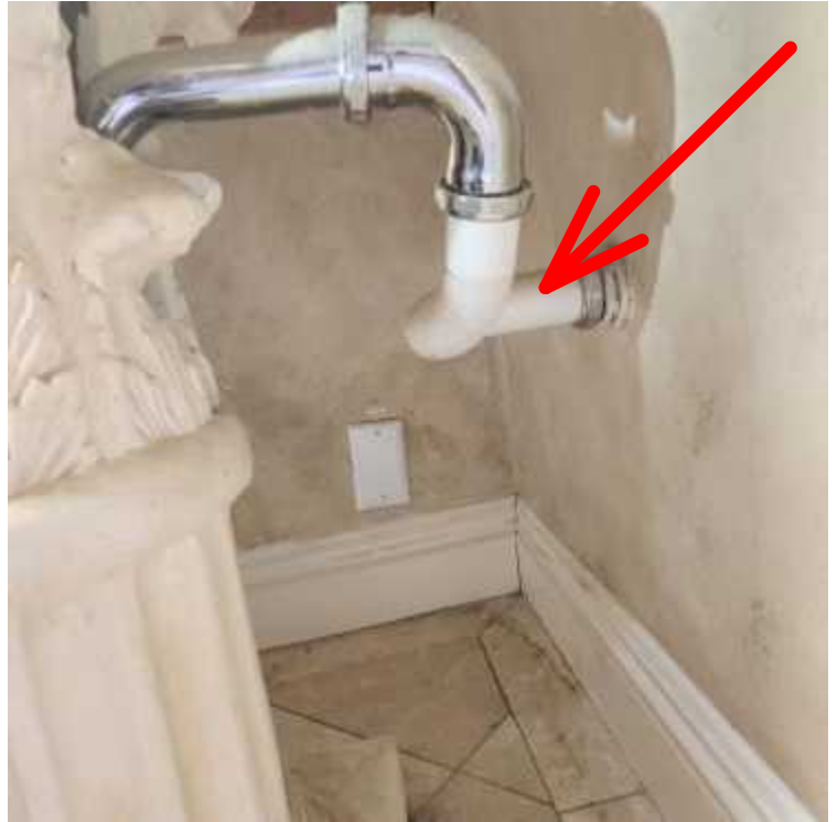
Improper material used for section of drain pipe below south sink in primary bathroom-NTBS/Accordion flexible type present
