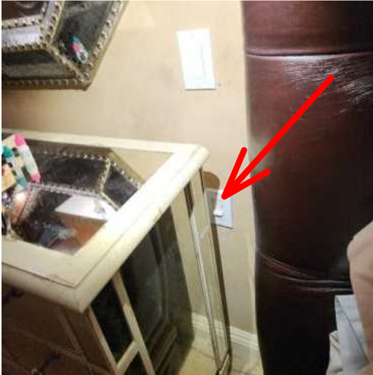
(1) Damaged dimmer switch on east wall in primary bedroom
