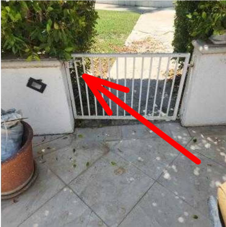
Gate on south patio does not align/latch
