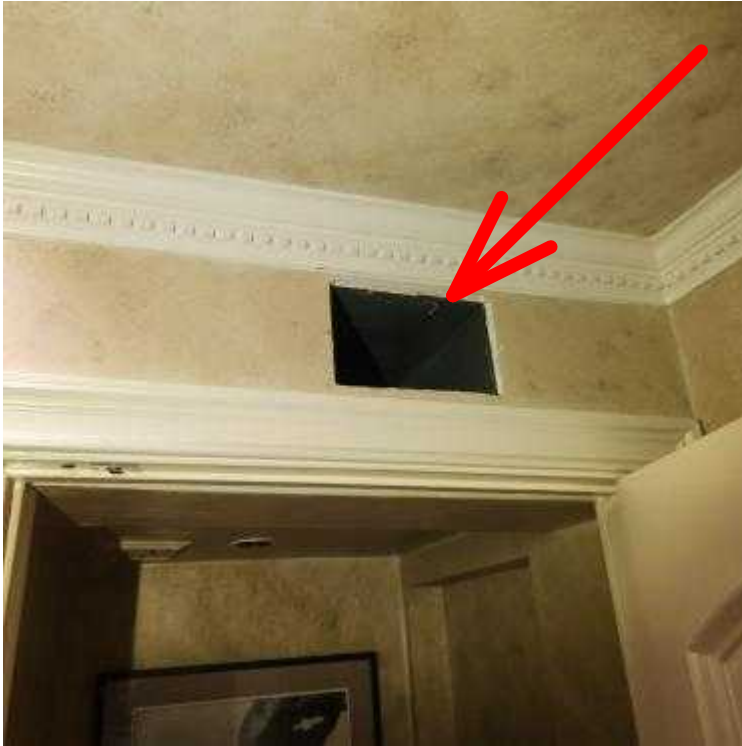
Missing HVAC register cover on wall in primary bathroom
