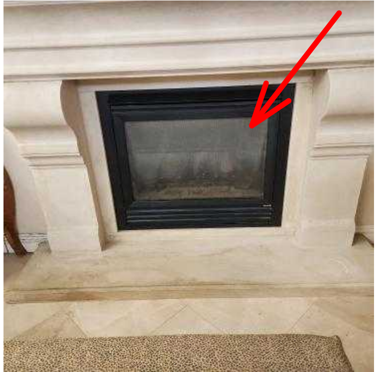
Fireplace not tested at time of inspection-Unable to locate remote
