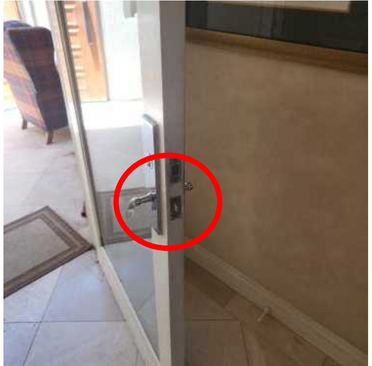
Lockset on entry door to house worn/does not function properly
