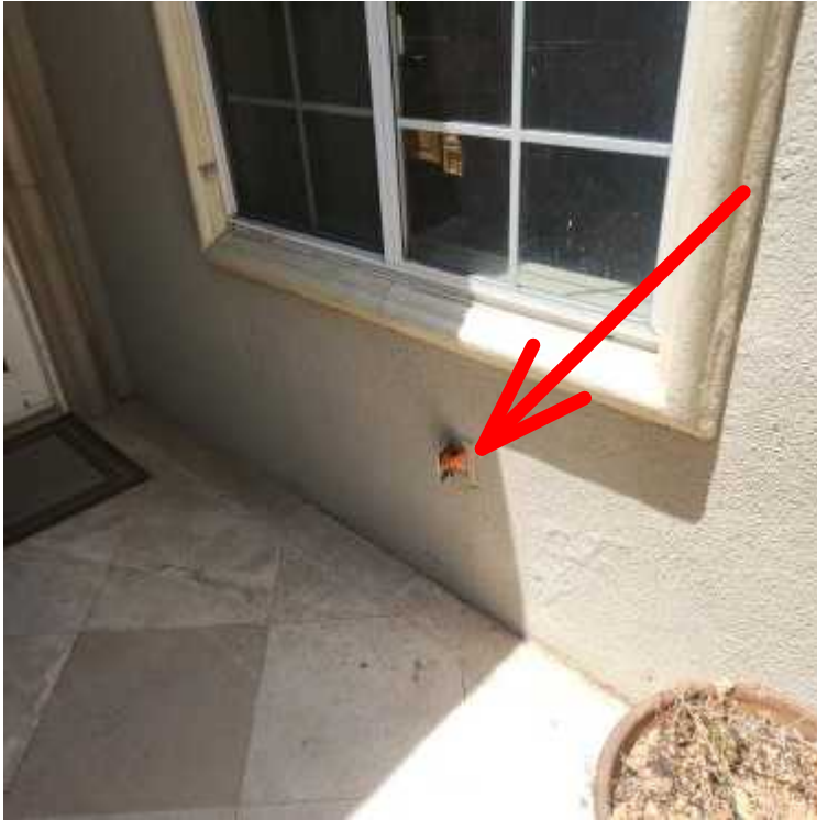
GFCI outlet on west wall in courtyard did not trip-NTBS
