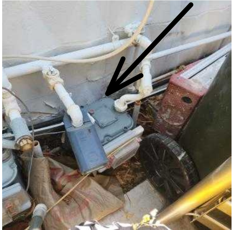
Gas meter to property GV (Located on west side of house)
