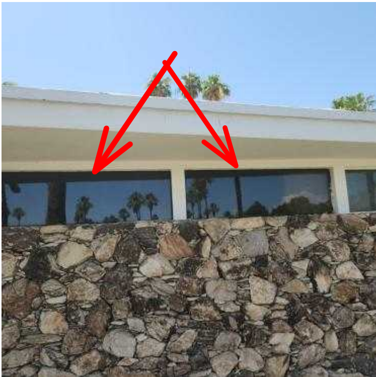
Missing exterior glazing strip to (2) windows on north side of house
