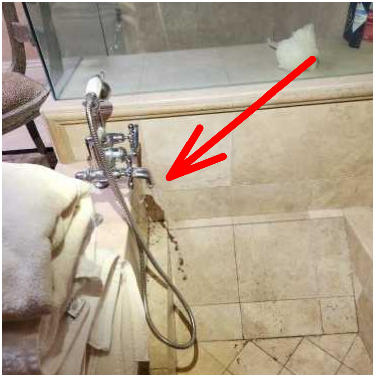
Low water flow from primary bathroom tub faucet-Faucet worn & drips continuously
