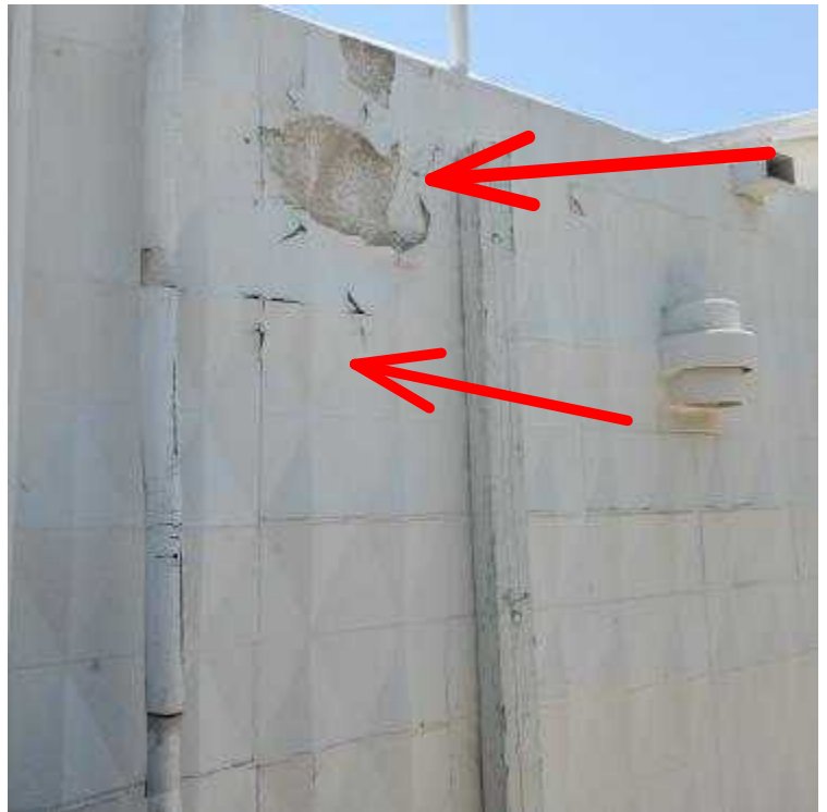
Cracking/Peeling paint on west side of house
