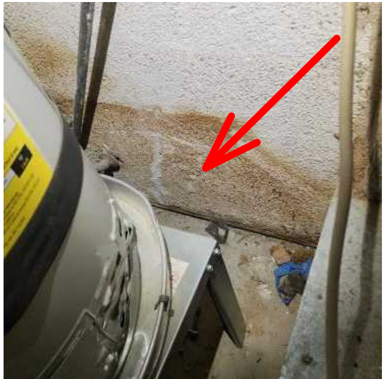
Dry moisture stains present on interior walls in utility closet
