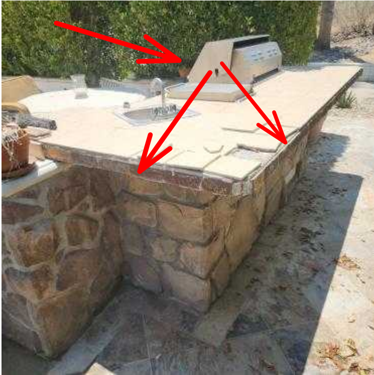
Igniter to BBQ on south patio inoperative, Multiple broken/missing tiles on BBQ structure
