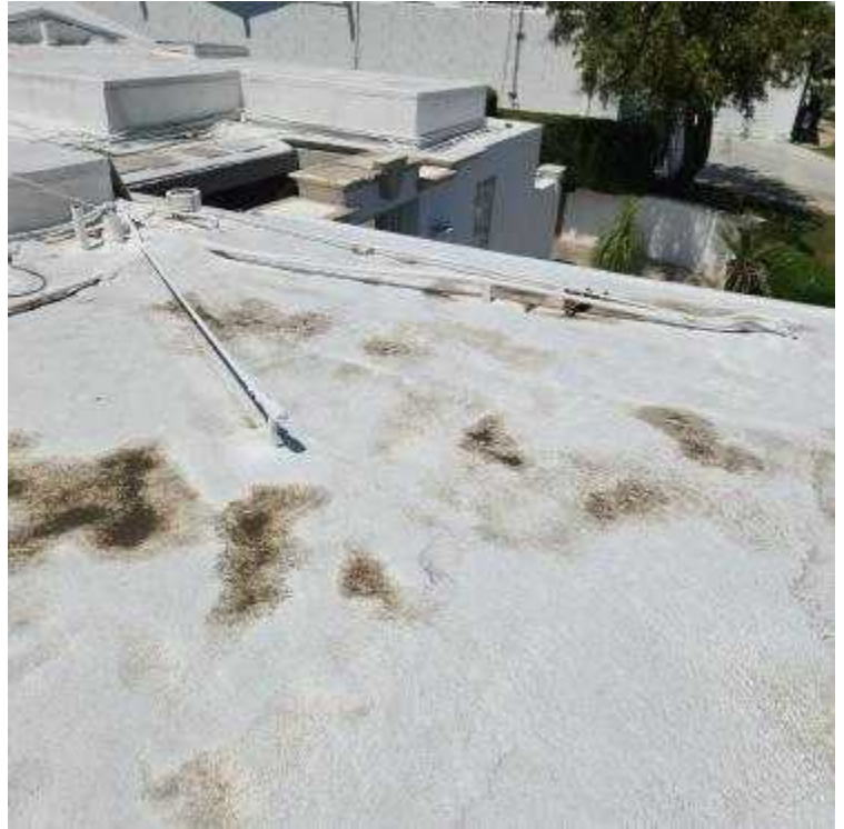
Roof GV-Standing water present (Rained overnight on 6-3-25)
