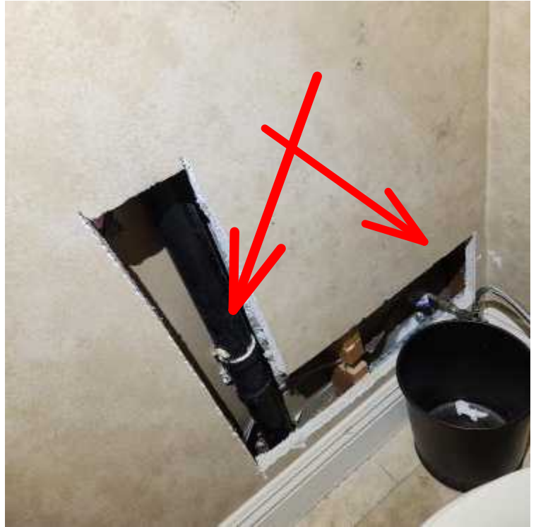
Hole present/Missing drywall in primary bathroom on wall in toilet room
