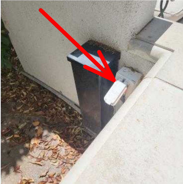
Dead north outlet on north wall on south patio
