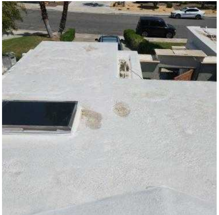
Roof GV-Standing water present (Rained overnight on 6-3-25)
