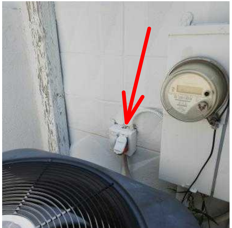
North exterior outlet on west side of house not GFCI protected-NTBS
