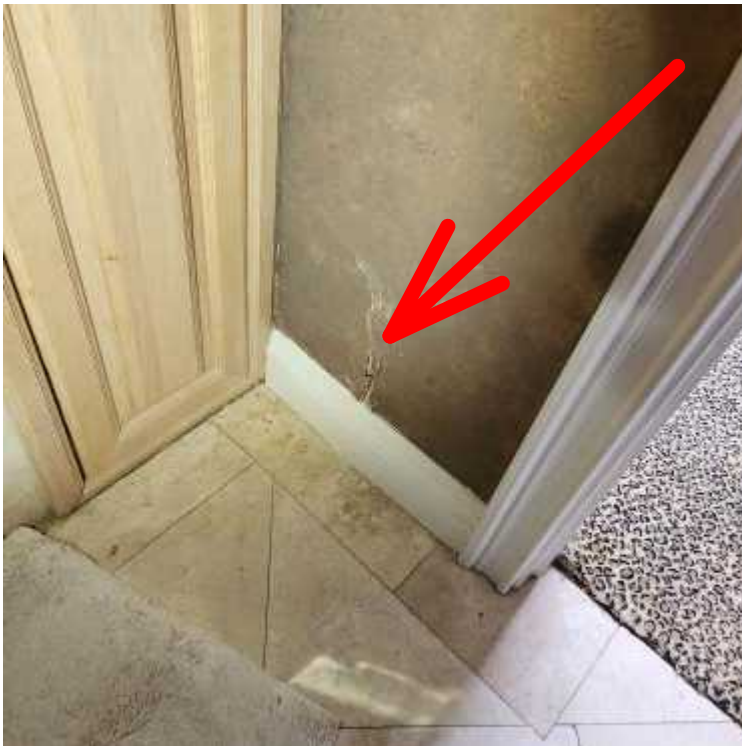
Damaged drywall on east wall in north bathroom
