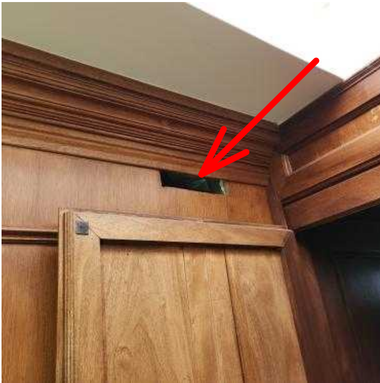
Missing HVAC register cover on west wall in office
