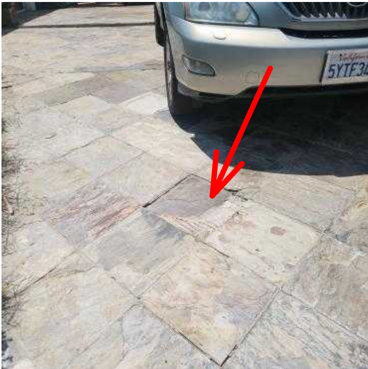
Broken/Missing tiles in driveway
