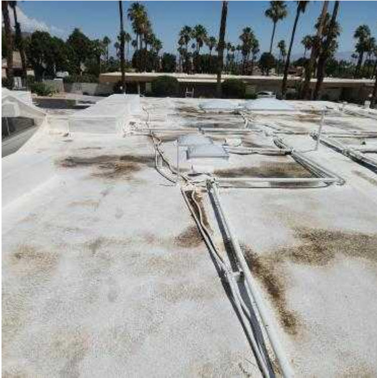
Roof GV-Standing water present (Rained overnight on 6-3-25)
