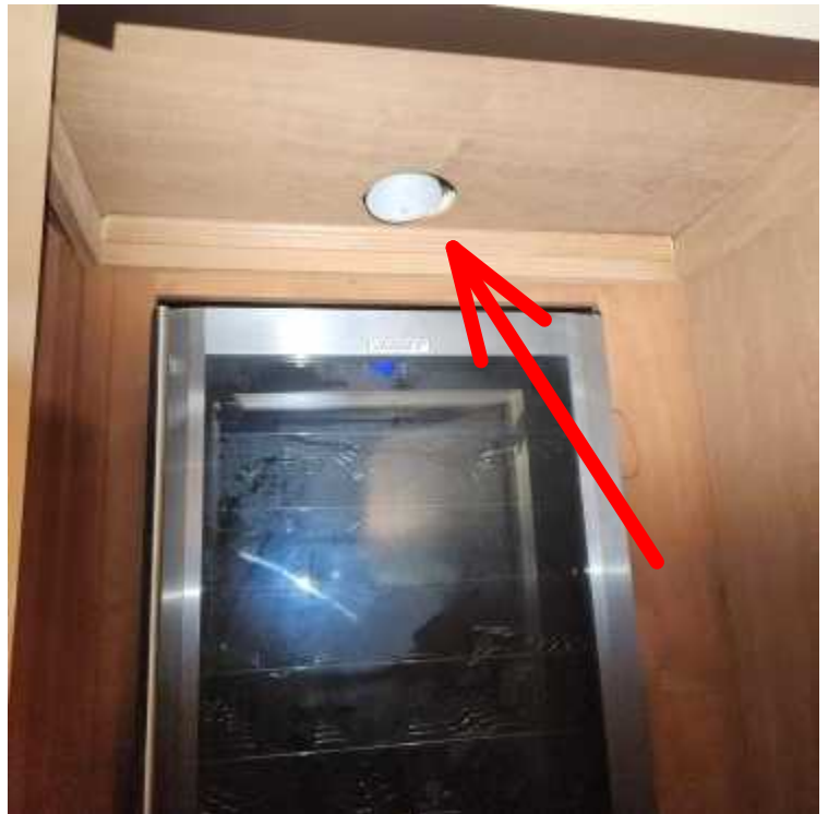
Inoperative fixture/bulb on ceiling in wine closet
