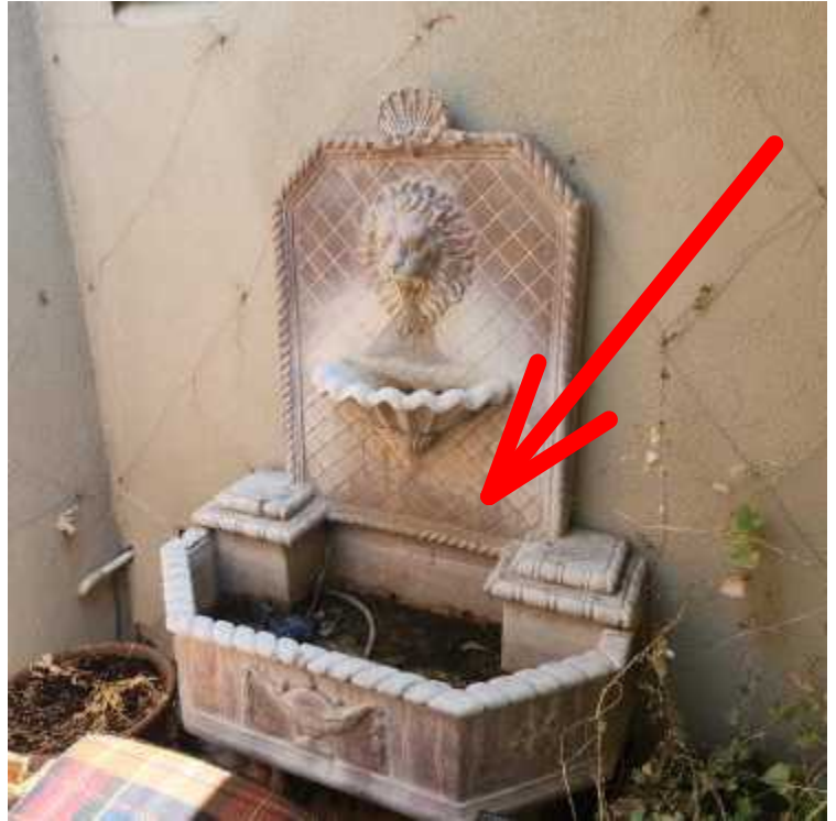
Water Feature in courtyard has inoperative pump at time of inspection
