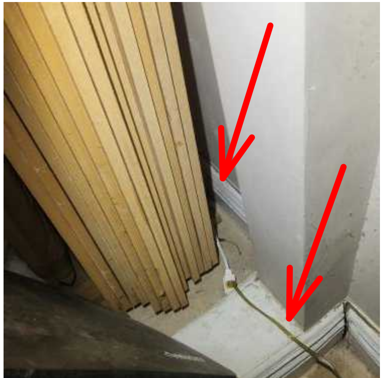
Moisture damage present to baseboard in areas on west wall in living room
