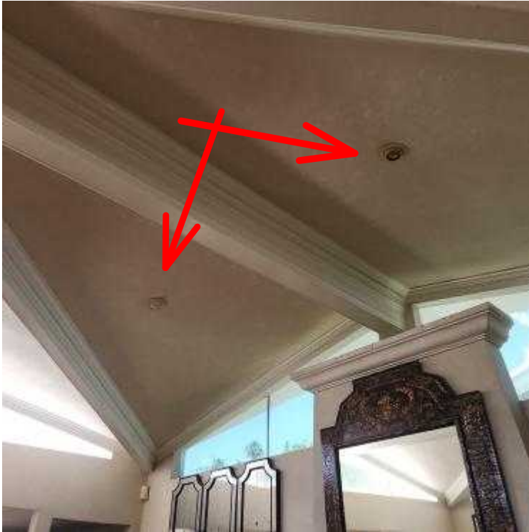
(2) Inoperative fixtures/bulbs on ceiling in living room
