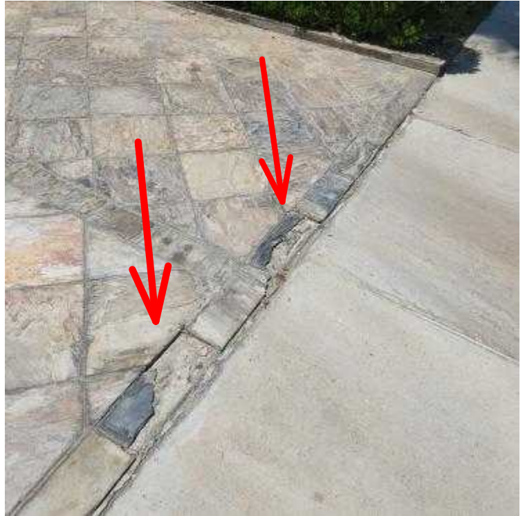
Broken/Missing tiles in driveway
