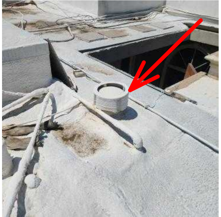
Vent pipe on roof to water heater & heater does not extend a minimum of 12 inches above roof surface-NTBS
