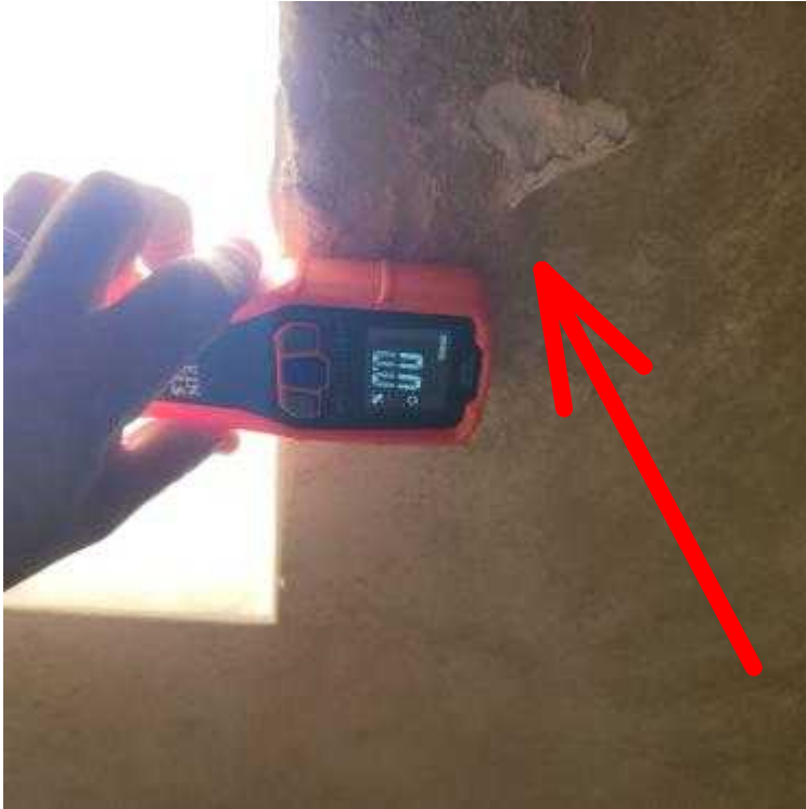
Dry moisture damage on primary bathroom ceiling adjacent to skylight-Evidence of past roof leak
