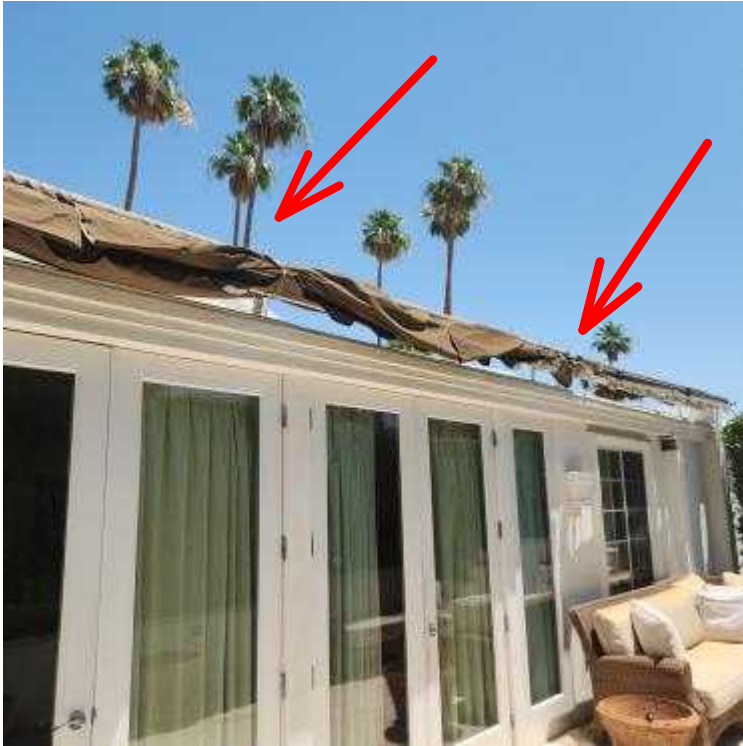
(2) Electric Awnings on south side of house damaged/unable to test at time of inspection
