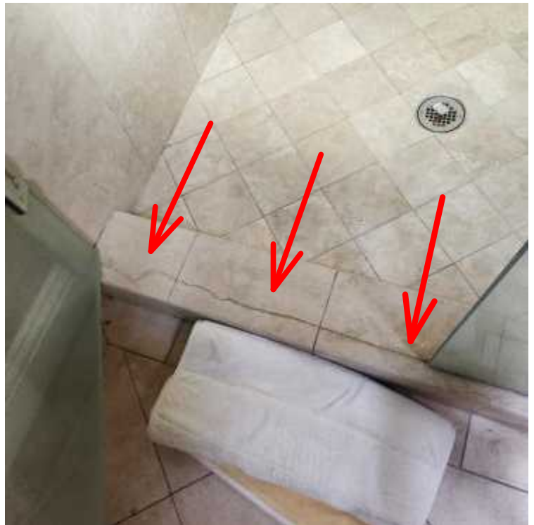
Cracked tiles on primary bathroom shower pan step
