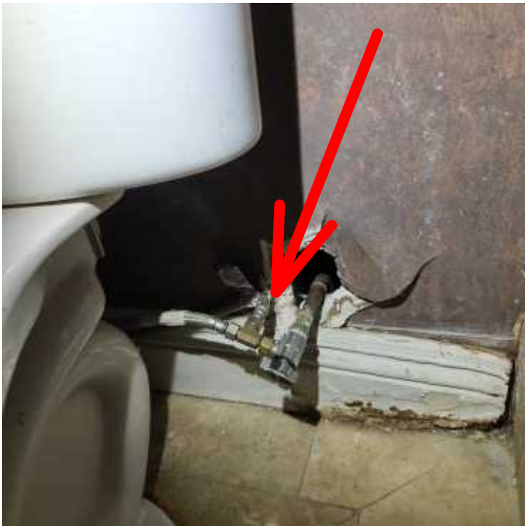
Cold water supply to north bathroom sink faucet has been abandoned-Using toilet supply pipe for cold water water to sink
