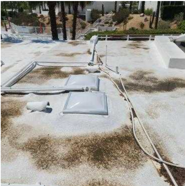
Roof GV-Standing water present (Rained overnight on 6-3-25)
