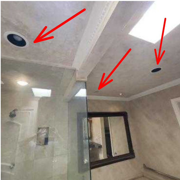
(3) Inoperative fixtures/bulbs on ceiling in primary bathroom
