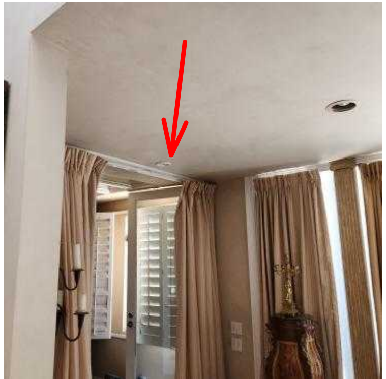
Missing smoke & carbon monoxide alarm outside bedroom-NTBS
