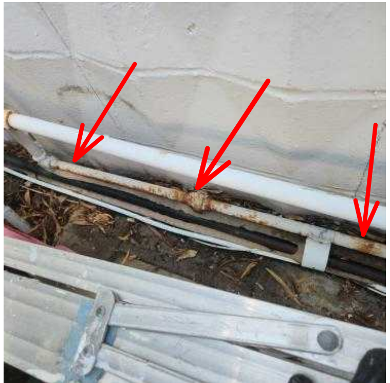
Rusted pipes on/from gas meter
