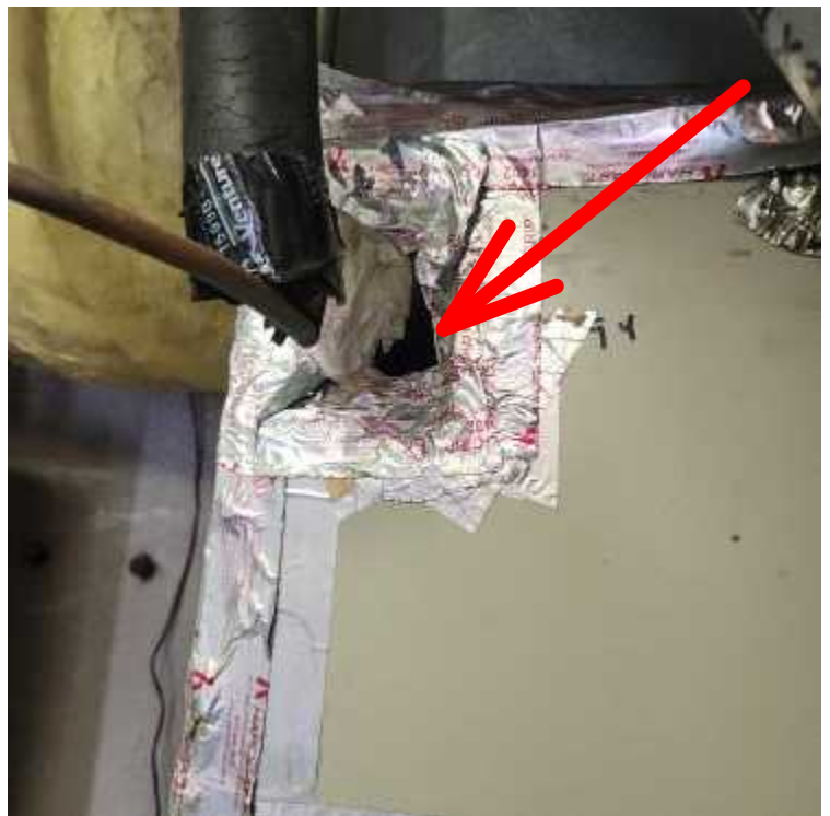
Air leaking from coil on heater
