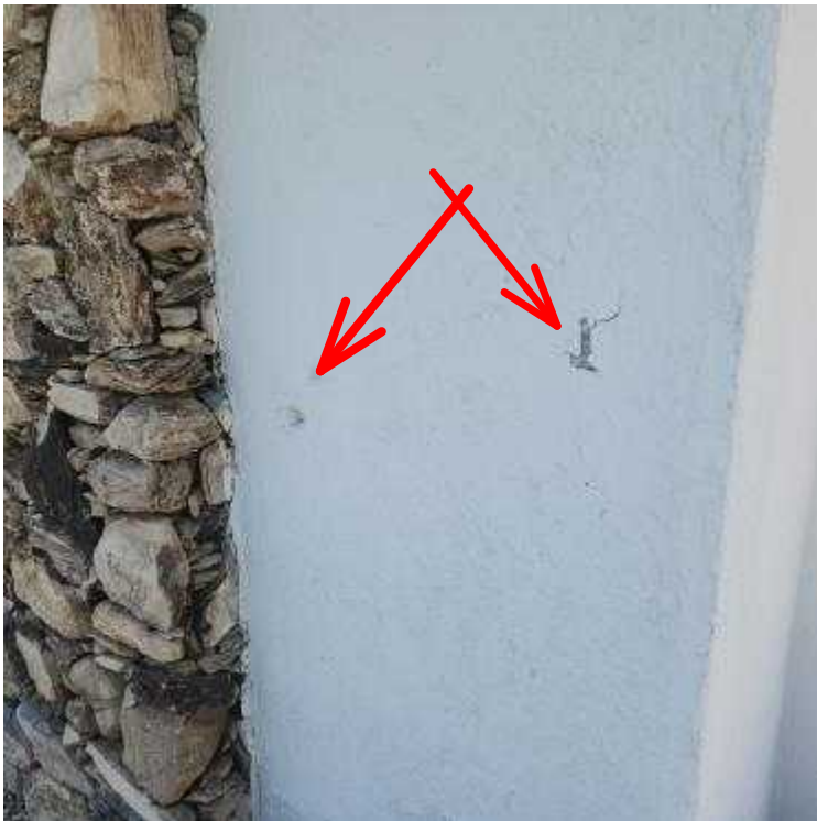
Chipped/Peeling stucco top coat in areas on north side of house
