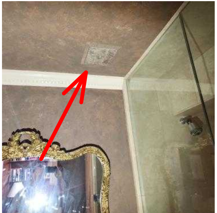
Inoperative exhaust fan in north bathroom-NTBS
