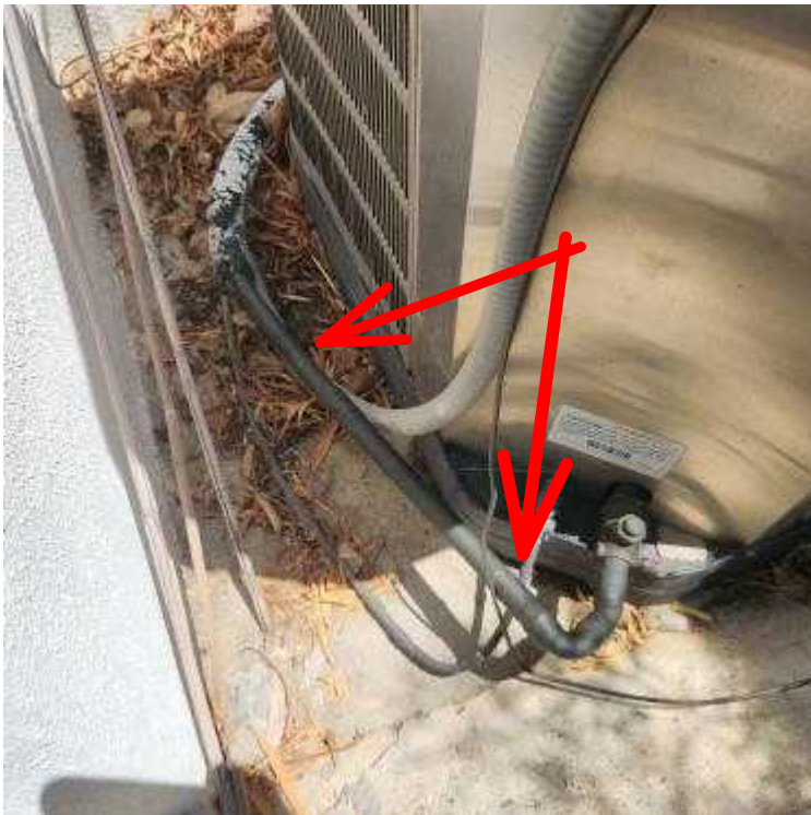
Missing insulation/Exposed copper on refrigerant pipe to AC Condenser
