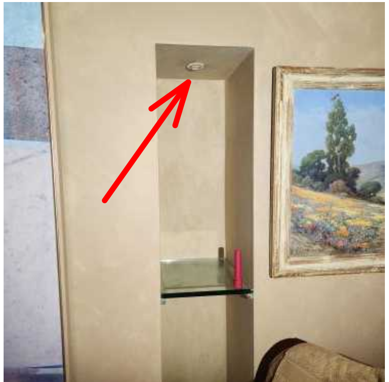
Inoperative fixture/bulb in north wall niche in primary bedroom
