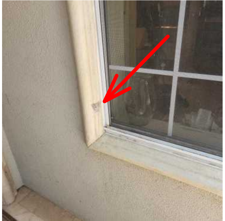
Chipped window trim/Exposed foam on west wall in courtyard
