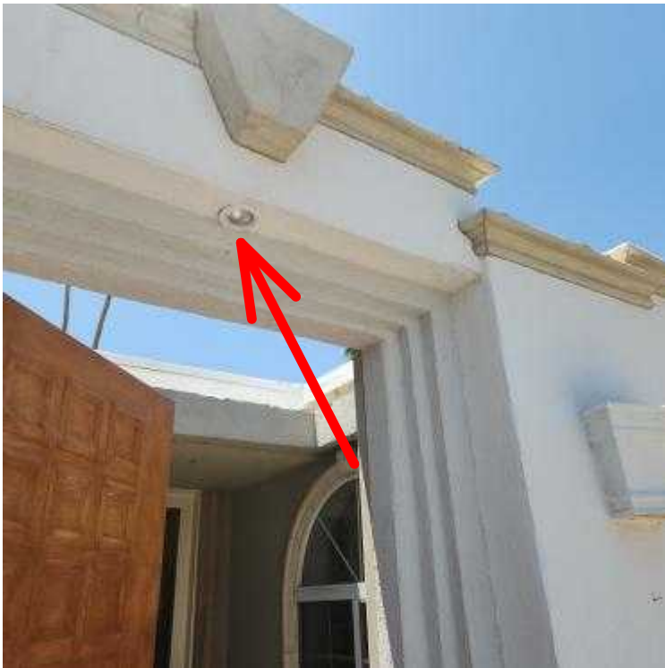
Inoperative fixture/bulb on portico
