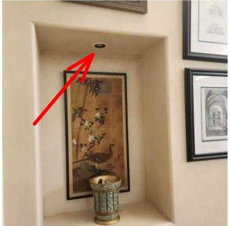
Inoperative fixture/bulb on east wall niche in living room
