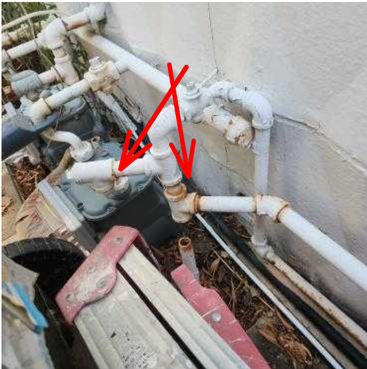
Rusted pipes on/from gas meter
