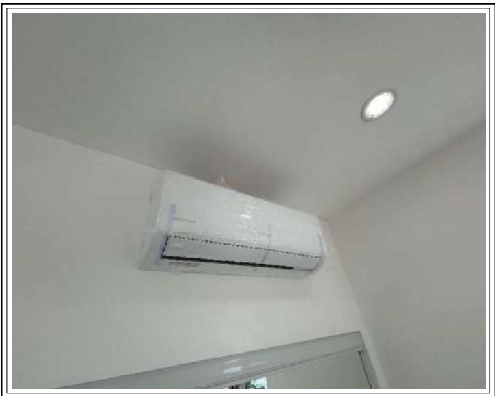
Combo Split AC Unit Unit 4132
