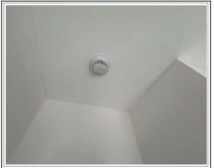
Smoke Alarm Unit 4132
