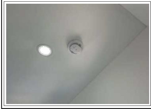
Smoke Alarm Unit 4130
