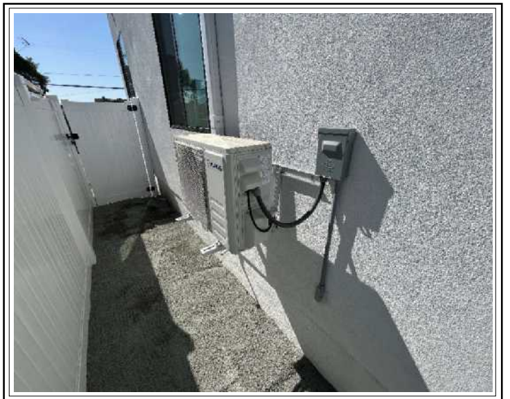
Combo Split AC Unit Unit 4132
