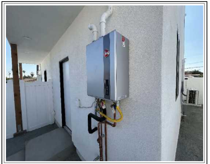
Tankless Water Heater Unit 4130
