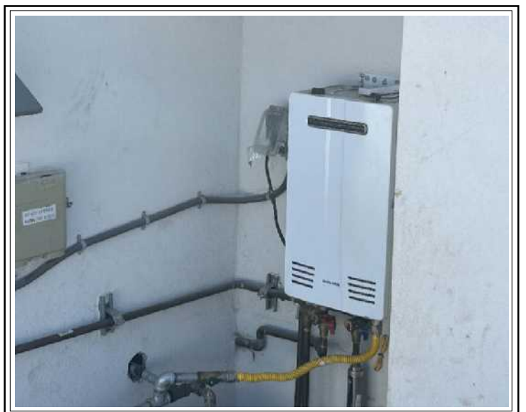
Tankless Water Heater Unit 4128
