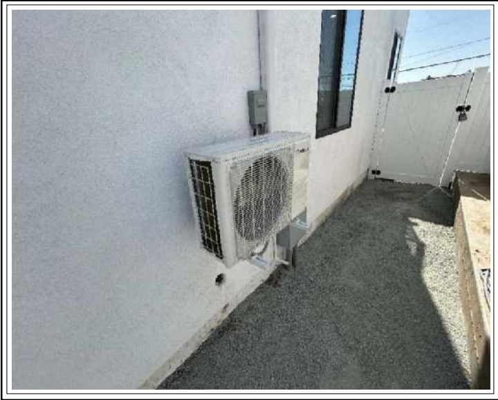
Combo Split AC Unit Unit 4130
