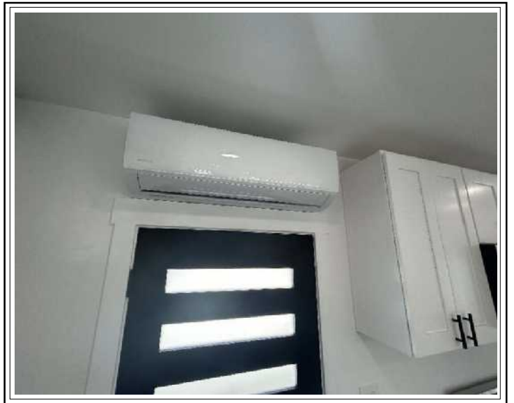
Combo Split AC Unit Unit 4128
