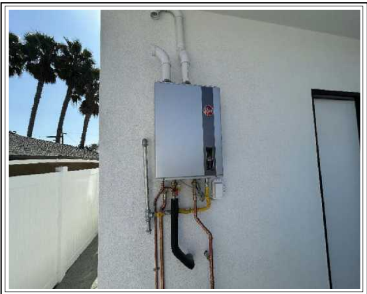
Tankless Water Heater Unit 4132
