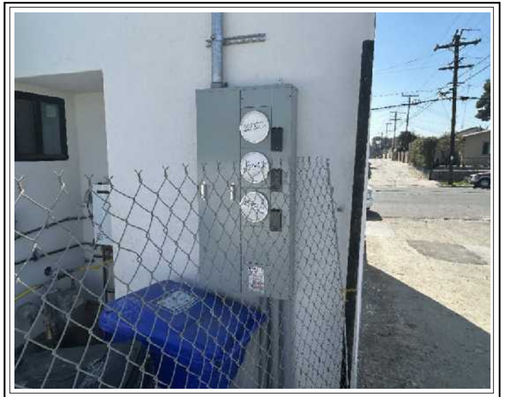
Electric Panel Meter Unit 4128
