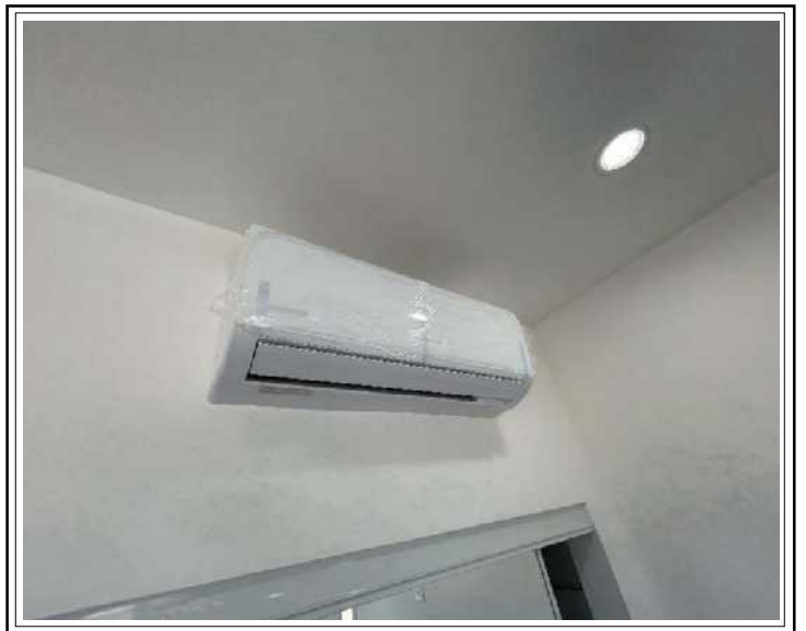
Combo Split AC Unit Unit 4132
