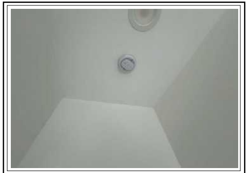
Smoke Alarm Unit 4130
