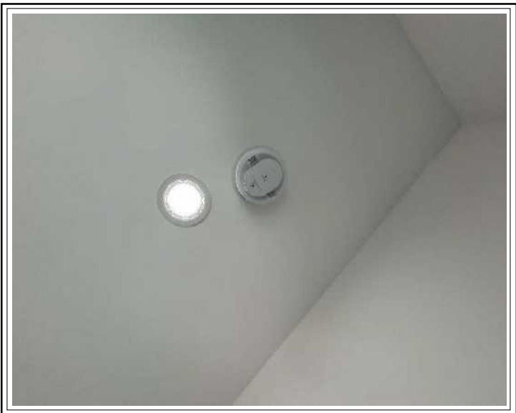
Smoke Alarm Unit 4132
