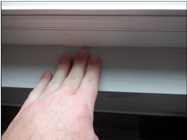
4.4 Item 1(Picture) Primary bedroom window not sealed
