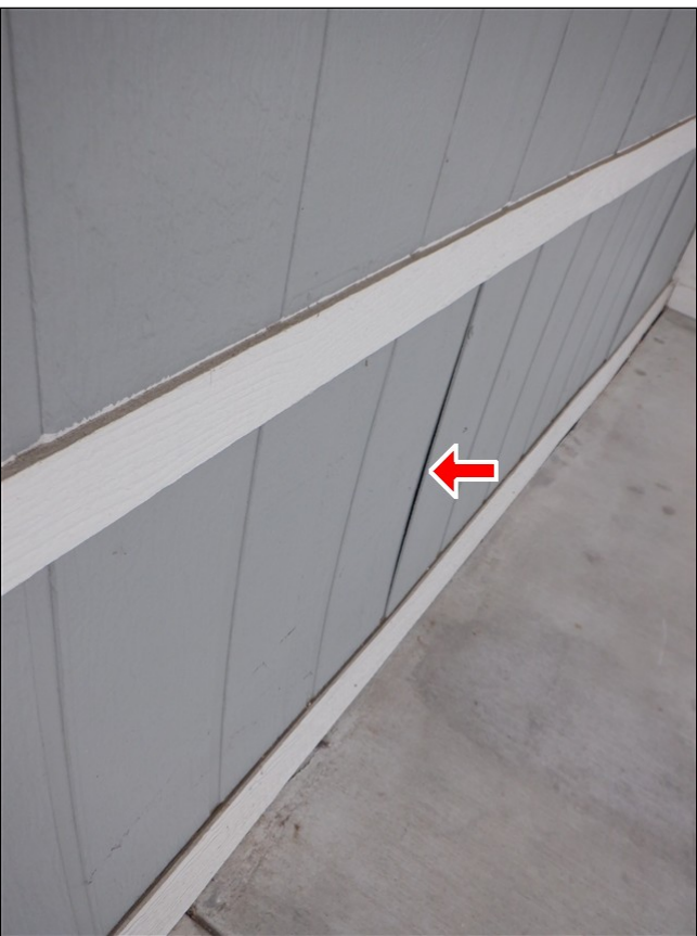
2.0 Item 2(Picture) Gap in skirting
