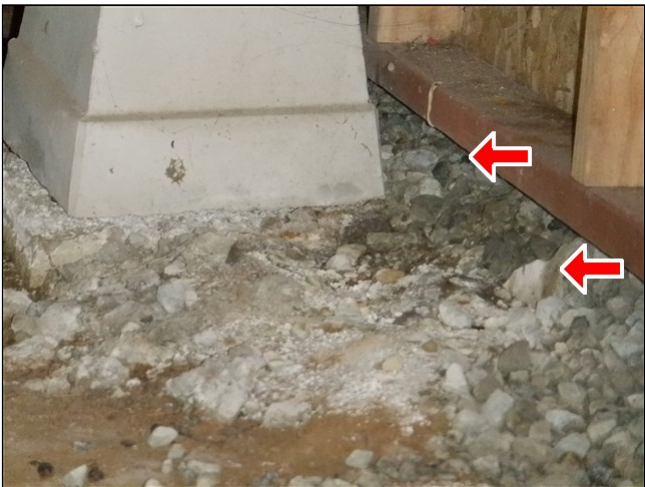
6.0 Item 4(Picture) Moisture under deck
