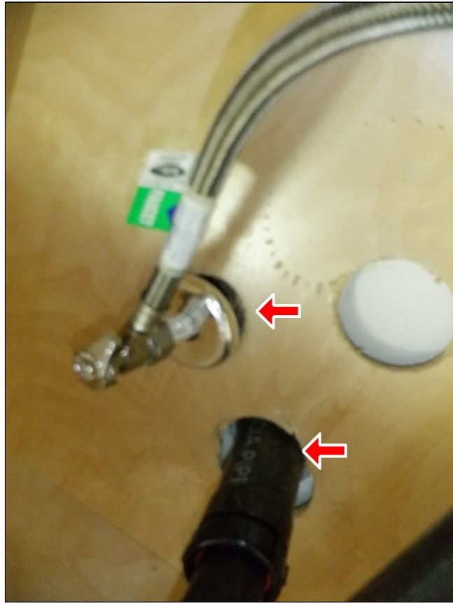
5.6 Item 4(Picture) Plumbing not sealed under sinks
