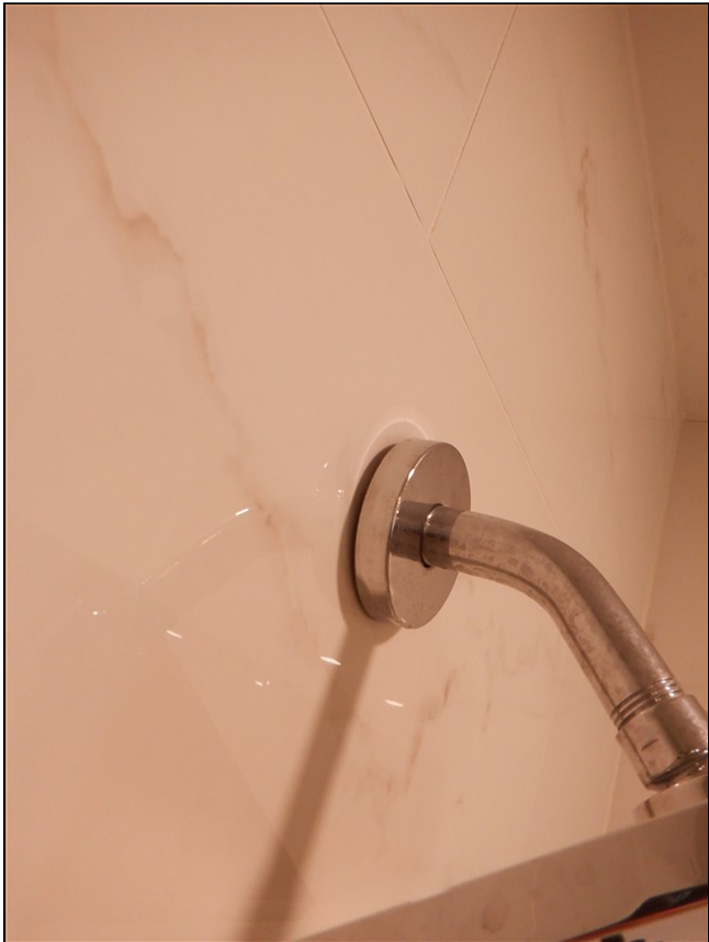
5.7 Item 3(Picture) Primary bath showerhead not sealed
