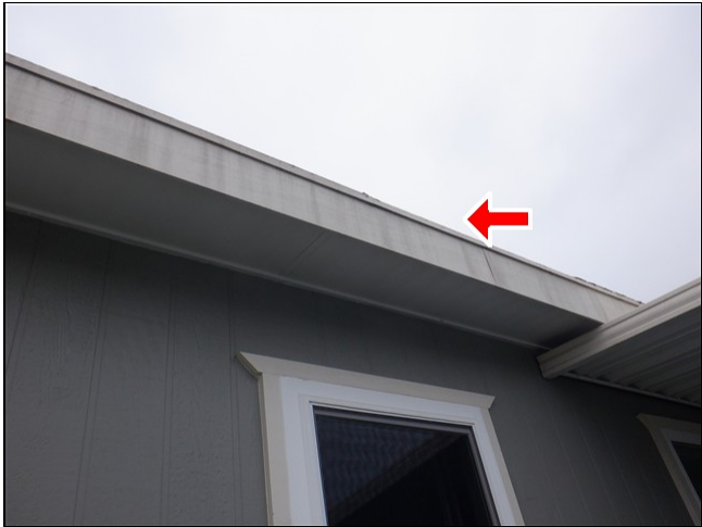
1.2 Item 1(Picture) Missing gutters
