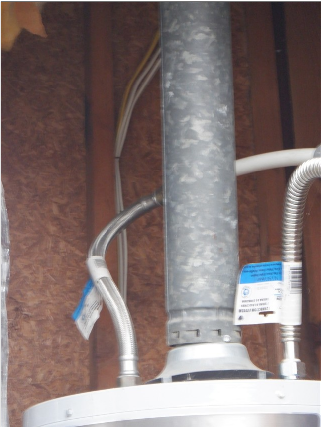
7.1 Item 6(Picture) Flue venting and water lines
