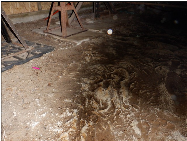
6.0 Item 3(Picture) Moisture under home
