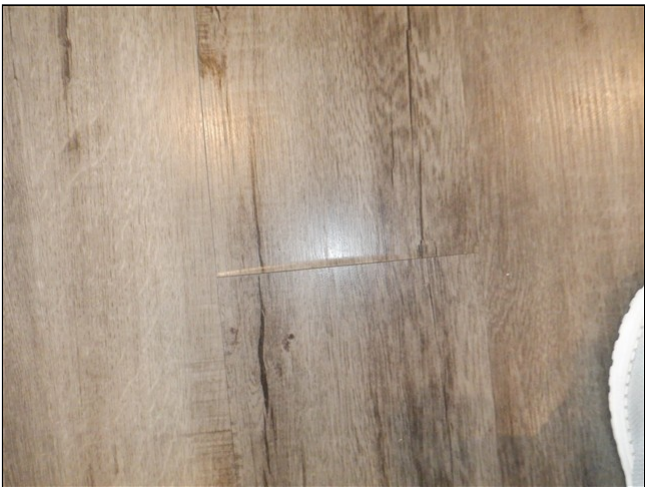
4.2 Item 6(Picture) Damage to floor by kitchen island
