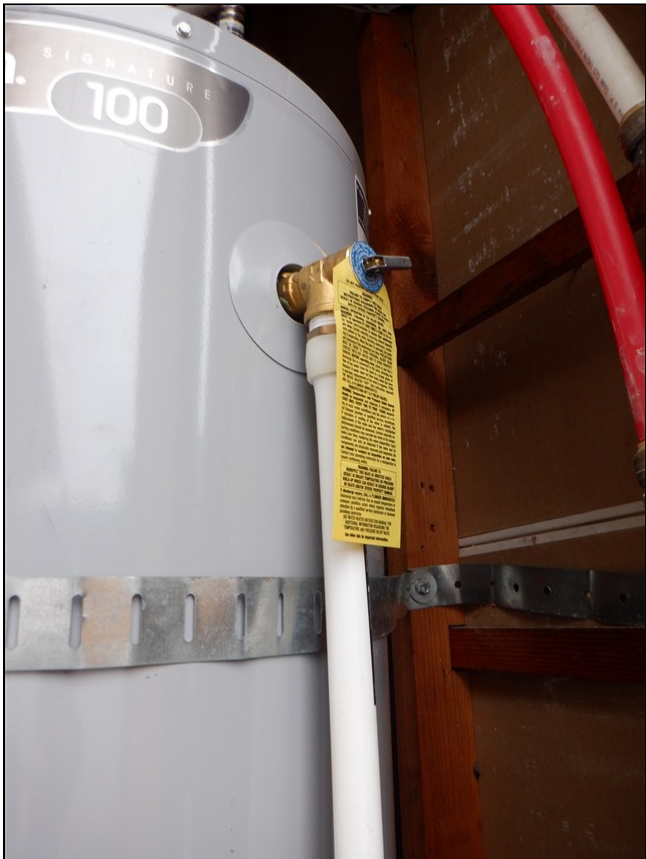
7.1 Item 5(Picture) T&P plumbing
