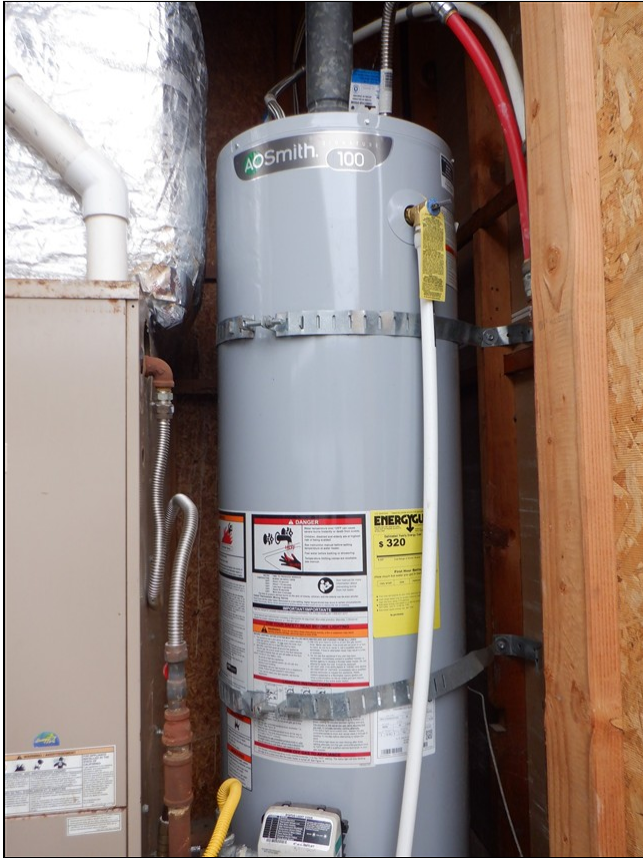
7.1 Item 1(Picture) Water heater
