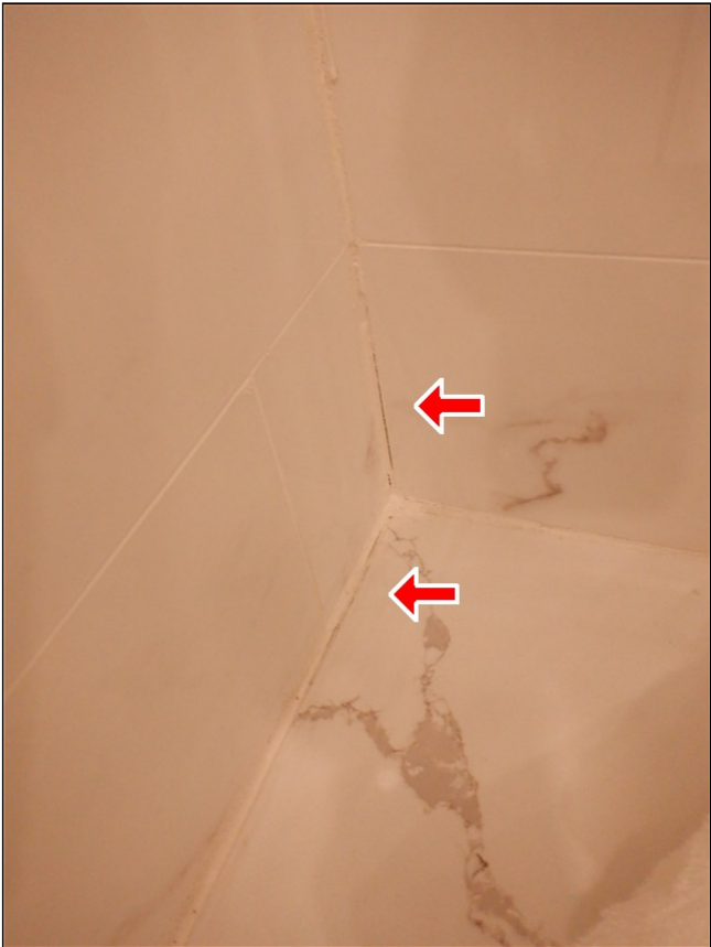
5.7 Item 4(Picture) Primary bath shower caulking cracking and peeling
