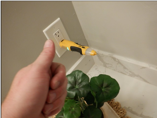
5.8 Item 1(Picture) Good GFCI in bathrooms
