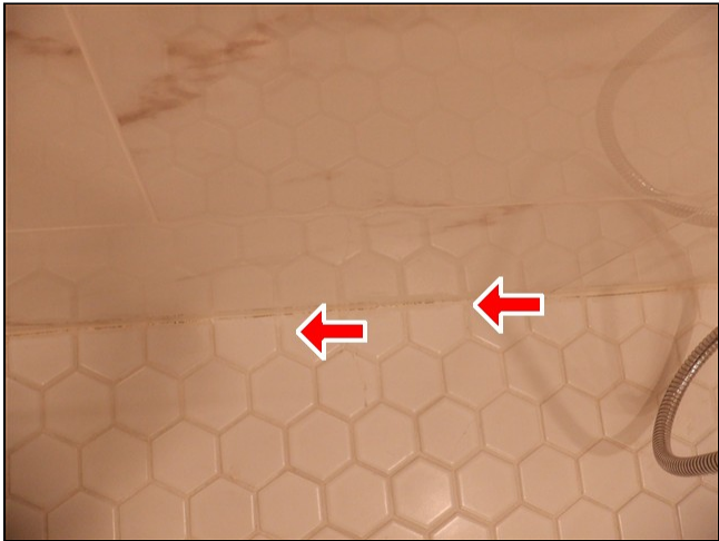
5.7 Item 5(Picture) Primary bath shower not sealed properly
