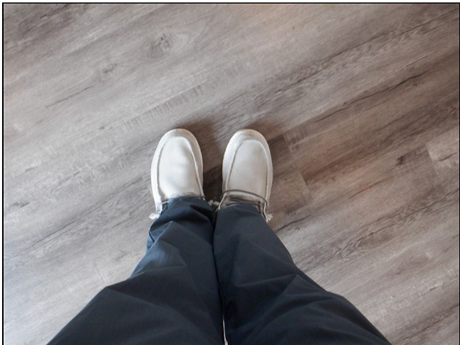
4.2 Item 9(Picture) Soft spots in living room
