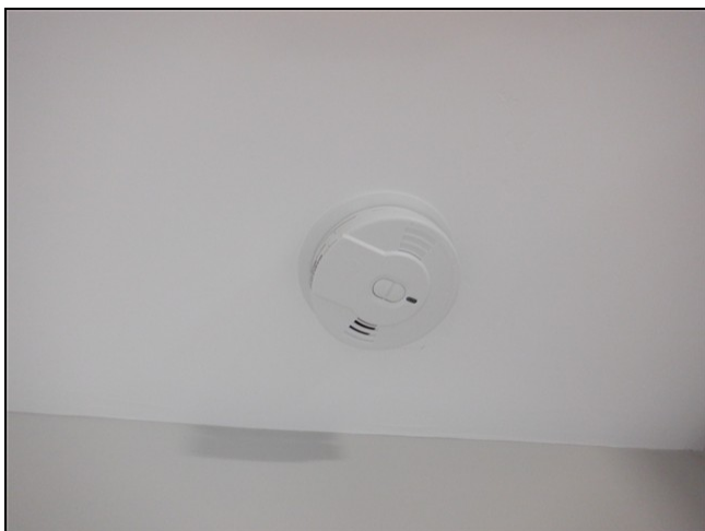
8.5 Item 1(Picture) Smoke detectors
