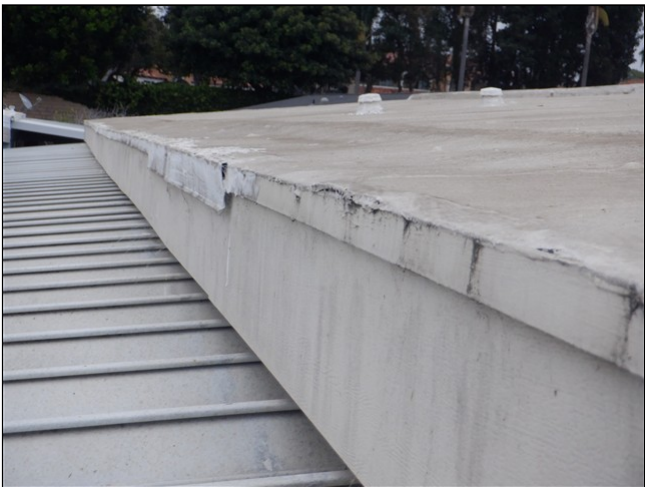
1.0 Item 10(Picture) Roof covering / edges need to be re-sealed
