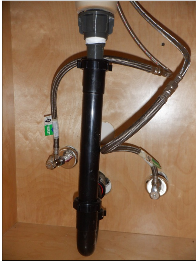
5.6 Item 2(Picture) Primary bath sink plumbing / no leaks
