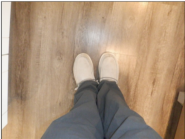
3.2 Item 1(Picture) Soft sub floor in kitchen
