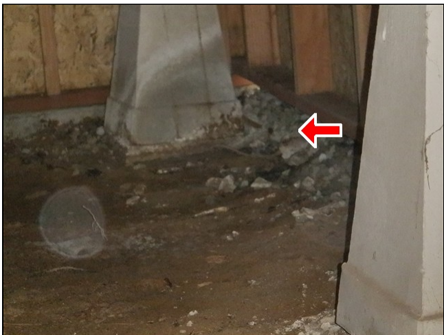
6.0 Item 5(Picture) Moisture under deck
