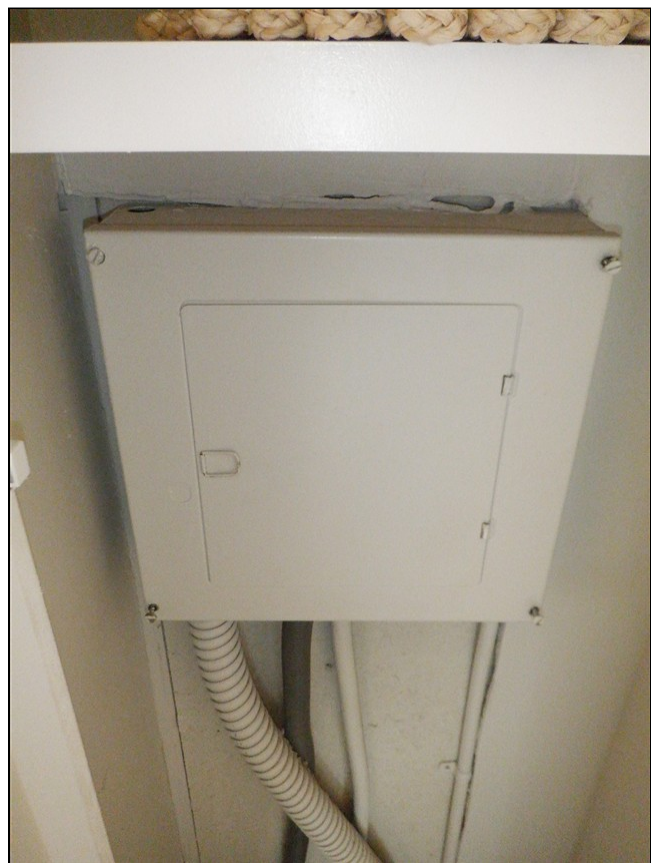
8.0 Item 1(Picture) Electrical panel
