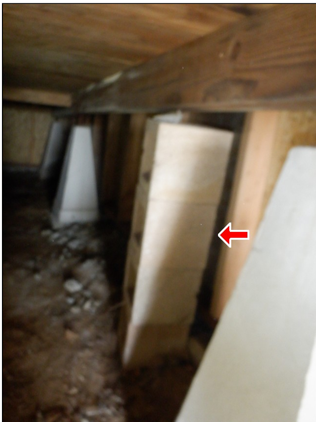
6.2 Item 7(Picture) Improper concrete pier under deck
