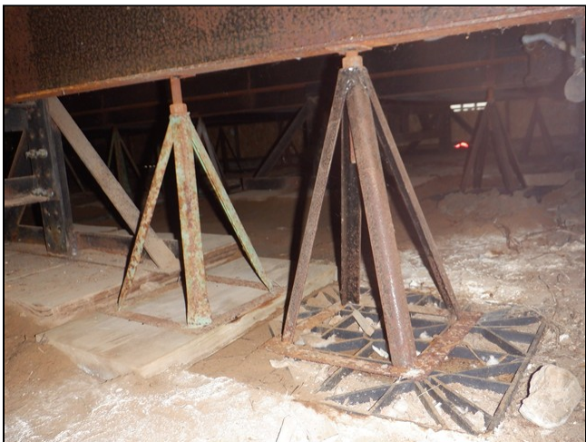
6.2 Item 1(Picture) Steel jacks
