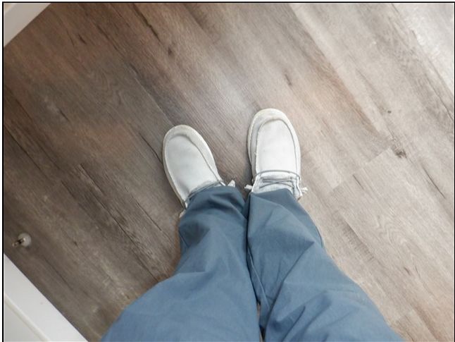
4.2 Item 7(Picture) Soft spot in laundry room
