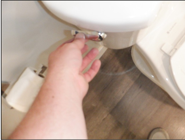
5.7 Item 7(Picture) Loose primary bath toilet handle
