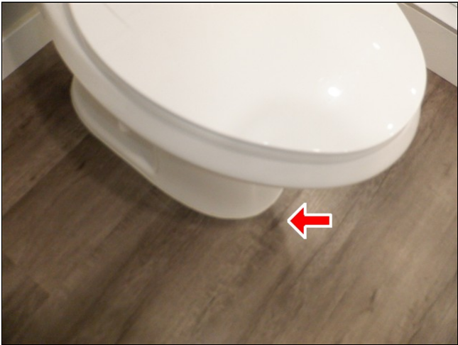
5.7 Item 6(Picture) Loose primary bath toilet
