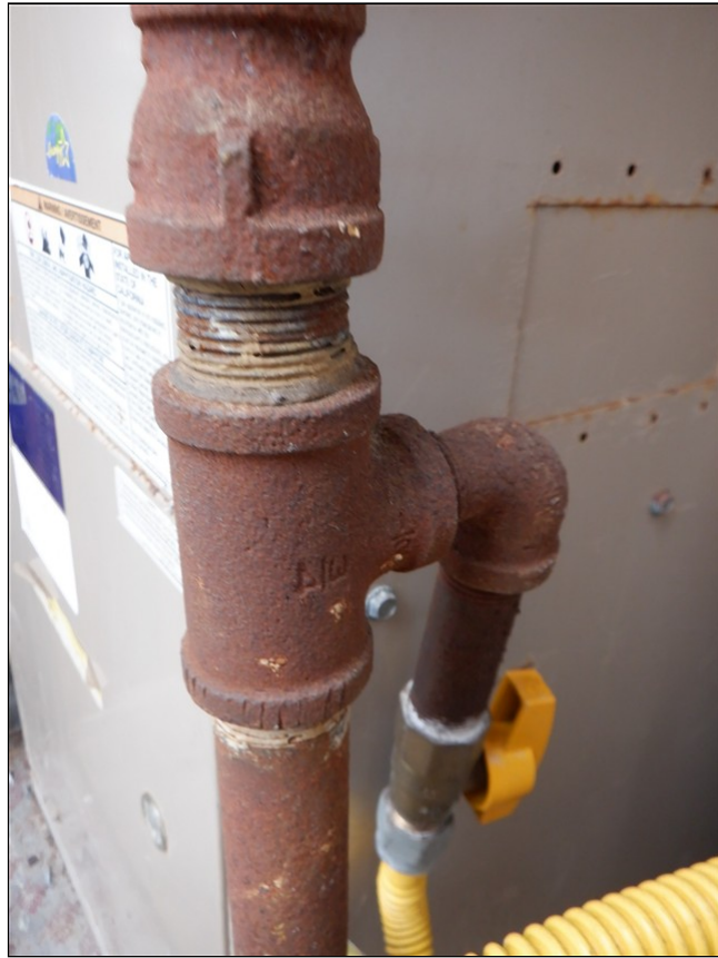
9.0 Item 2(Picture) Missing sediment trap
