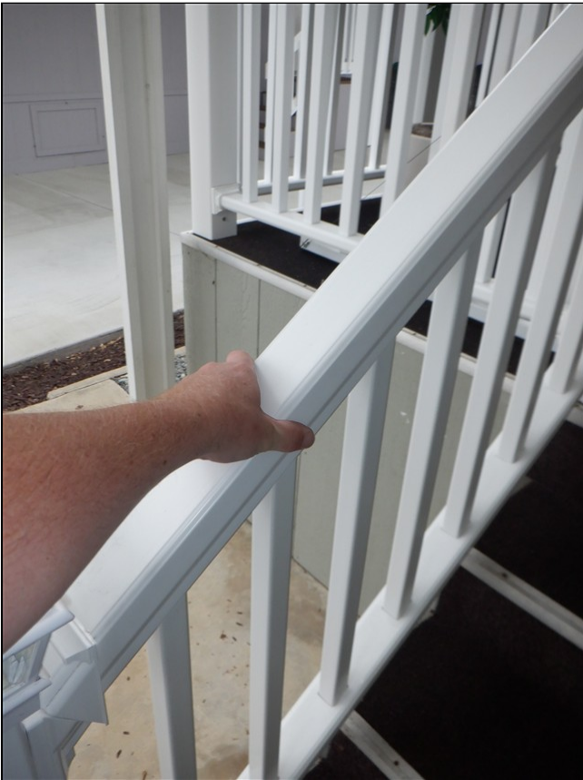
2.3 Item 1(Picture) Loose railing
