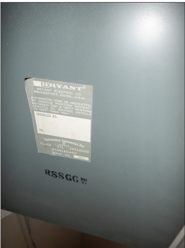
8.0 Item 2(Picture) Bryant panel
