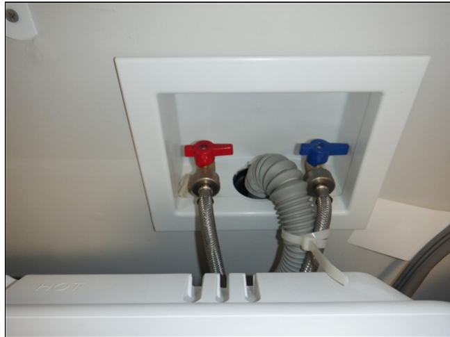
3.13 Item 4(Picture) Washer valves / drain
