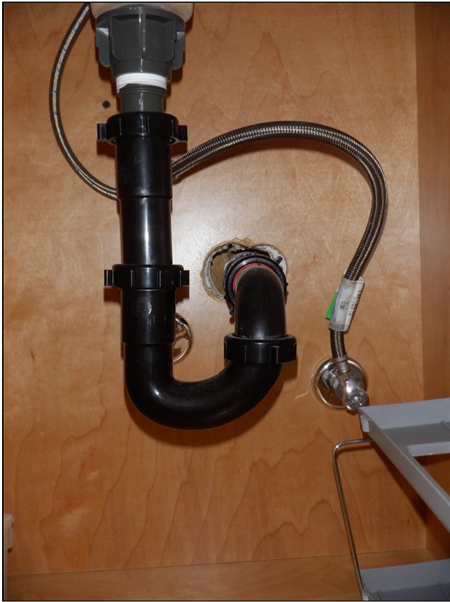
5.6 Item 3(Picture) Primary bath sink plumbing / no leaks
