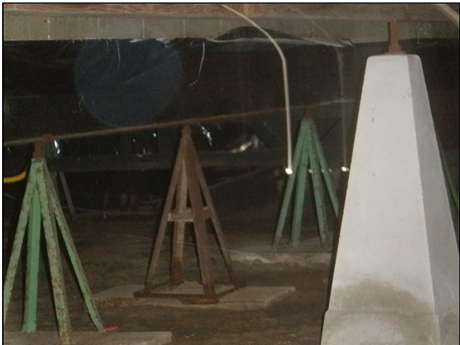
6.2 Item 5(Picture) Steel jacks
