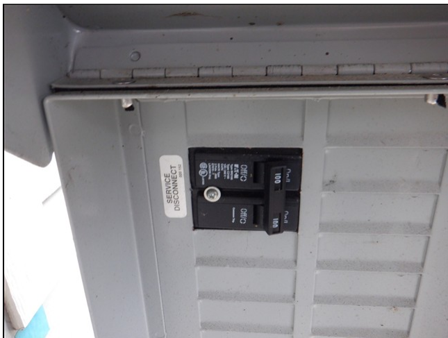
8.4 Item 1(Picture) Main 100 amp breaker
