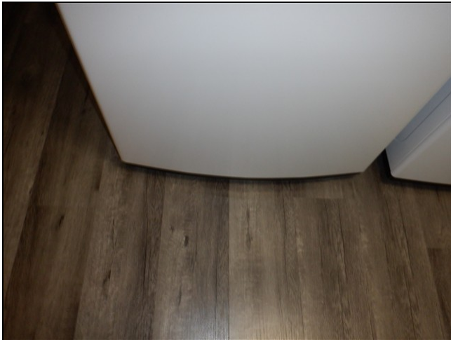
3.13 Item 3(Picture) Missing drip pan
