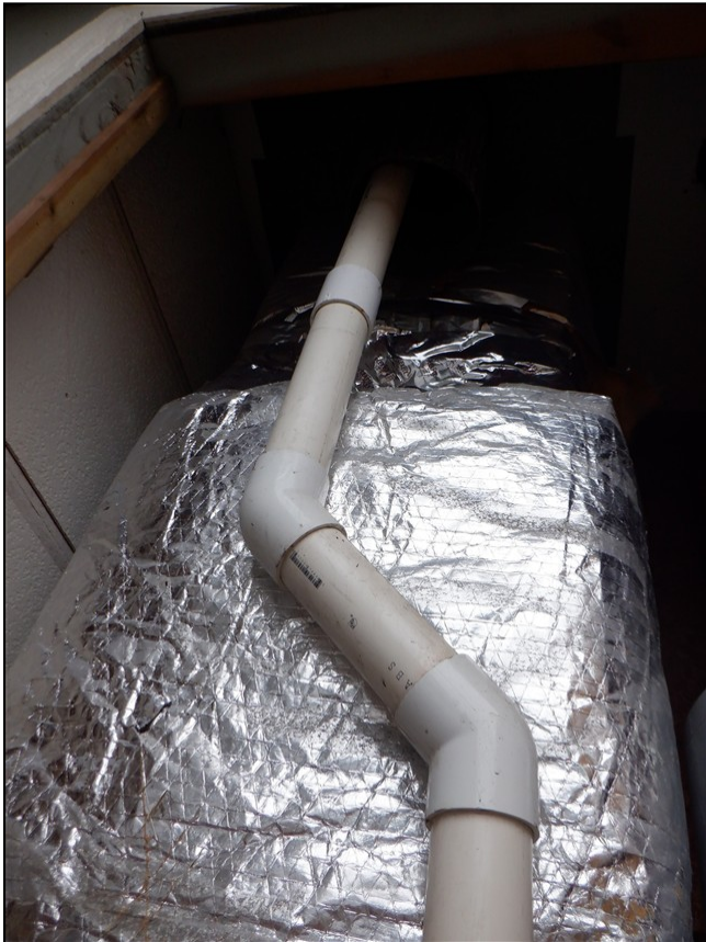
9.0 Item 3(Picture) Flue venting
