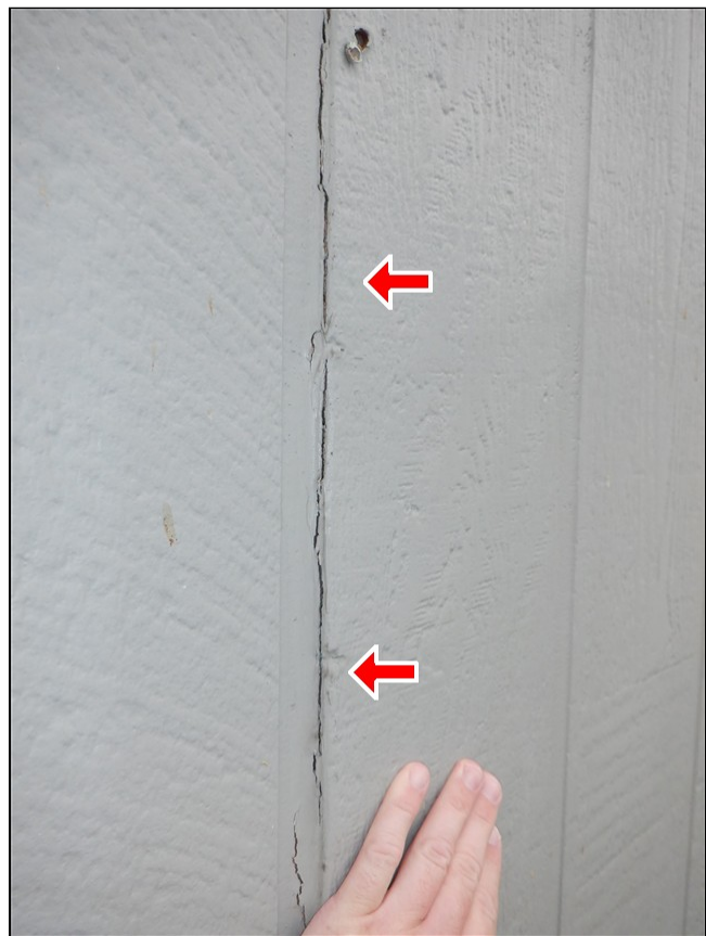
2.0 Item 1(Picture) Siding not sealed at back of home
