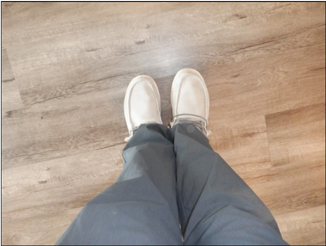
4.2 Item 2(Picture) Soft sub floor
