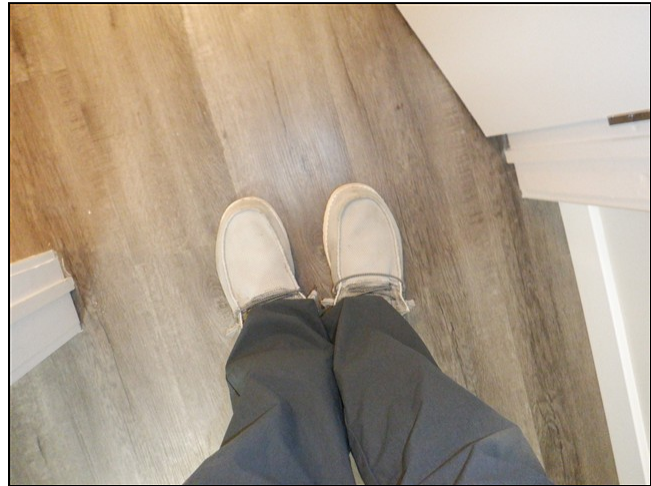
4.2 Item 1(Picture) Soft spots in sub floor
