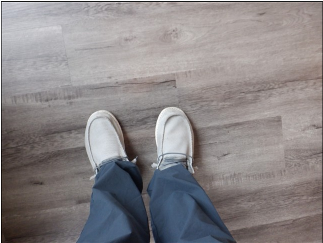
4.2 Item 8(Picture) Soft spots in living room
