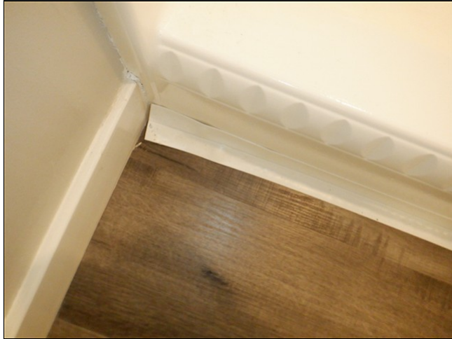
5.7 Item 2(Picture) Base of hallway bath shower not properly sealed
