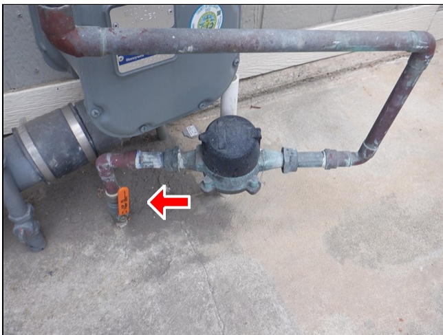
7.2 Item 1(Picture) Main water shut off
