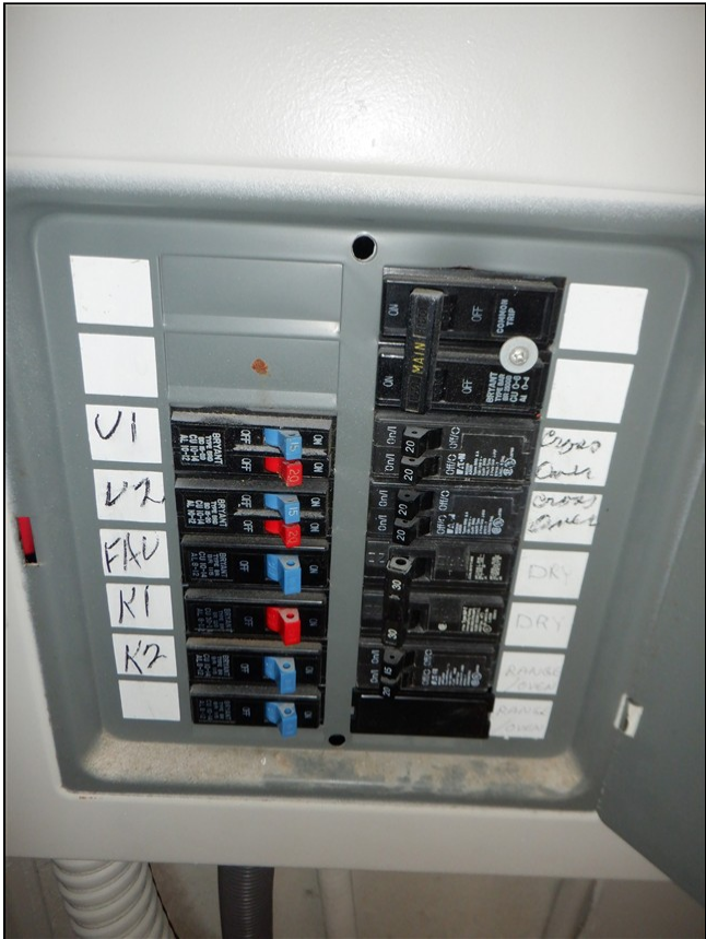
8.0 Item 3(Picture) Circuit breakers
