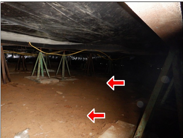
6.0 Item 6(Picture) Moist under home / no vapor barrier
