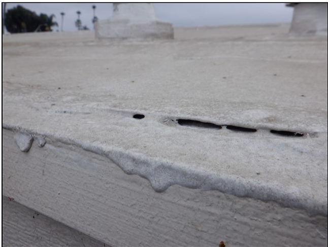
1.0 Item 9(Picture) Roof covering / edges need to be re-sealed
