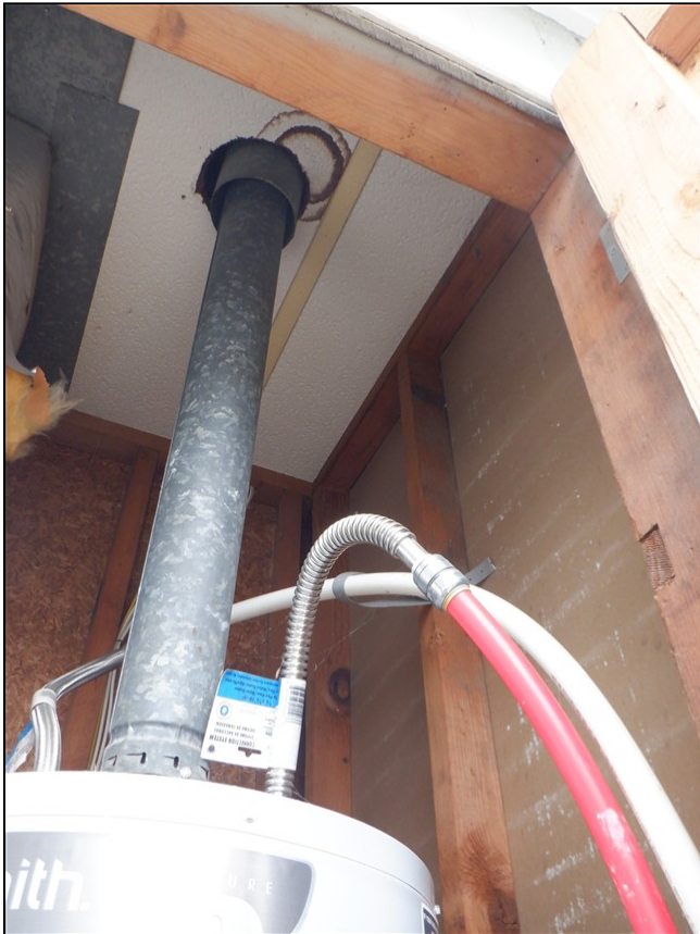
7.1 Item 7(Picture) Missing expansion tank
