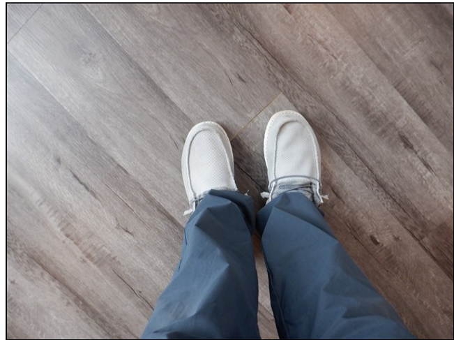
4.2 Item 3(Picture) Soft sub floor
