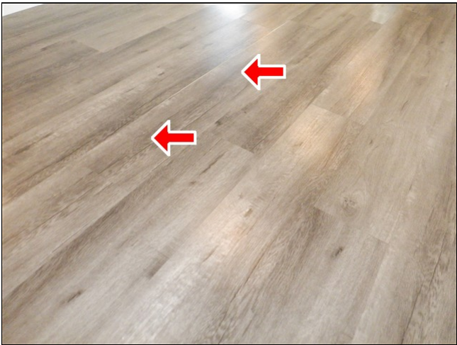
4.2 Item 4(Picture) Damage to flooring
