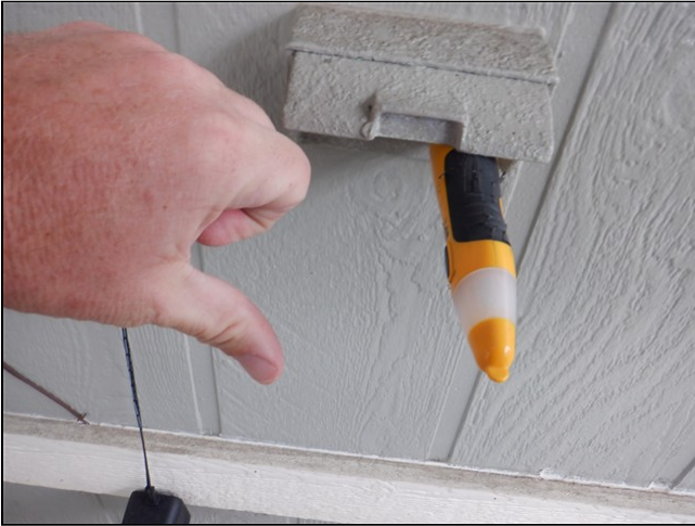
2.7 Item 1(Picture) Not GFCI protected
