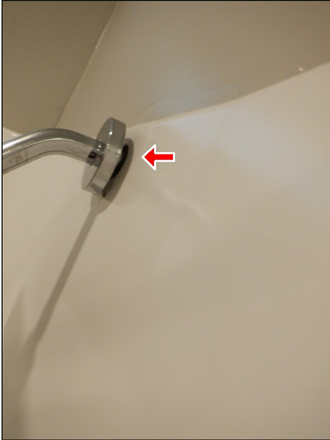
5.7 Item 1(Picture) Showerheads not sealed
