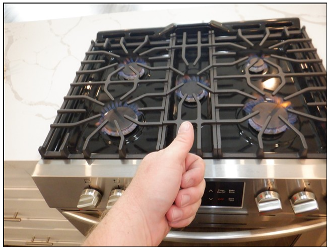
3.9 Item 1(Picture) Cook top burners
