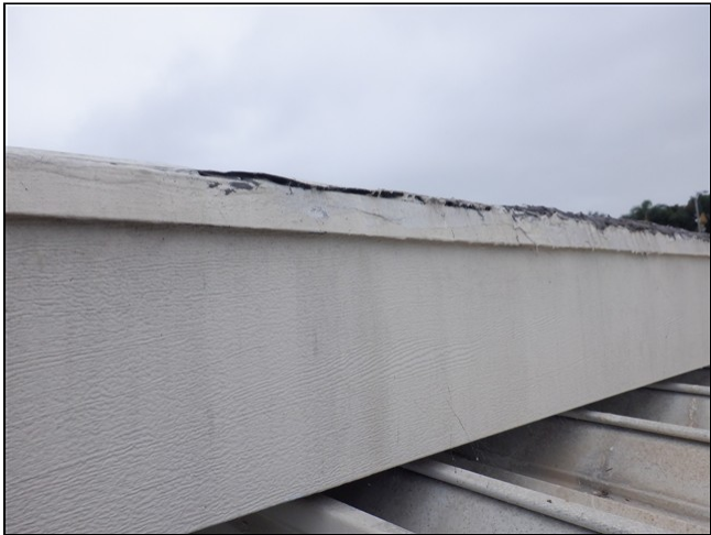
1.0 Item 11(Picture) Roof covering / edges need to be re-sealed
