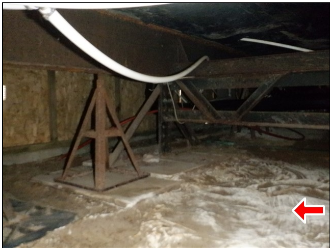
6.0 Item 1(Picture) Moisture under home
