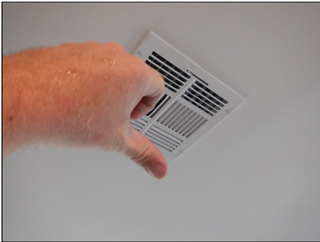
9.0 Item 5(Picture) No air flow from vents
