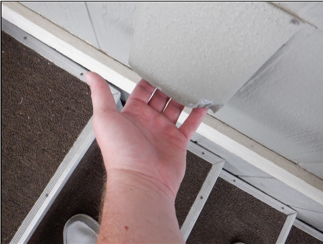
3.13 Item 1(Picture) Missing screen on dryer vent
