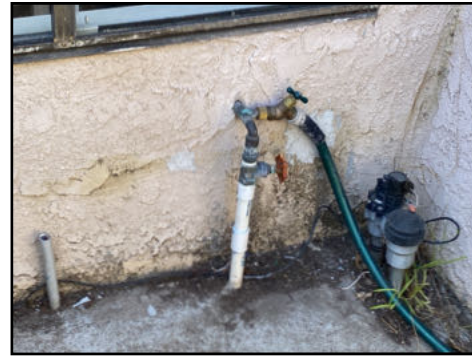
Blistered due to exterior plumbing - recommend adjusting away from structure areas
