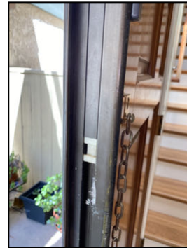
Did not operate/properly - needs to be serviced
