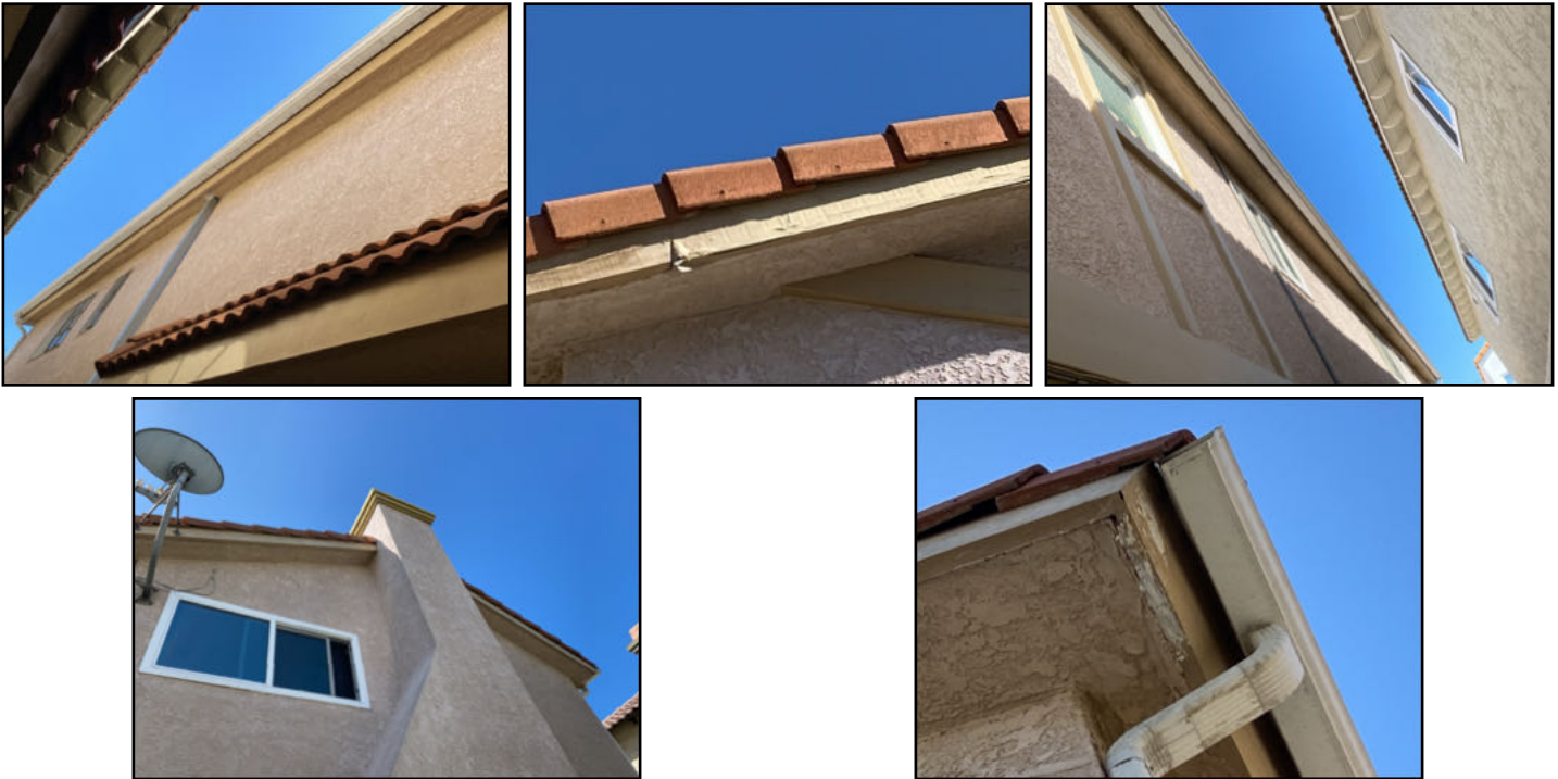
Deteriorated wood at corner joints of fascia - needs to be serviced
