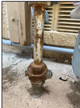
Minor rusting - typical for exterior weathering - recommend rust treatment
