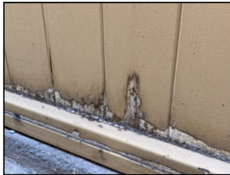
Wood deterioration - needs to be serviced
