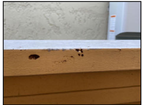
Wood deterioration - needs to be serviced
