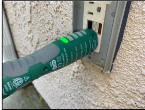
Test did not operate- needs to be serviced
