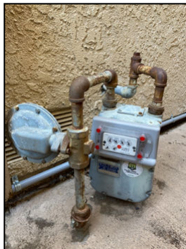
Significant rusting - needs to be serviced
