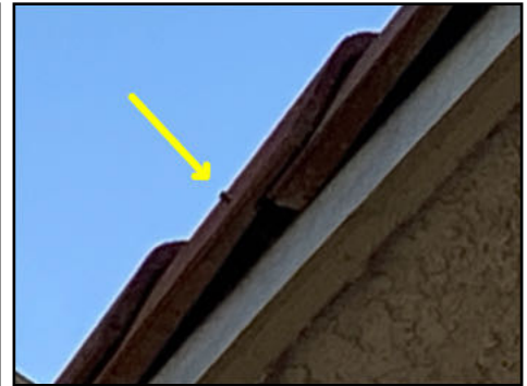
Loose/slipping tiles/shingles - needs to be serviced
