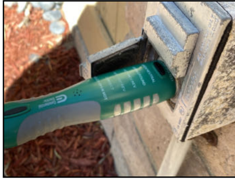
Non- energized (dead) outlet(s) - needs to be serviced
