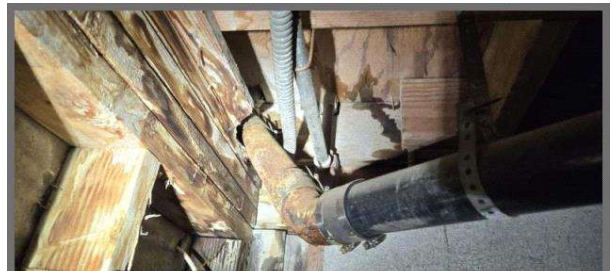
BLISTERS AND LEAK
