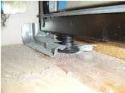
Example of an installed device
