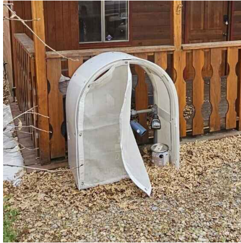
Gas Meter Cover
