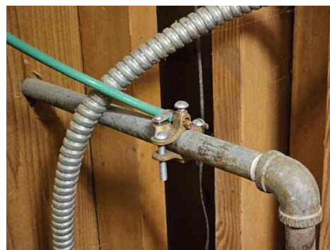
Gas Piping Bonding
