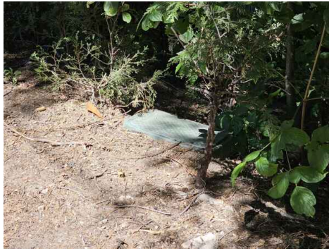
Water Meter Box
