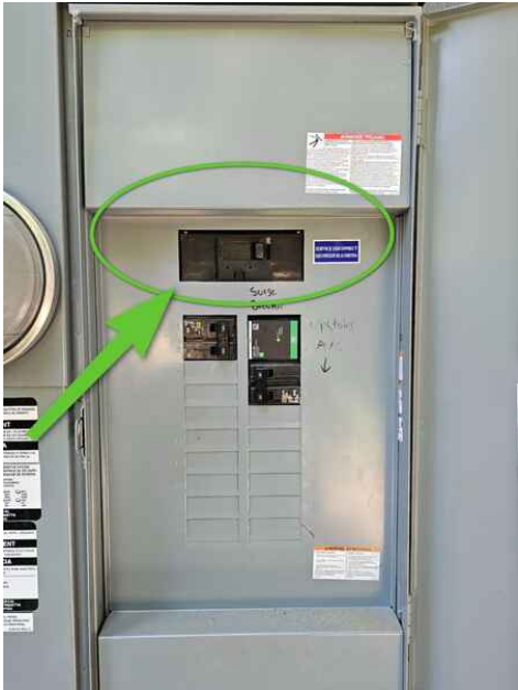
Main Panel & Main Breaker
