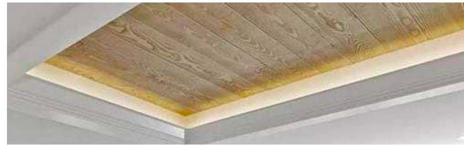
TRAY CEILING LIKE IMAGE COVERED WITH WALLPAPER OR WOOD PLANKS COVE LIGHTING
