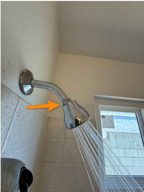
Hall Bathroom Shower, Appeared to be leaking from here
