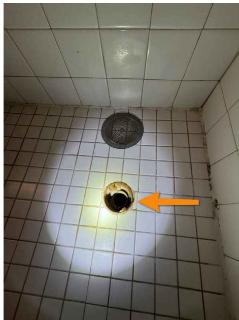
Example noted at Primary Bathroom Shower drain
