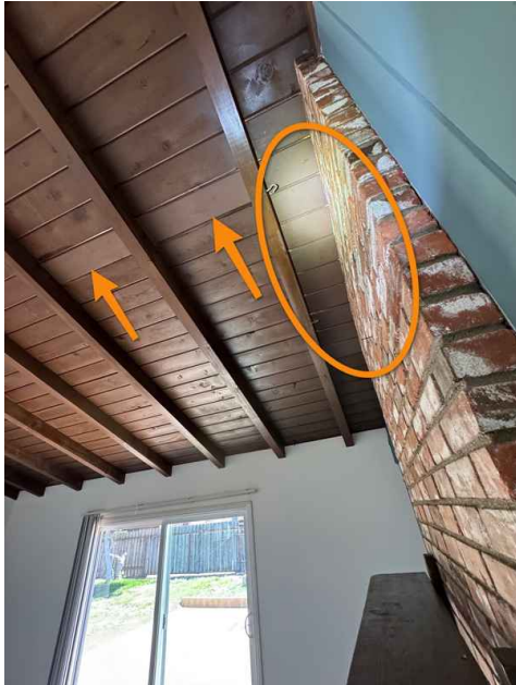
Example of Possible Repairs noted at Living Room
