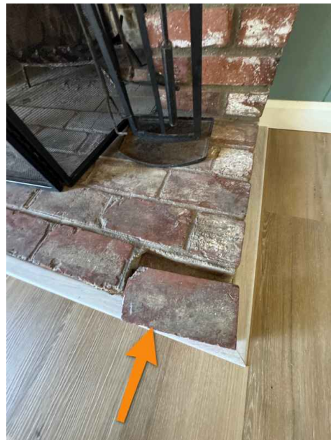
Example of loose brick noted at Fireplace
