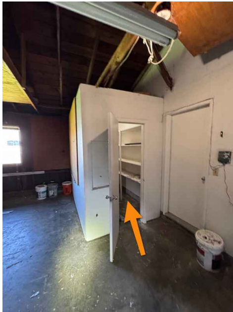
Example noted at Garage Rear
