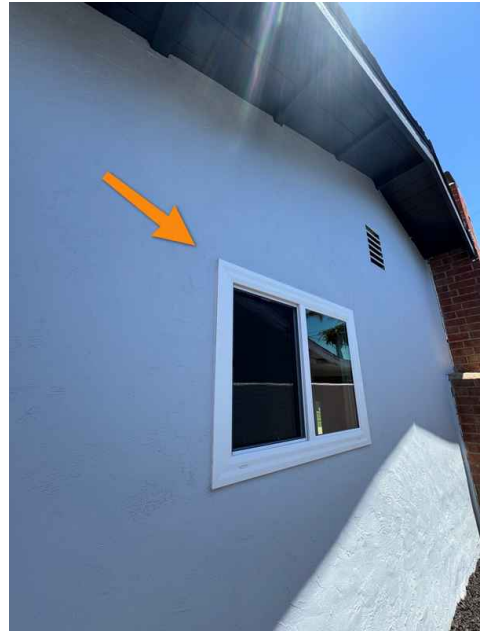
Example noted at Right Side of Home
