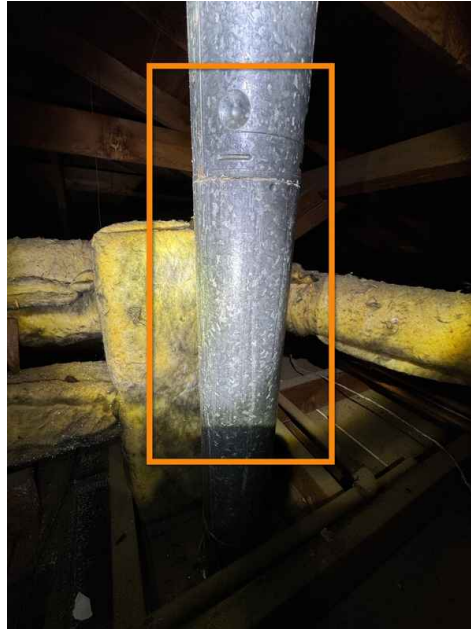
Example of moisture staining noted at flue in Attic
