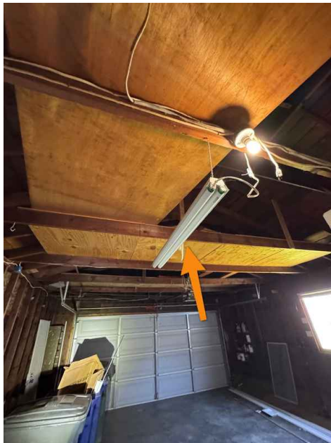
Example noted at Garage
