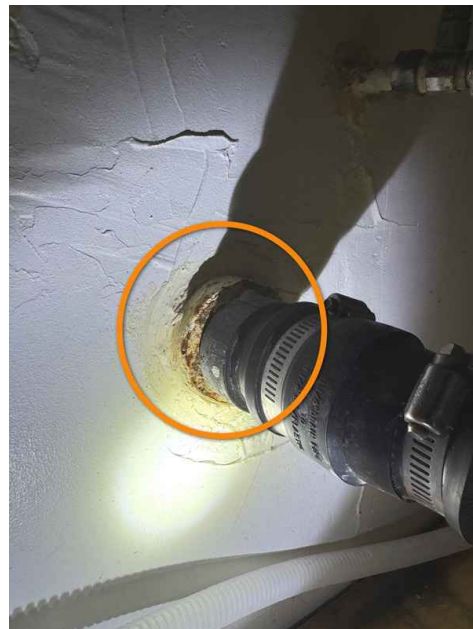
Example of rust noted
