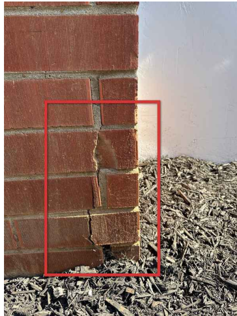
Example of damage noted, Rear Right Side of Home
