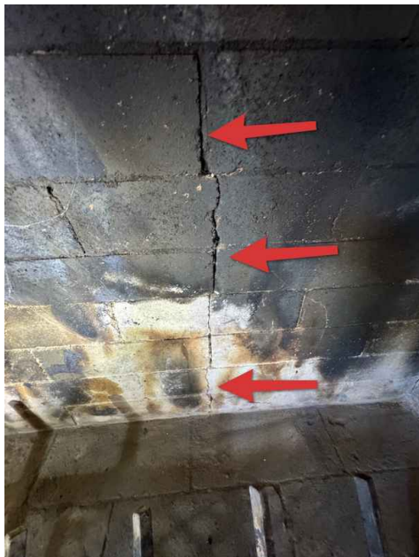
Example of cracking noted
