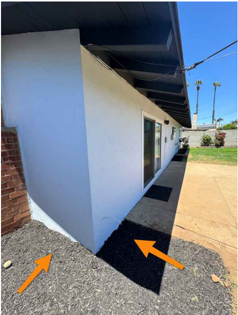
Example noted at Rear, Right Side of Home
