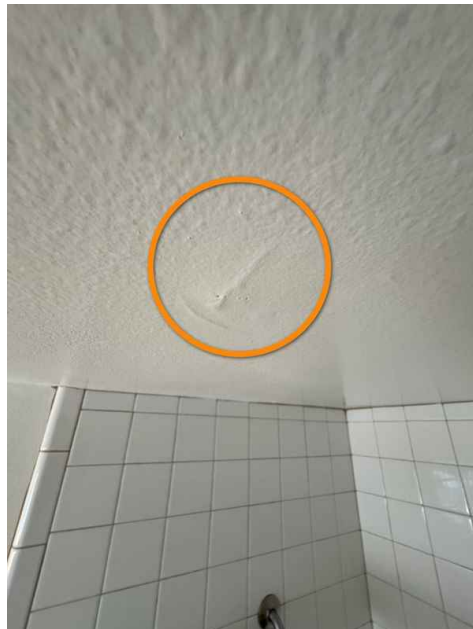
Example of moisture damage noted
