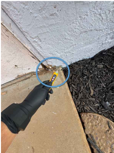
Wires did not appear powered
