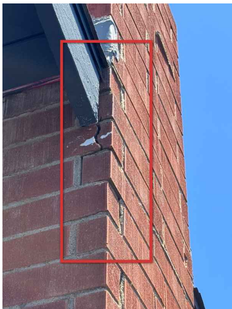
Example of cracking noted, Right Side of Home
