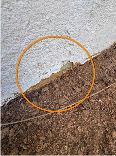
Example of moisture damage noted
