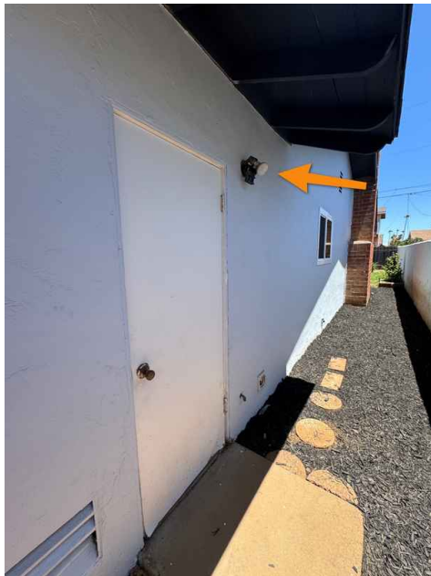
Example noted at Right Side of Home
