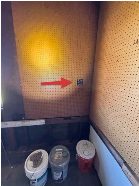
Example noted at Garage
