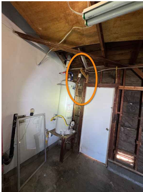
Example noted at Garage Rear
