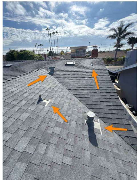
Example of exposed nail heads noted at Roof flashings
