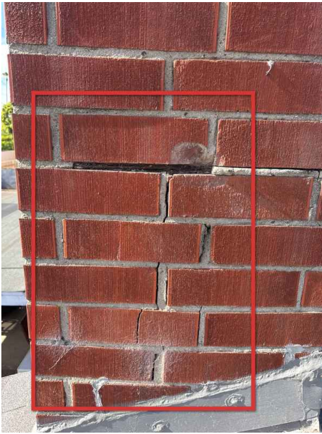
Example of cracking noted
