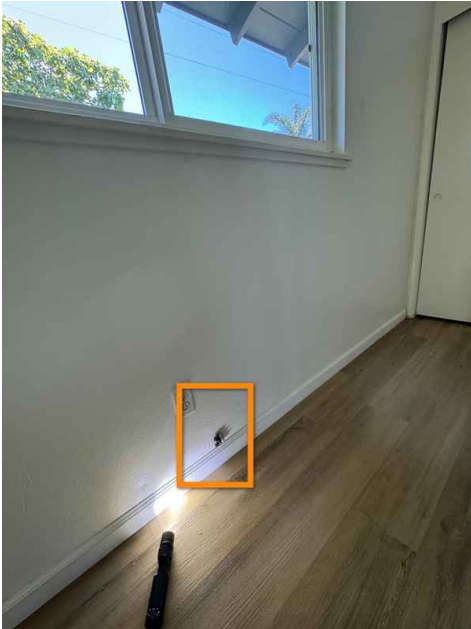
Example noted at Bedroom #2
