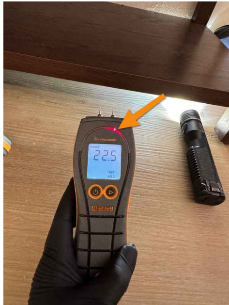
Elevated levels of moisture detected
