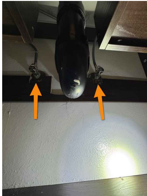
Example noted at Hall Bathroom Sink, loose
