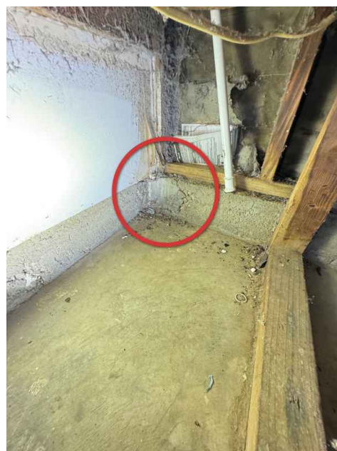
Example noted at Garage, Rear Left Side Below Water Heater
