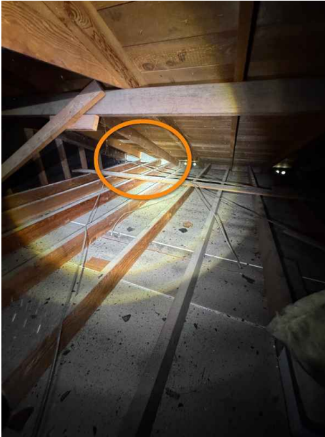
Example noted at Attic, Rear Left Side
