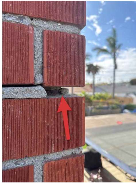
Example of missing mortar noted, Rear Roof
