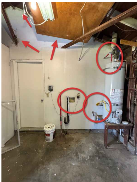
Example noted at Garage Rear
