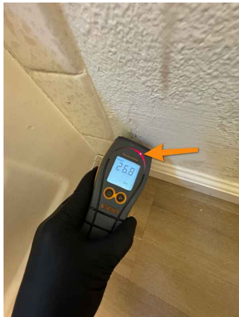
Elevated levels of moisture detected
