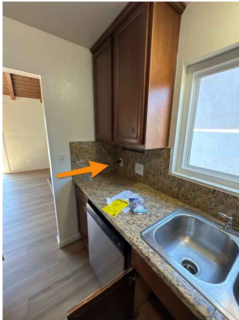
Example noted at Kitchen, loose
