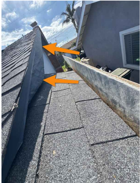
Example of damage and repairs noted, Right Side Roof
