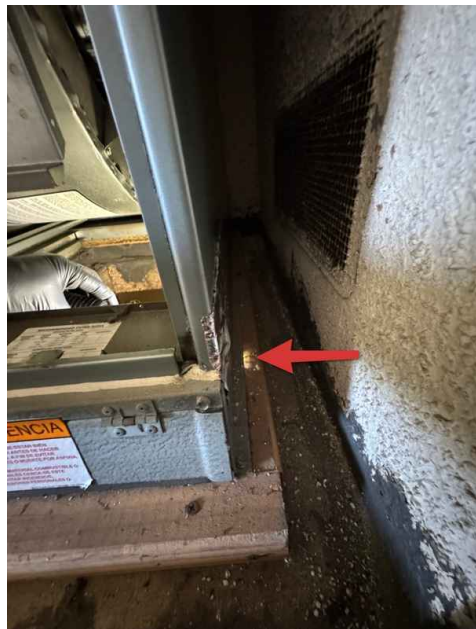
Example of inadequate seal noted
