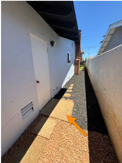
Example of crack noted at Right Side of Home
