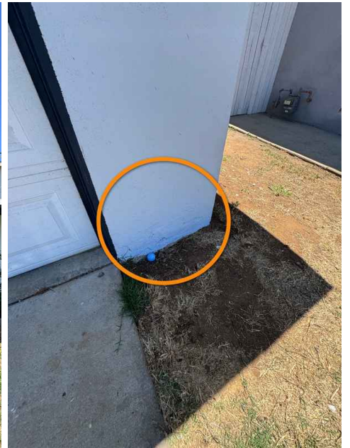
Example of damage noted
