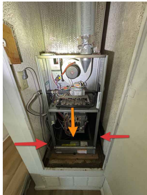
Example noted Below HVAC Unit, Hallway Utility Closet
