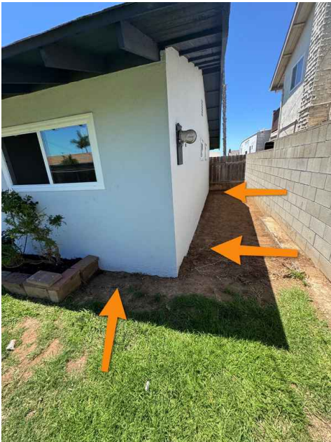
Example noted at Rear, Left Side of Home
