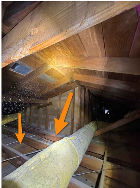
Example noted at Attic, Rear
