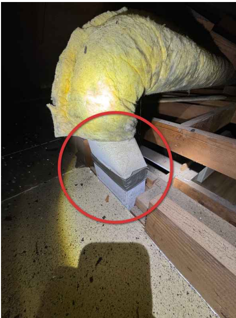
Example noted at Attic
