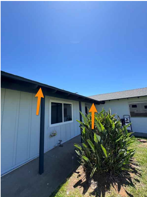
Example noted at Front Roof
