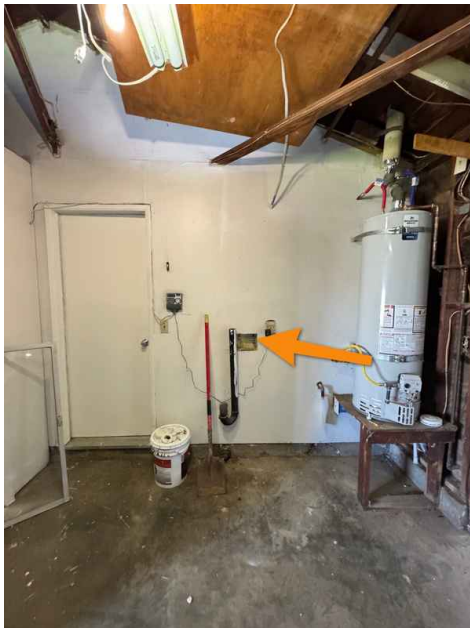
Example noted at Garage Rear, Laundry Area
