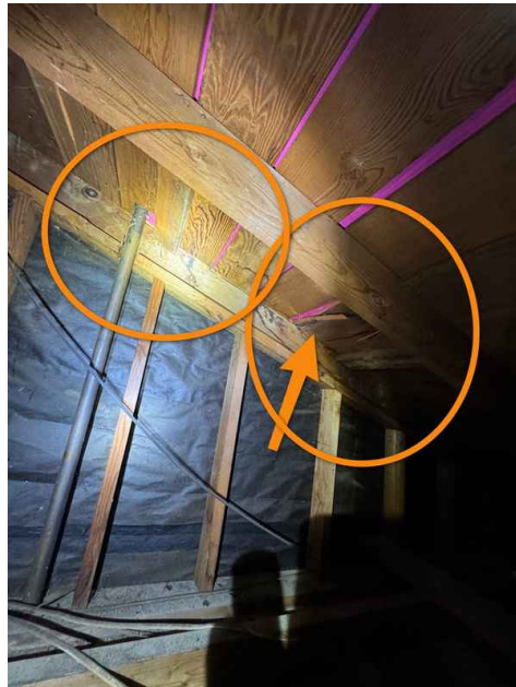
Example of damage, staining noted at Attic
