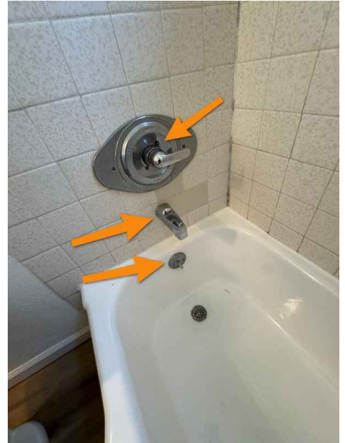
Example noted at Hall Bathroom Shower Bathtub
