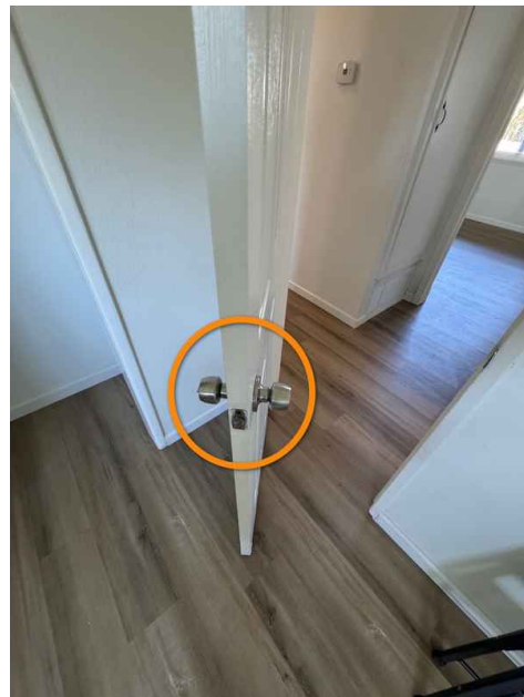
Example noted at Bedroom #2, handle loose, missing stopper
