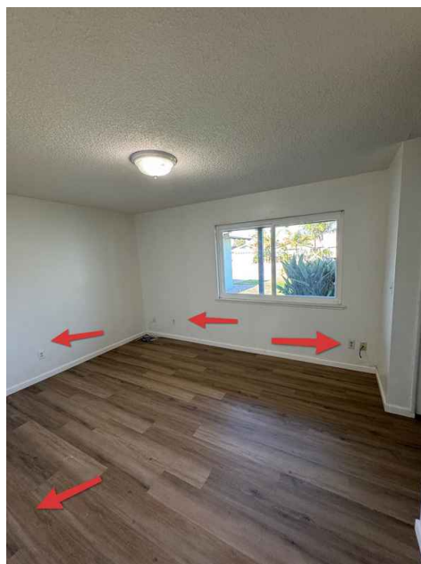
Example noted at Primary Bedroom
