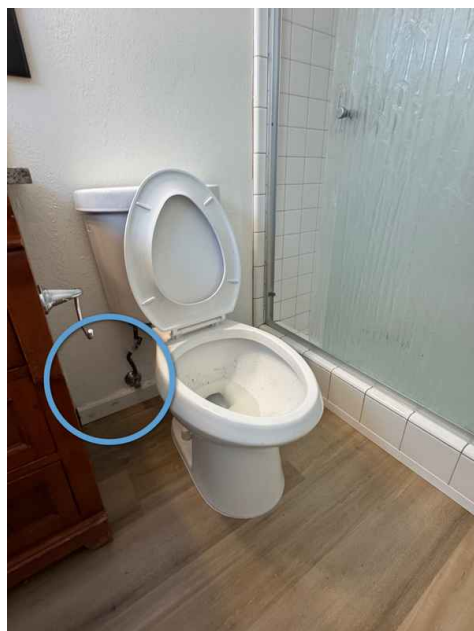
Example noted at Primary Bathroom
