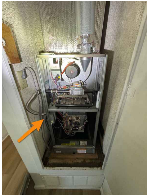
Missing Gas Sediment Trap
