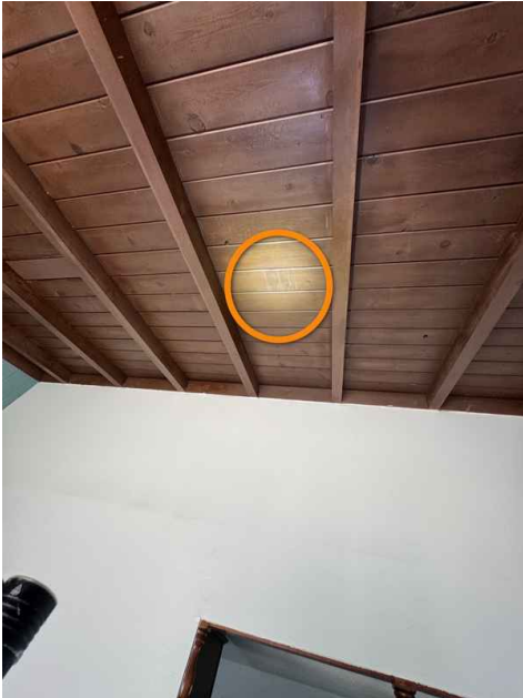
Example of staining noted at Living Room
