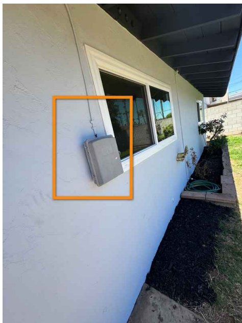
Example noted at Rear of Home
