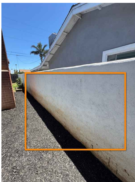
Example noted at Right Side wall, cracking noted, no weep holes visible
