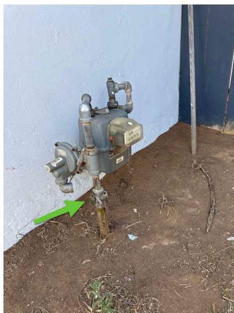
Main Gas Shut-off Valve
