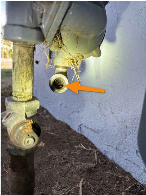
Cap or pipe appeared to be missing
