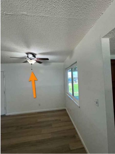
Example noted at Dining Room
