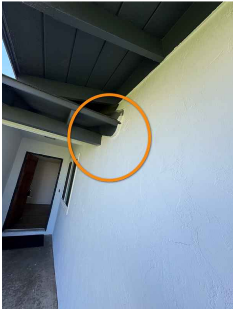
Example of repairs noted at Front
