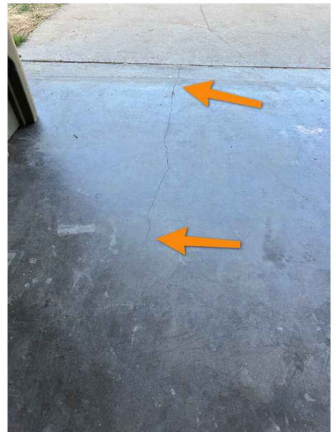
Example of crack noted, Garage, Front Left Side facing outwards
