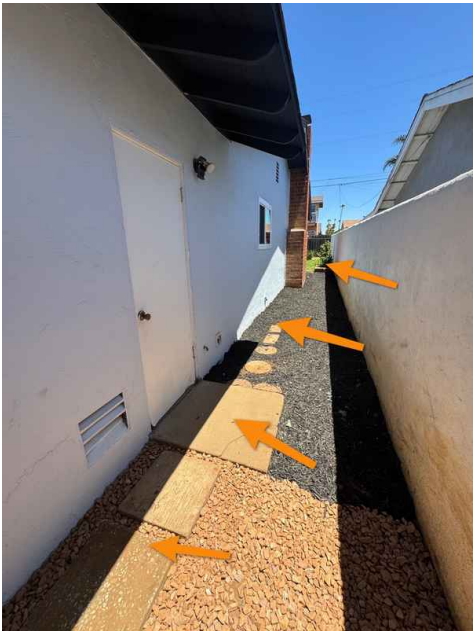
Example of low areas noted at Right Side of Home
