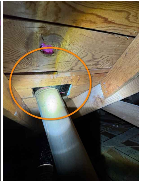
Example of damage noted, Attic
