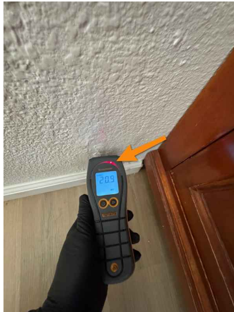
Elevated levels of moisture detected
