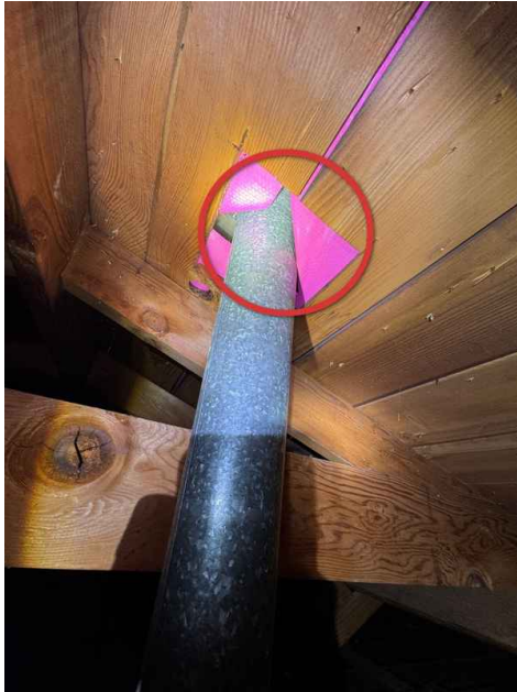
Example noted at Attic, Above HVAC Unit
