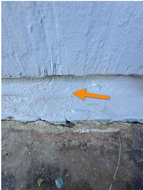
Example of crack noted
