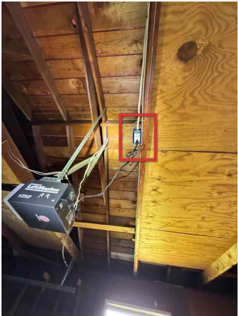
Example noted at Garage, missing faceplate
