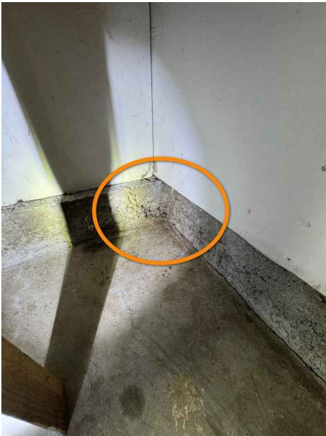
Example of spalling noted
