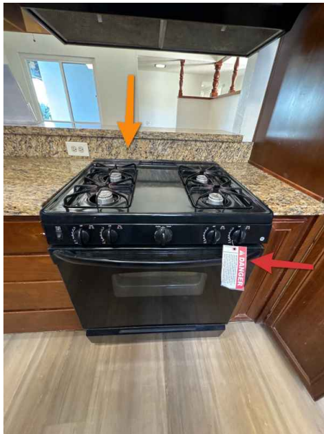
Kitchen, anti-tip bracket also missing
