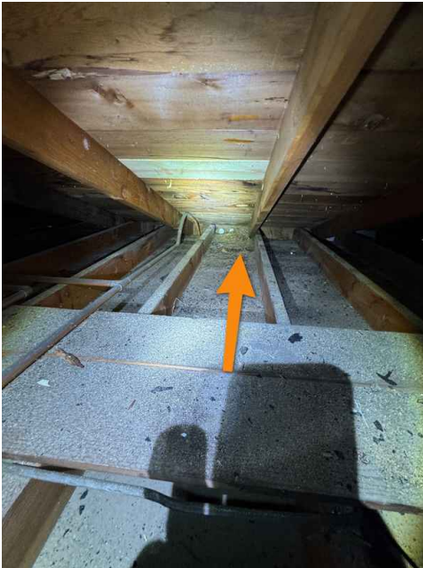
Example noted at Attic, Front
