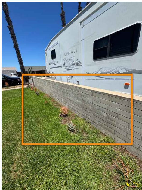
Example noted at Front Left Side Yard, no weep holes visible
