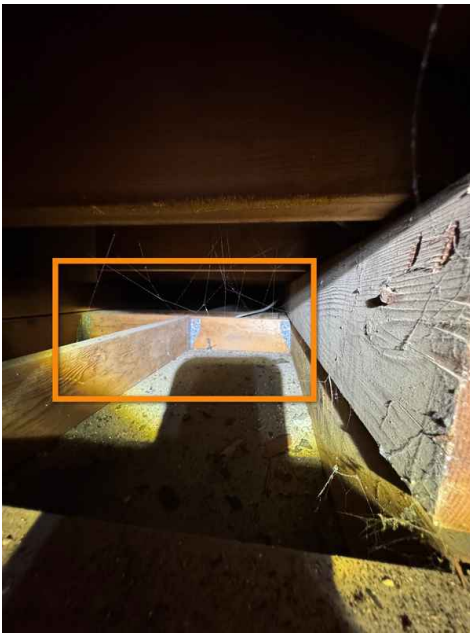
Example noted at Attic
