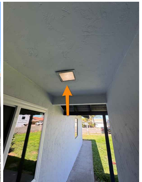
Example noted at Front Entry, loose
