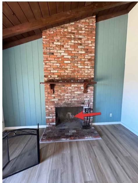
Example noted at Living Room Fireplace, missing permanent screen
