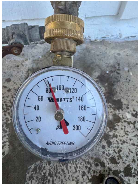
80-85 PSI, Water Pressure Gauge used
