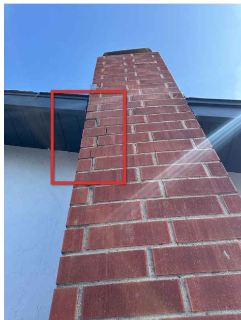
Example noted at Chimney, Right Side of Home
