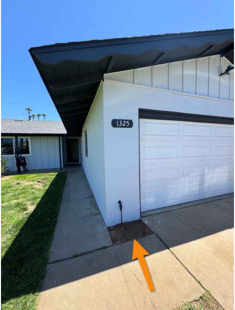
Example noted at Front of Home
