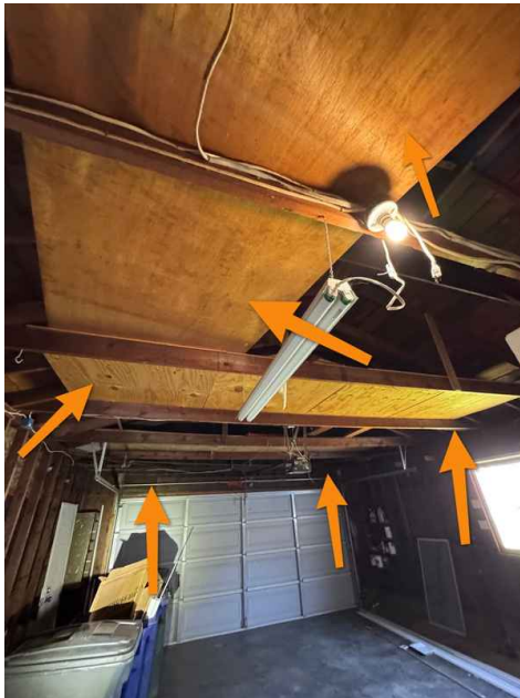
Example noted at Garage
