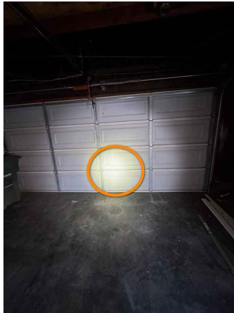
Example noted at Garage
