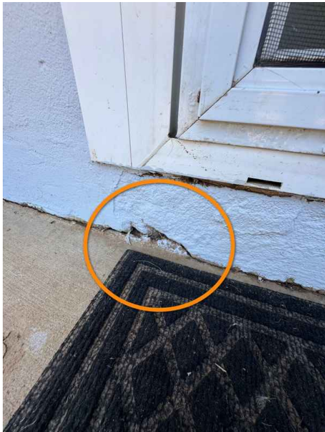
Example of damage noted
