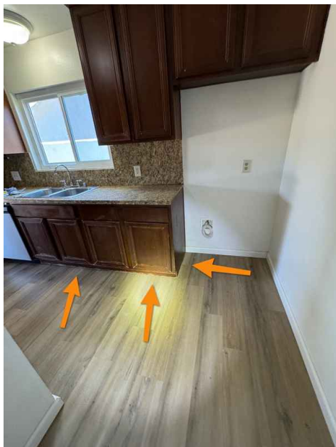
Example noted at Kitchen
