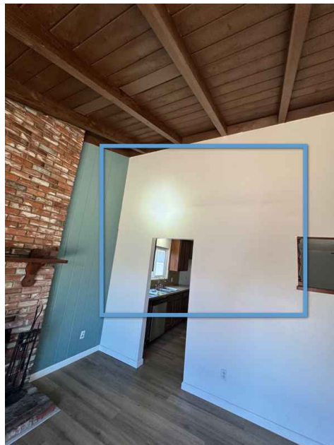
Example noted at Living Room
