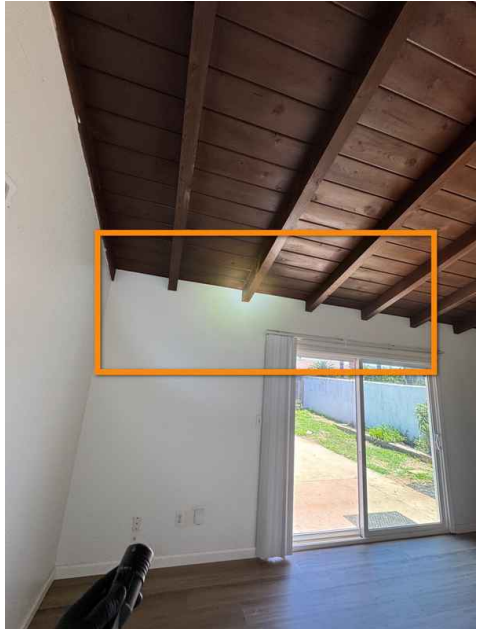
Example of Possible Repairs noted at Living Room
