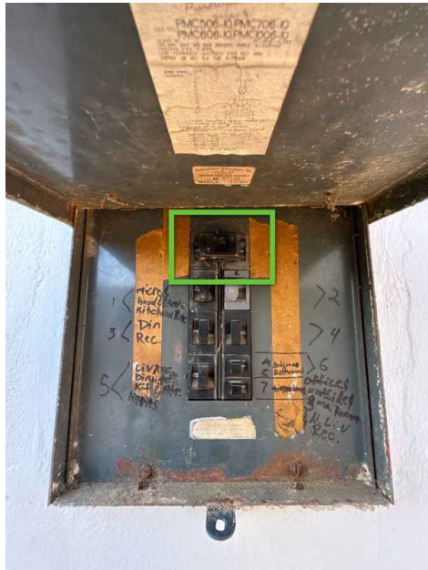
Main Panel, Electrical Service Disconnect
