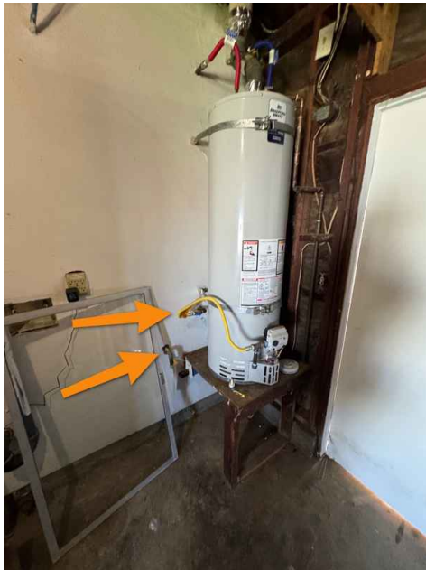
Example noted at Garage Rear
