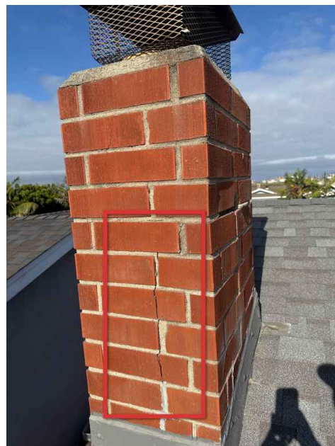
Example of cracking noted, Rear Roof
