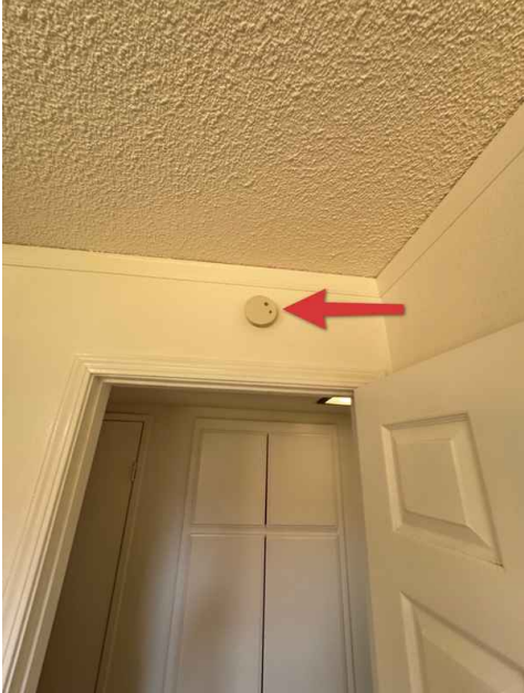
Example noted at Bedroom #3, inoperable
