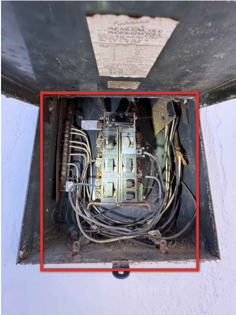
Dirt/Debris noted Inside Main Panel
