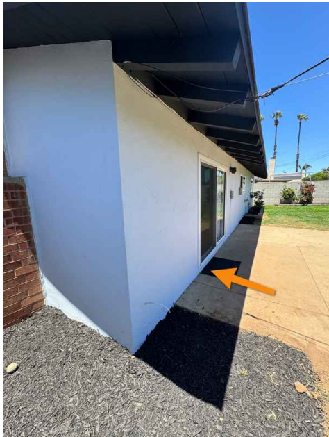
Example noted at Rear of Home
