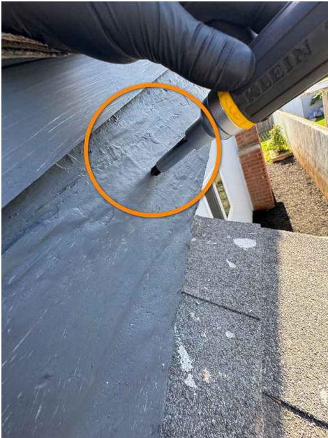
Example of moisture damage noted
