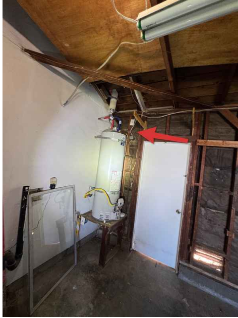
Example noted at Garage Rear
