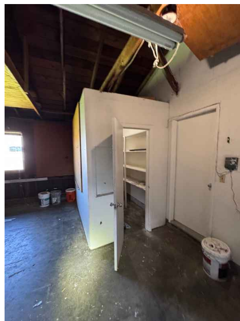
Example noted at Garage
