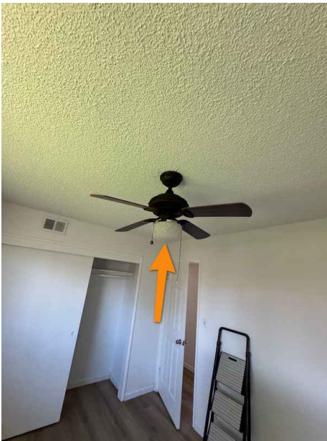
Example noted at Bedroom #2
