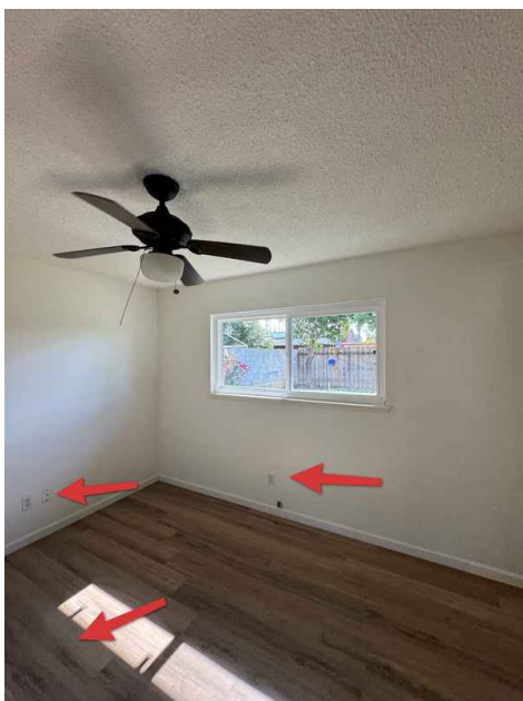
Example noted at Bedroom #2
