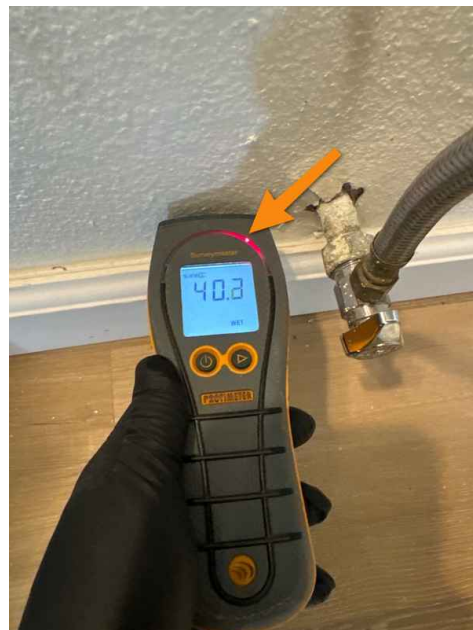
Elevated levels of moisture detected
