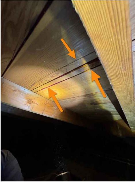
Example of damage noted, Attic
