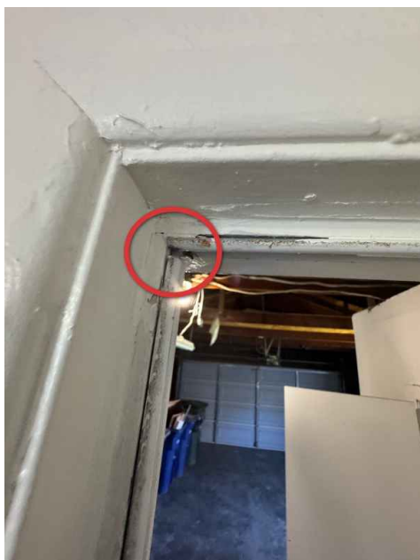
Example of inadequate seals noted at occupant doorway
