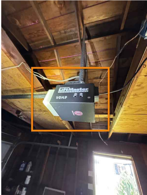
Garage automatic door opener missing battery backup
