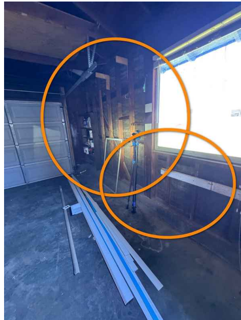
Example noted at Garage, Right Side facing outwards
