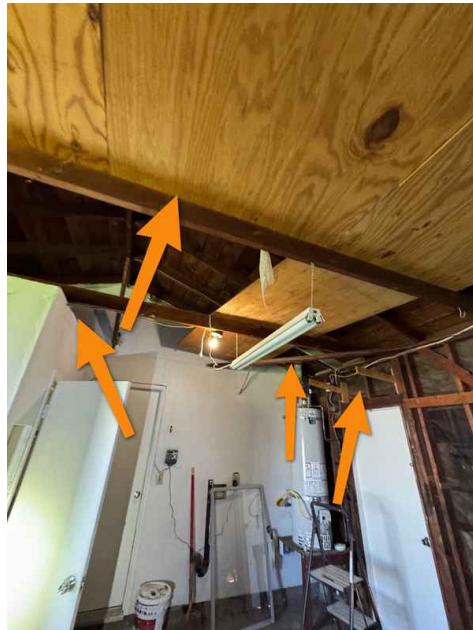
Example noted at Garage
