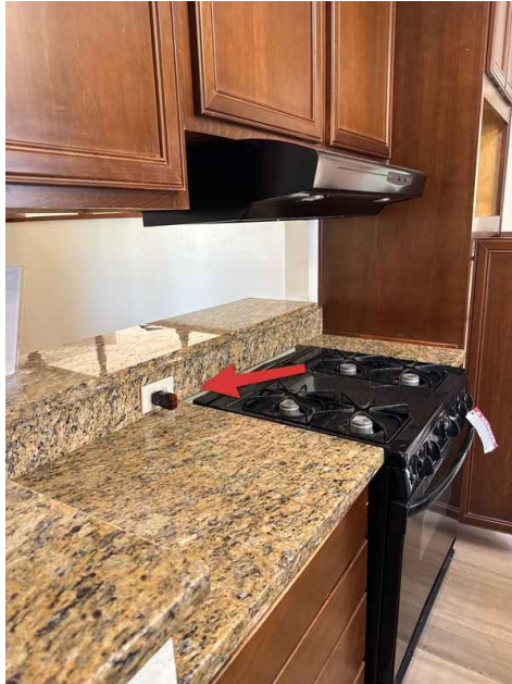
Example noted at Kitchen, loose
