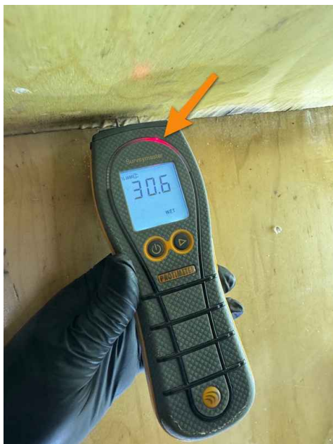
Elevated levels of moisture detected
