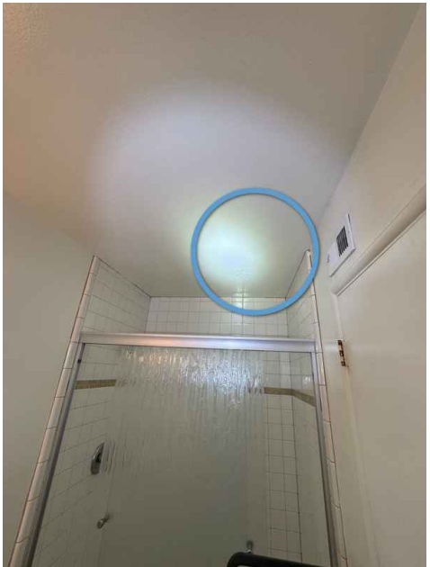
Example noted at Primary Bathroom Above Shower
