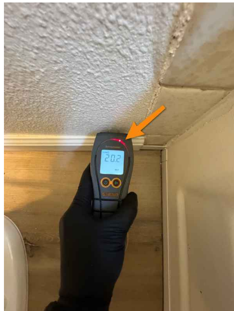
Elevated levels of moisture detected
