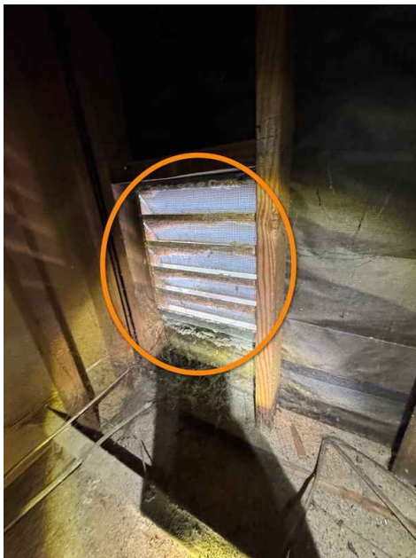
Example noted at Attic, Right Side
