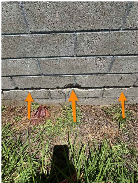
Example of cracking noted
