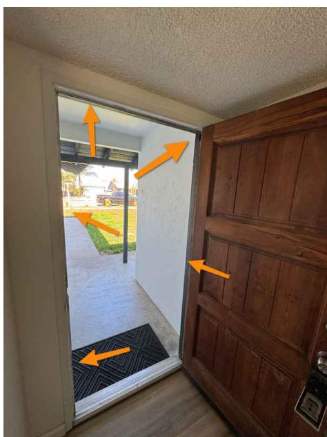
Example noted at Front Entry
