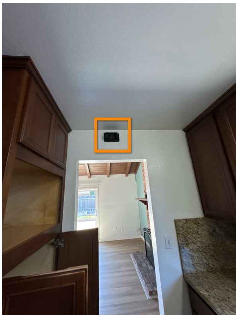
Example noted at Kitchen
