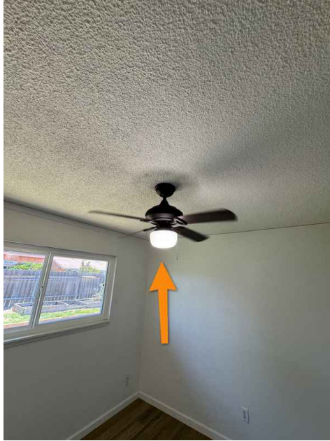
Example noted at Bedroom #3
