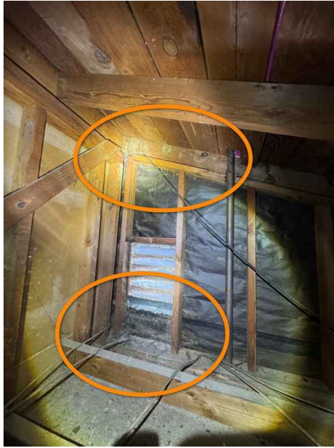
Example of staining noted at Attic
