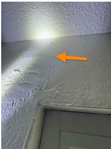
Example of crack noted
