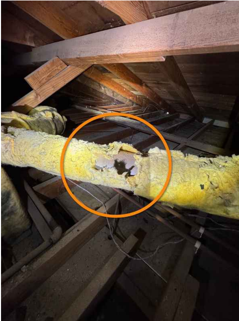
Example of damaged insulation noted, Attic
