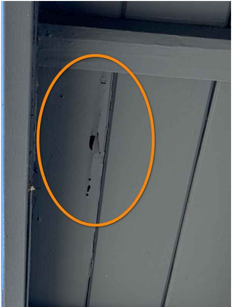
Example of damage noted
