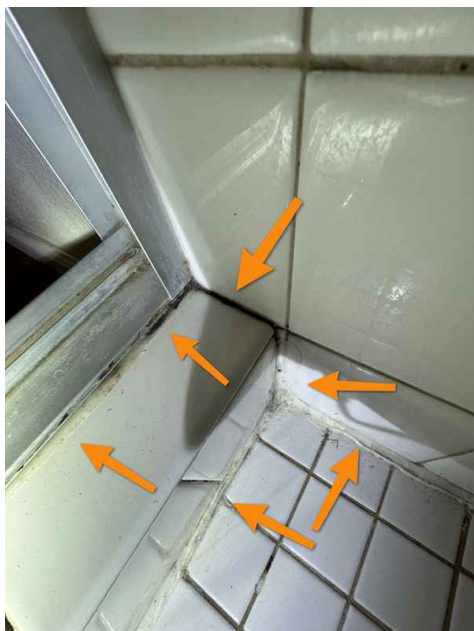
Example of Possible Repairs noted at Primary Bathroom Shower
