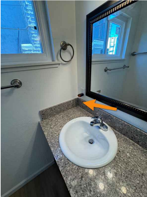
Example noted at Primary Bathroom Sink
