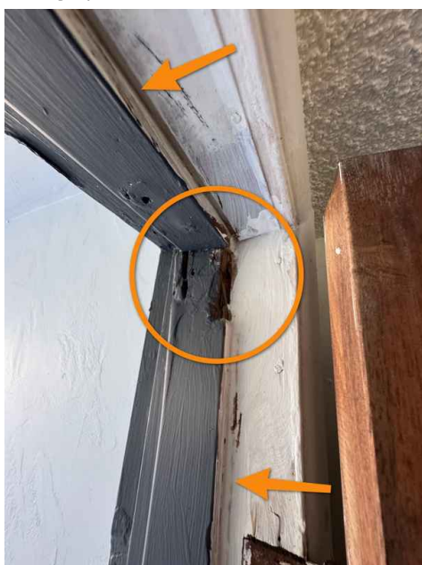
Example of damage, missing weather stripping noted
