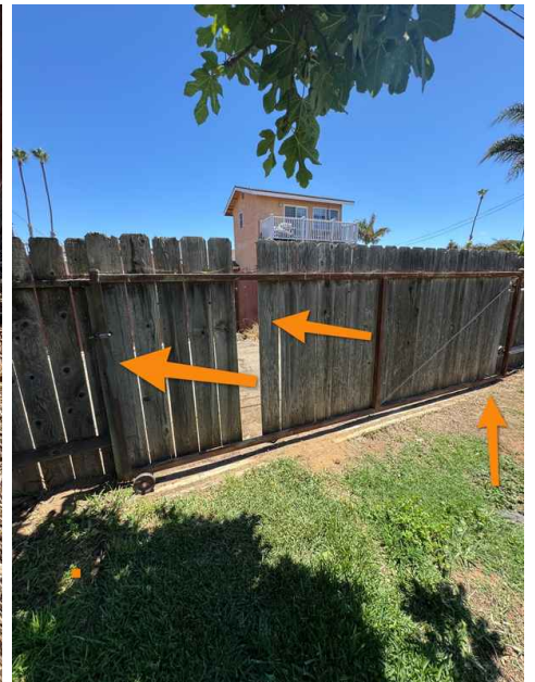
Example noted at Rear Yard, gate difficult to operate
