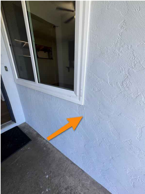
Example noted at Front Entry
