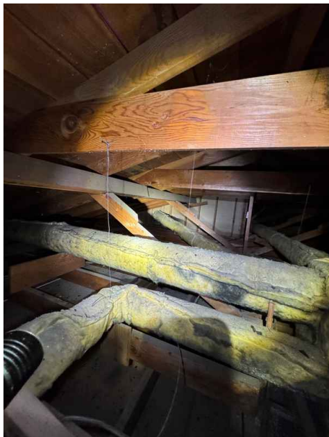
Example noted at Attic
