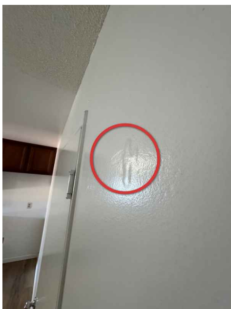
Example of failing paint noted
