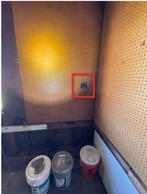
Example noted at Garage, Right Side facing outwards, missing faceplate
