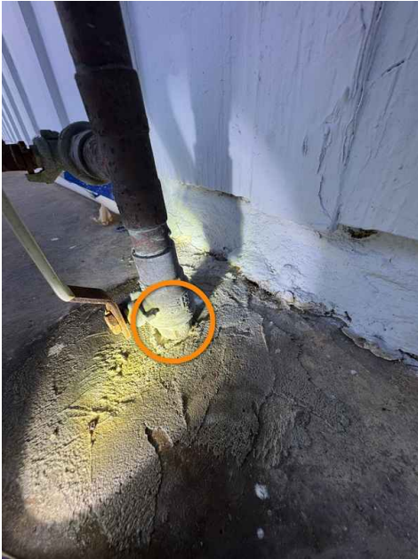
Main Water Shut-off pipe material undetermined
