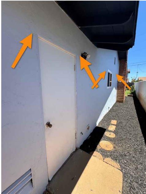
Example noted at Right Side of Home
