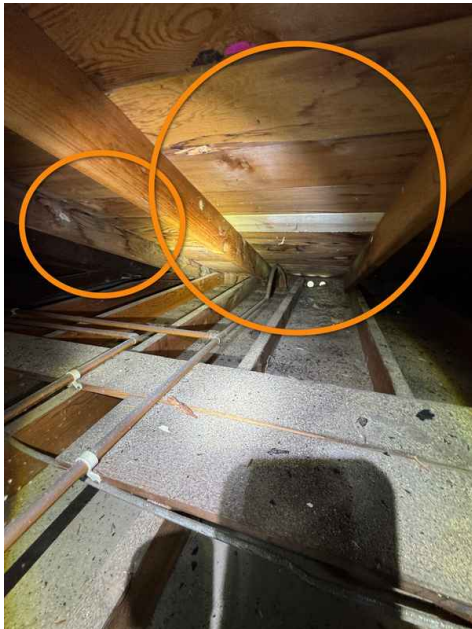
Example of staining and repairs noted at Attic
