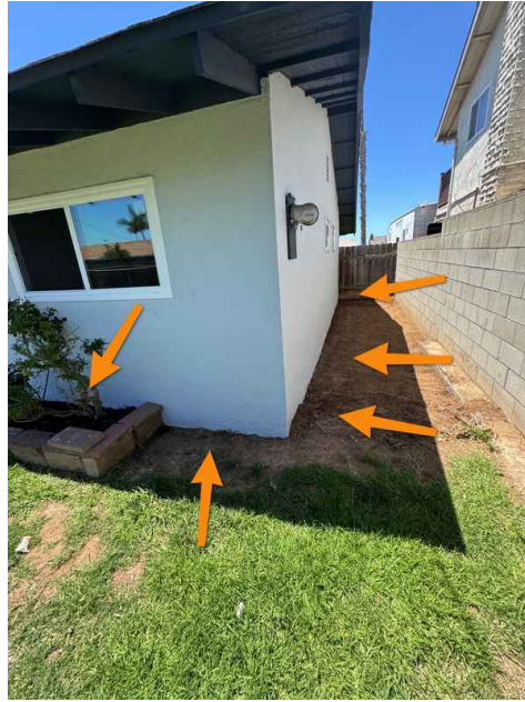
Example of damage, siding at grade noted at Rear, Left Side
