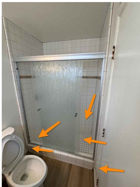
Example noted at Primary Bathroom Shower
