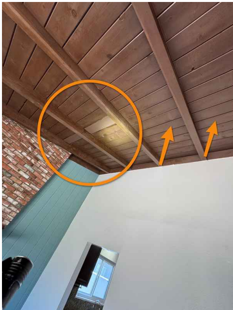
Example of repairs and staining noted at Living Room
