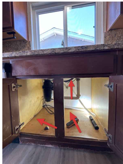
Example noted at Kitchen Sink
