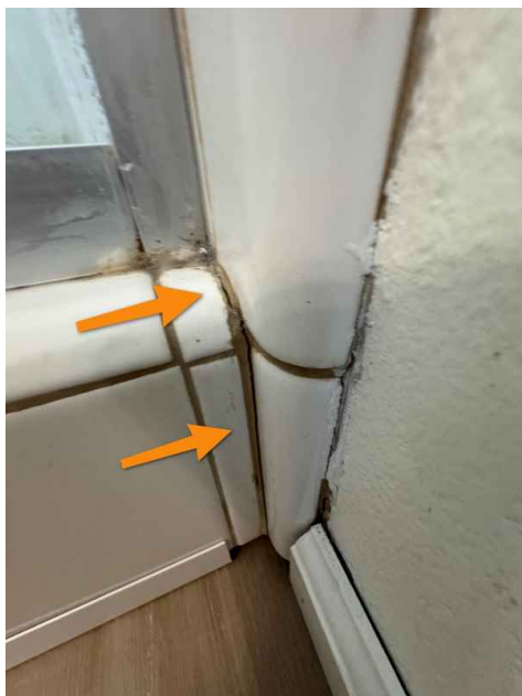
Example of failing grout noted
