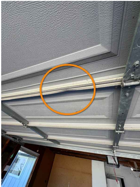
Example of damage noted
