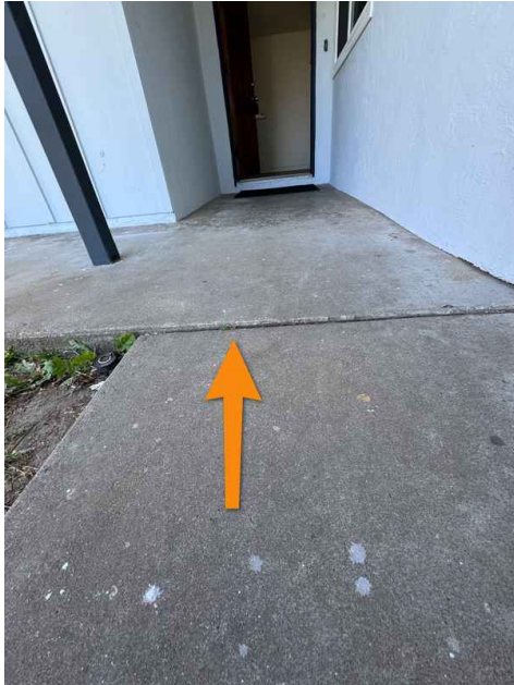
Example of heaving, possible tripping concern noted at Front of Home
