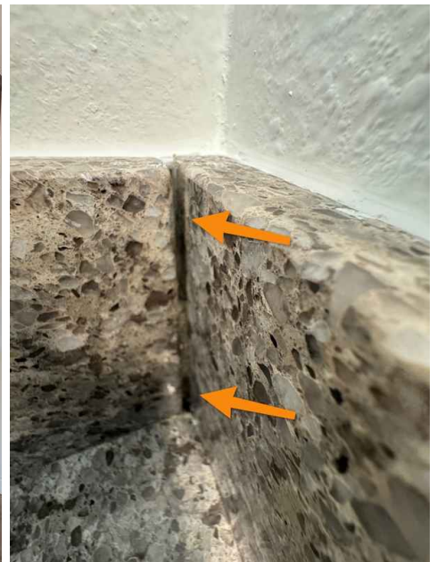
Example of missing grout noted
