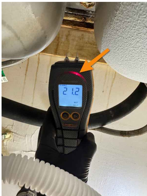
Elevated levels of moisture detected
