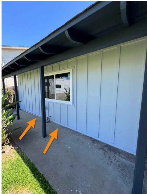
Example noted at Front Left Side of Home
