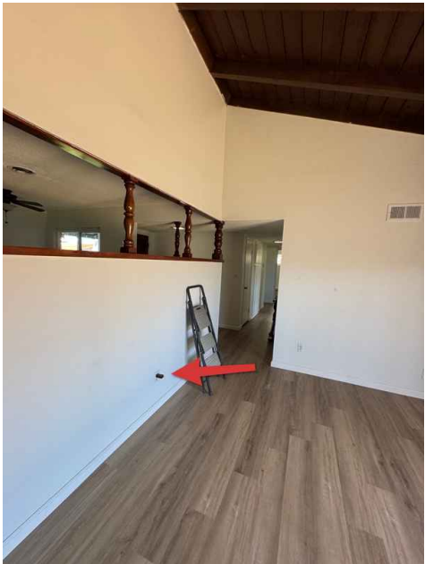
Example noted at Living Room, damaged
