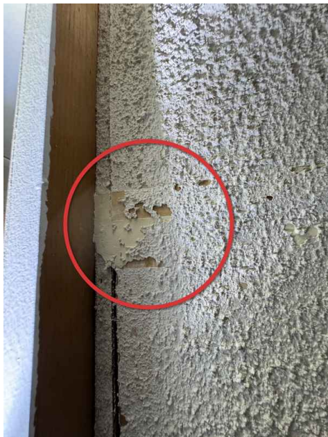
Example of damage noted
