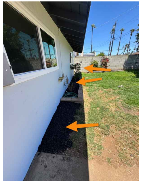
Example noted at Rear of Home
