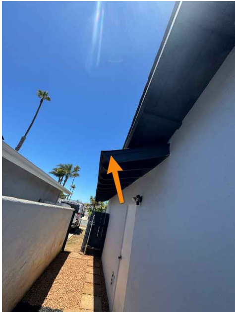
Example noted at Right Side Roof
