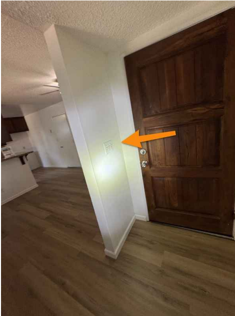
Example noted at Front Entry, missing screws
