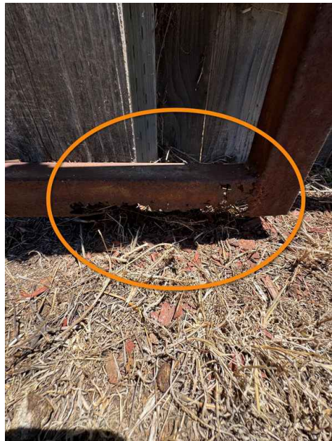
Example of rust and damage noted
