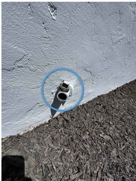
Cleanout cap not installed
