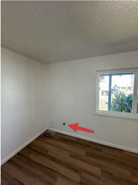
Example noted at Primary Bedroom, damaged
