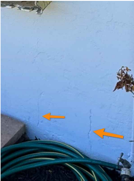
Example of cracks noted
