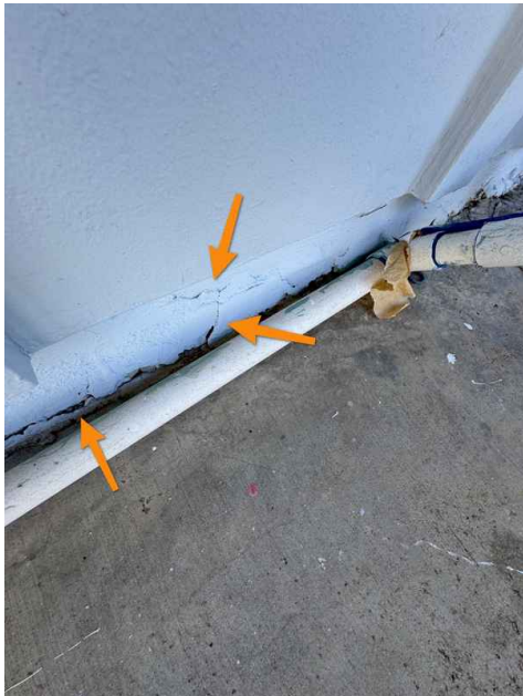
Example of cracking noted
