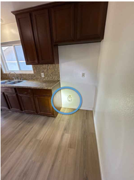
Example noted at Kitchen
