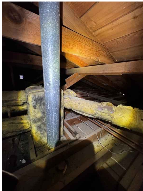
Example noted at Attic
