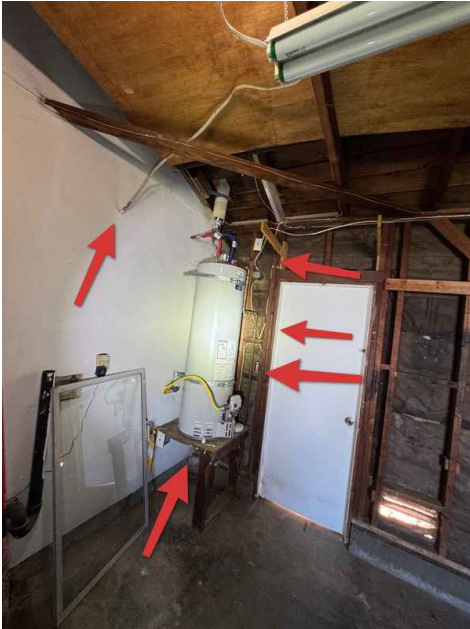
Example noted at Garage Rear
