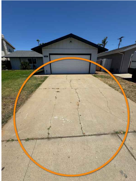
Example of cracks noted at Front driveway
