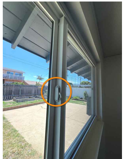
Example noted at Bedroom #3, lock sticks
