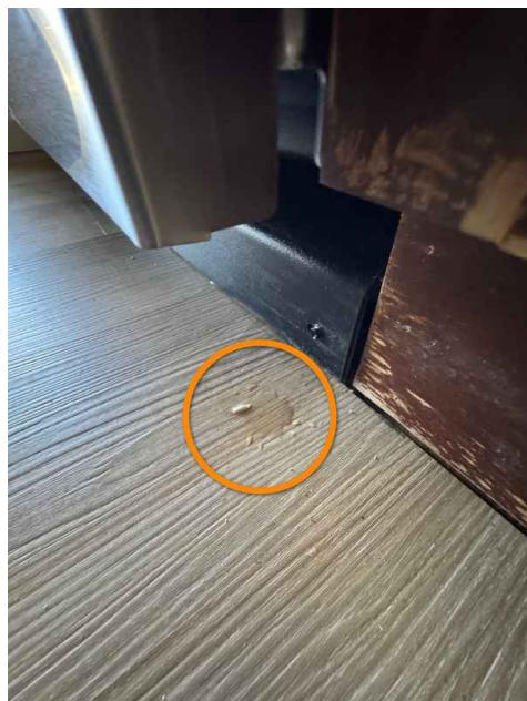
Water noted below unit
