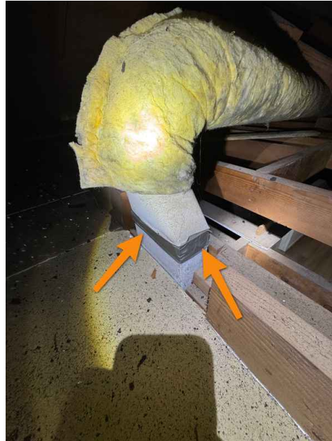
Example of aged duct tape noted at Attic
