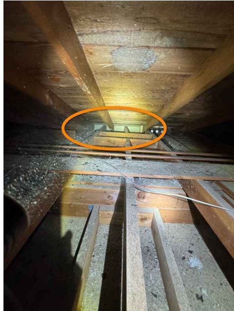
Example noted at Attic, Front
