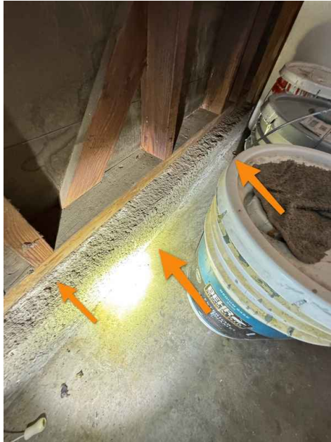
Example of efflorescence noted, Garage, Left Side facing outwards
