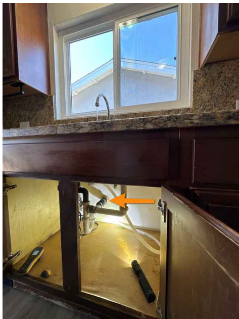
Example noted at Kitchen Sink
