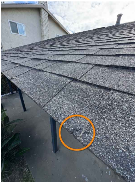
Example of damage noted, Front Left Side Roof
