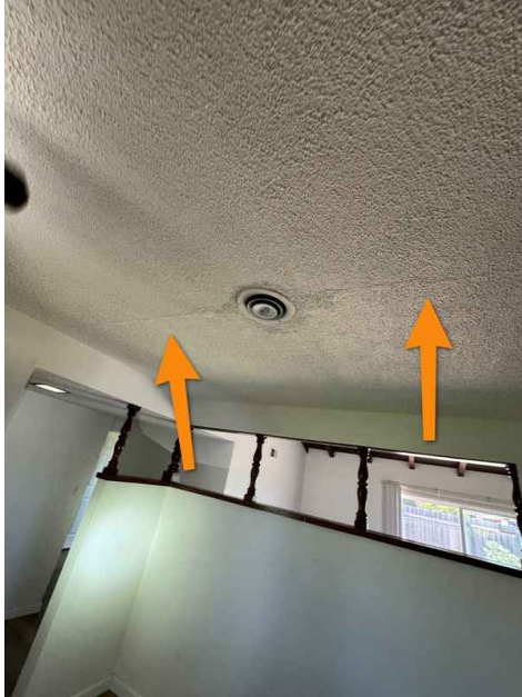
Example noted at Dining Room
