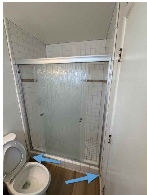
Example noted at Primary Bathroom
