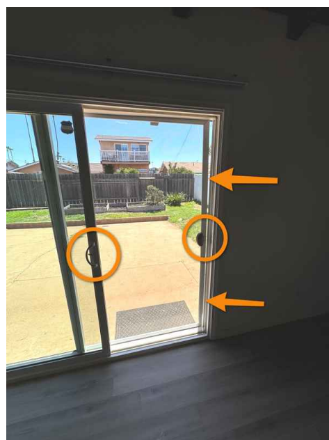
Example noted at Living Room, screen does not glide/latch, glass sliding door latch loose when closed
