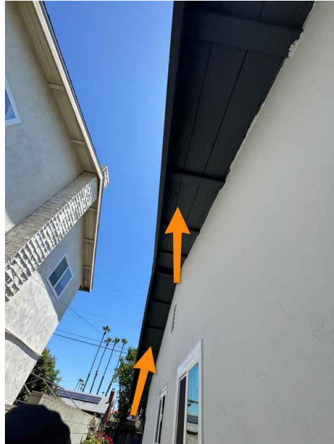
Example noted at Left Side Roof
