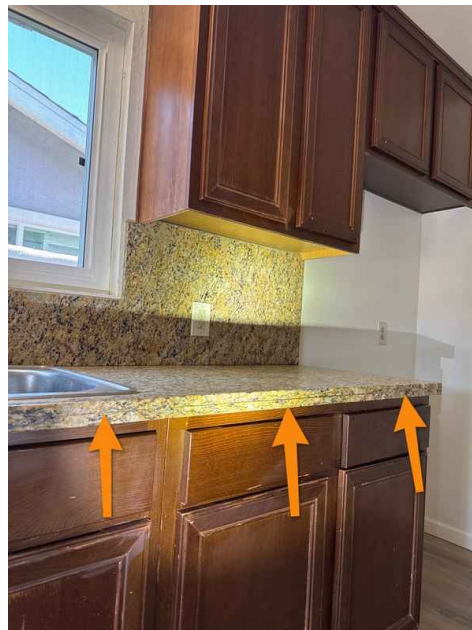
Example noted at Kitchen
