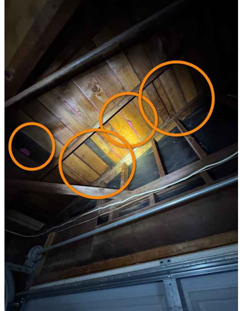
Example noted at Garage
