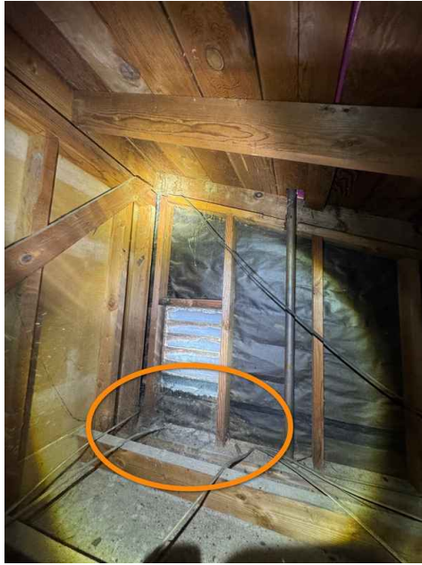
Example noted at Attic, Right Side
