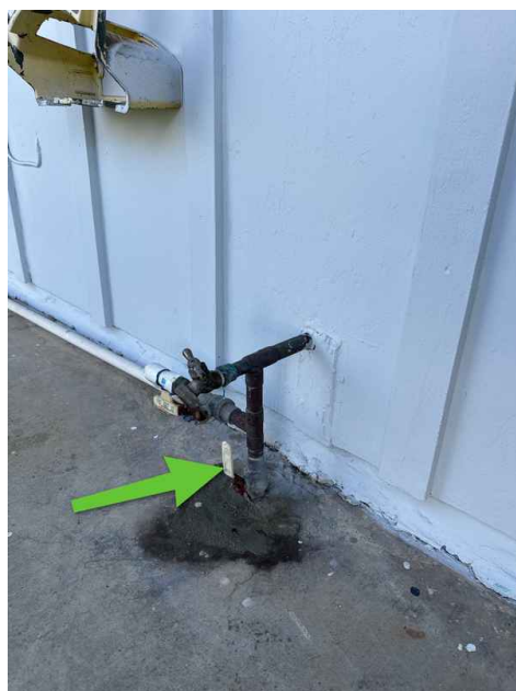
Main Water Shut-off Valve
