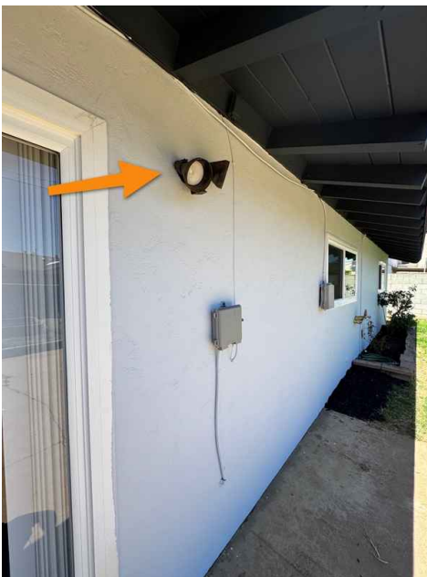
Example noted at Rear of Home
