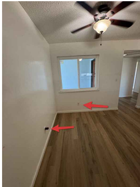
Example noted at Dining Room
