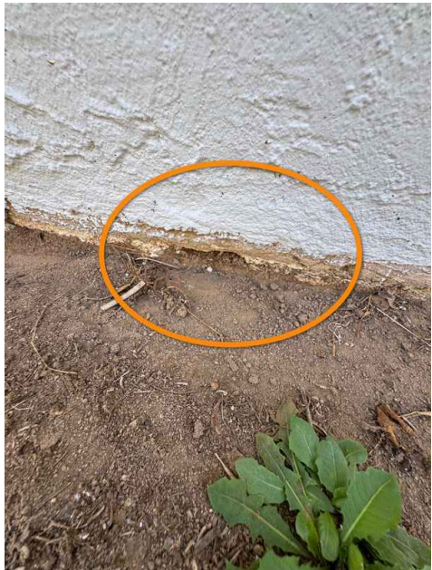
Example of damage noted
