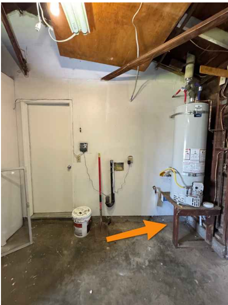
Example noted at Garage Rear
