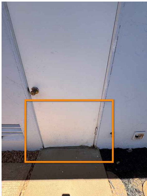
Example of moisture damage noted, Garage pedestrian door
