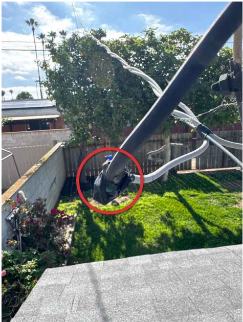
Example of damaged insulation noted, Rear Left Side Roof
