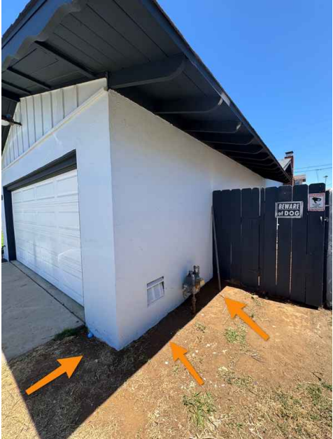
Example noted at Front, Right Side of Home
