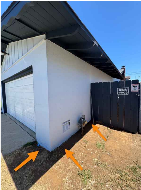
Example noted at Front, Right Side
