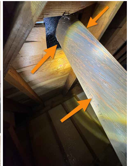
Example of moisture staining at duct noted at Attic
