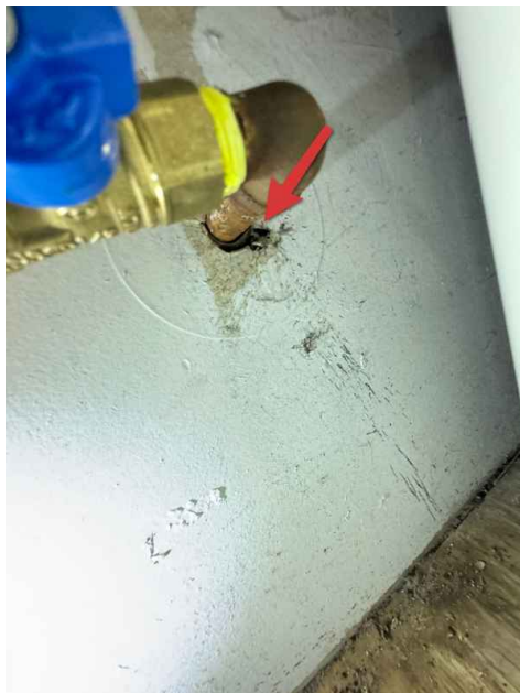
Example of gap noted
