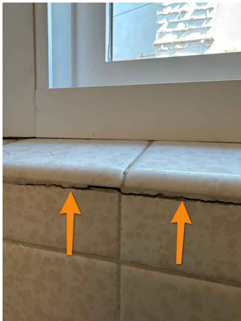
Example of loose tiles noted
