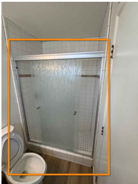
Example noted at Primary Bathroom Shower
