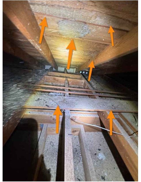
Example of staining noted at Attic
