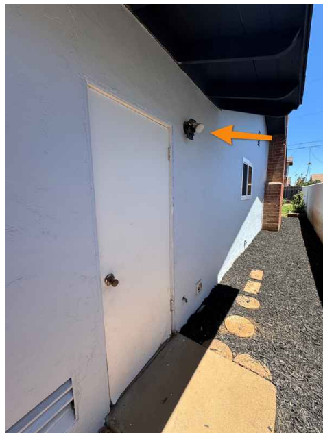
Example noted at Right Side of Home
