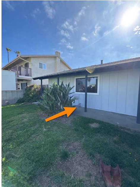
Main Water Shut-off, Front of Home
