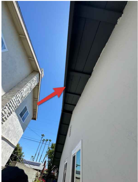
Example noted at Left Side of Home
