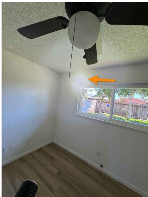
Example noted at Bedroom #2
