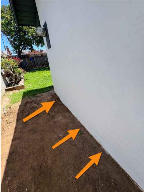
Example of damage and repairs noted, Rear Left Side of Home
