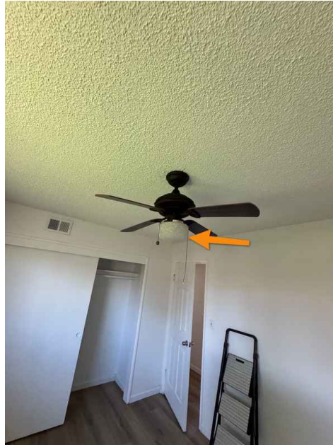
Example noted at Bedroom #2
