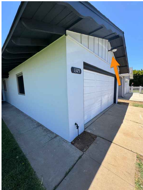
Example noted at Front of Home
