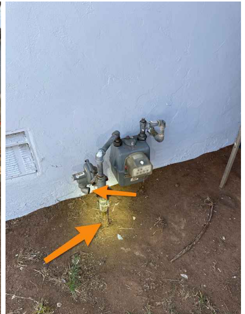
Example noted at Main Gas Shut-off, pipe noted loose
