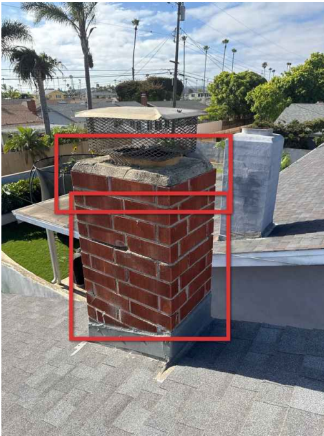
Example noted at Chimney, Rear Right Side Roof
