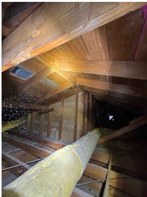
Example noted at Attic
