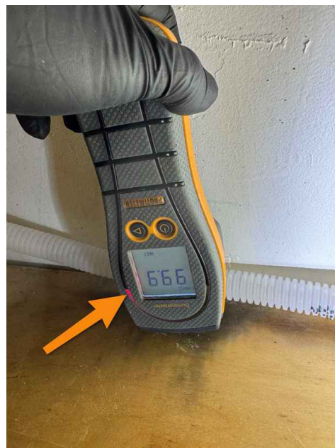
Elevated levels of moisture detected
