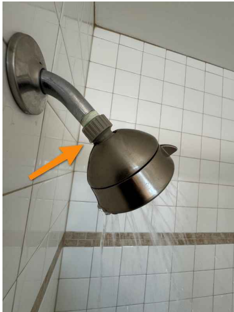
Primary Bathroom Shower, Appeared to be leaking from here
