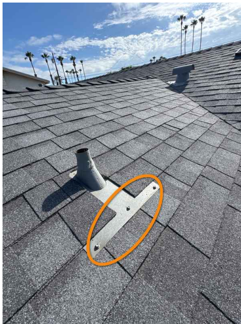
Example of expose nail heads noted
