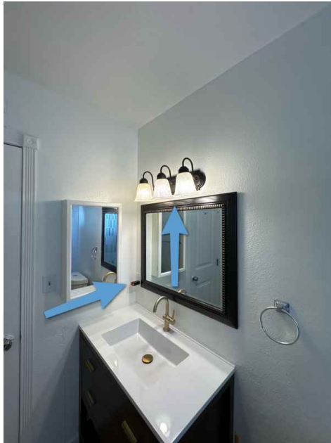
Example noted at Hall Bathroom
