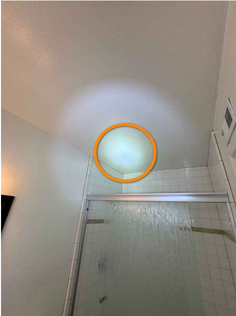
Example noted at Primary Bathroom Above Shower
