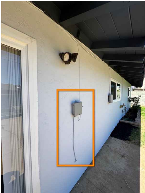
Example noted at Rear of Home
