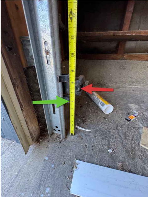
Example noted at Garage door photo eye sensors
