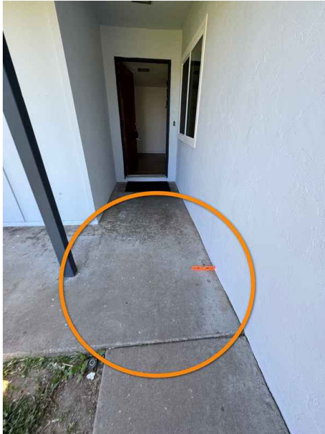
Example noted at Front of Home
