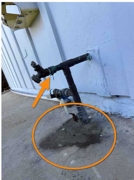
Appeared to be leaking from here
