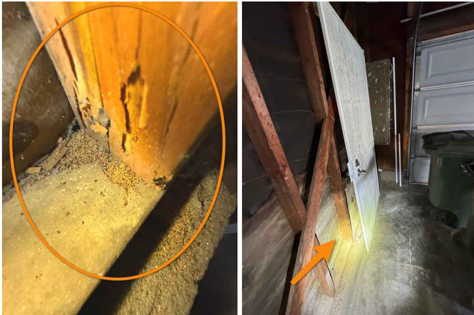
Example noted at Garage, Front Left Side facing outwards
