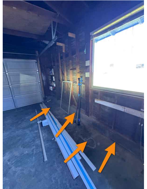
Example of efflorescence noted, Garage, Right Side facing outwards
