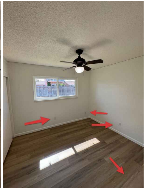
Example noted at Bedroom #3
