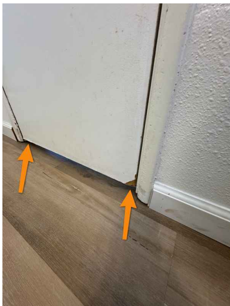
Example of damage noted, Primary Bathroom, stopper missing
