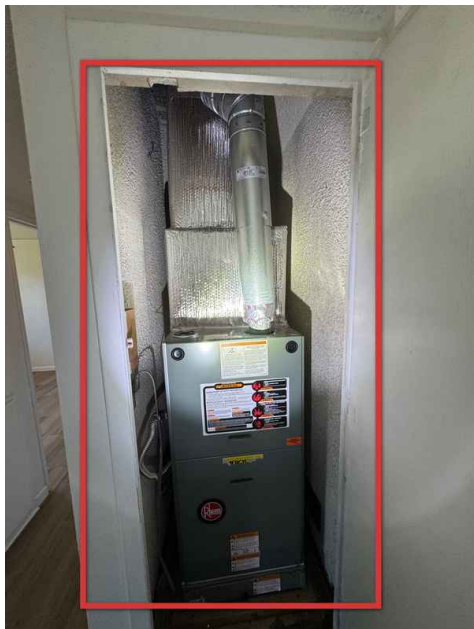
Example noted at Hallway Utility Closet
