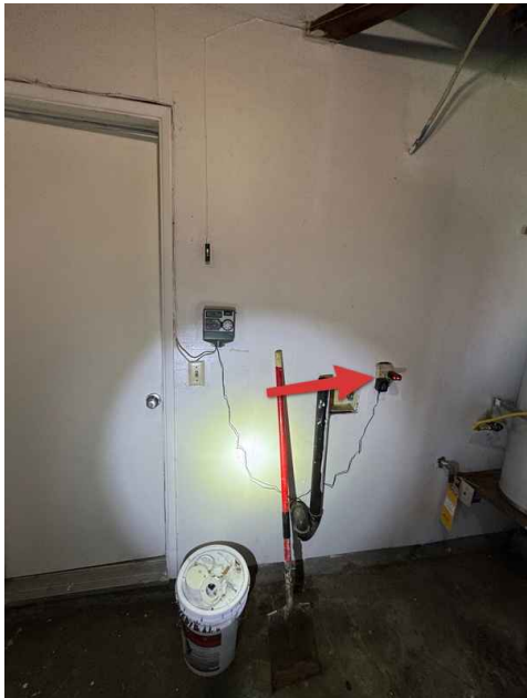
Example noted at Garage Rear, missing faceplate
