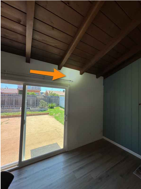
Example noted at Living Room
