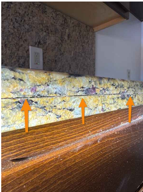
Example of cracking noted
