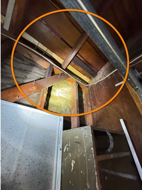
Example of staining, damage and repairs noted at Garage, Front Left Side facing outwards
