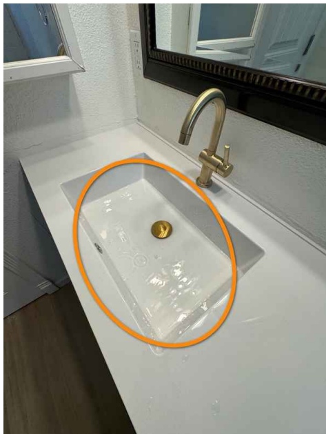
Hall Bathroom Sink
