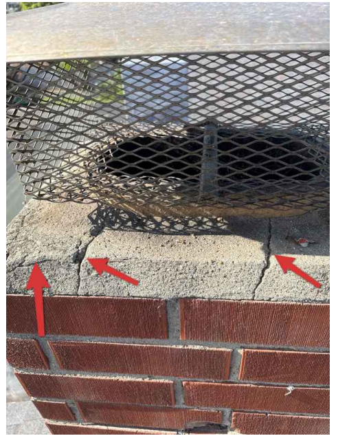
Example of cracking at crown noted
