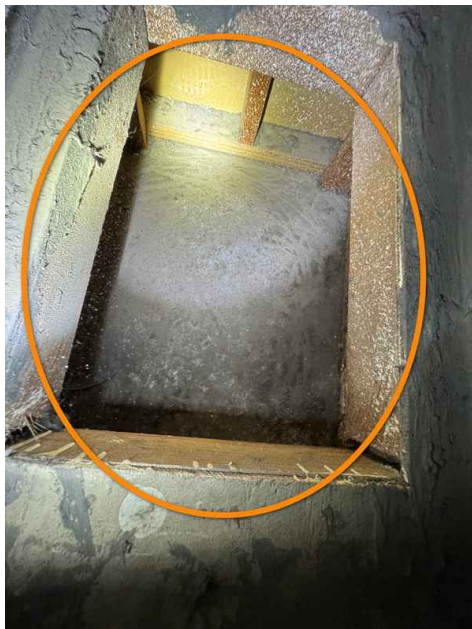
Dirt/Debris noted Inside return
