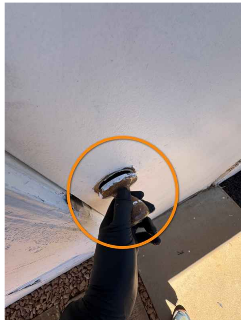
Garage pedestrian door handle loose
