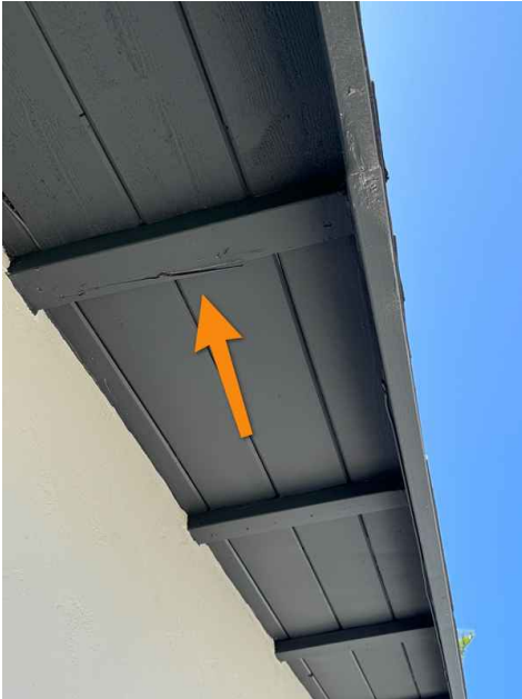
Example of damage noted
