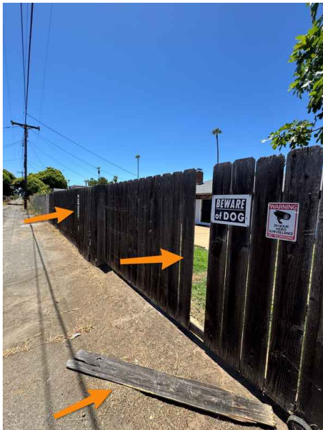
Example of damage noted, Rear Yard
