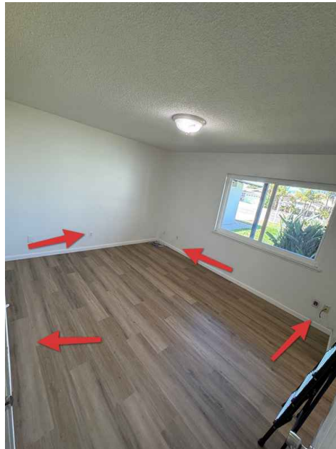
Example noted at Primary Bedroom
