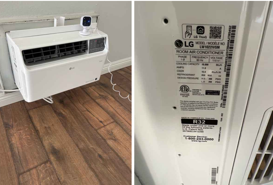
Photo of AC condenser
