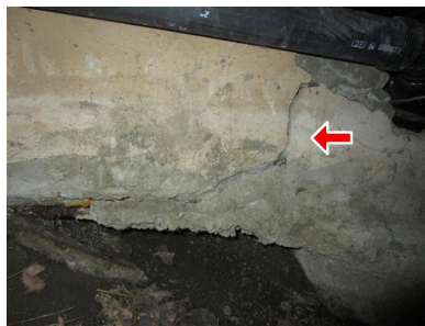
4.10 Item 2(Picture) below master bathroom
