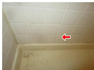
9.7 Item 1(Picture) guest bathroom shower
