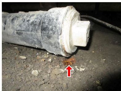
7.3 Item 4(Picture) south bedroom
