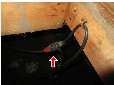
7.11 Item 2(Picture) extension chord use
