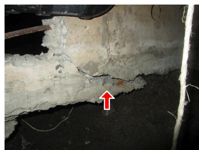
4.10 Item 1(Picture) below master bathroom
