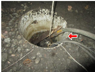
7.11 Item 3(Picture) improper installation
