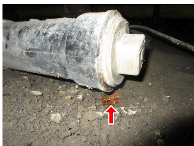
7.3 Item 4(Picture) south bedroom
