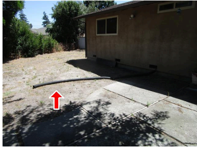
7.11 Item 1(Picture) drains to backyard
