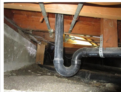
4.6 Item 9(Picture) guest bathroom shower
