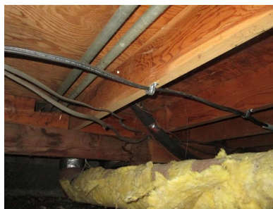
4.6 Item 5(Picture) water heater/furnace closet
