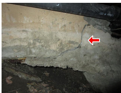
4.10 Item 2(Picture) below master bathroom
