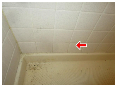
9.7 Item 1(Picture) guest bathroom shower
