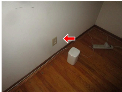
6.6 Item 5(Picture) south bedroom
