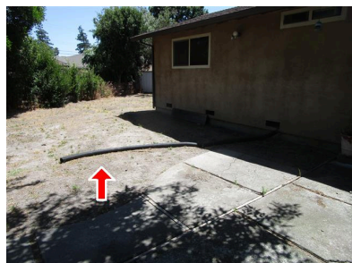
7.11 Item 1(Picture) drains to backyard
