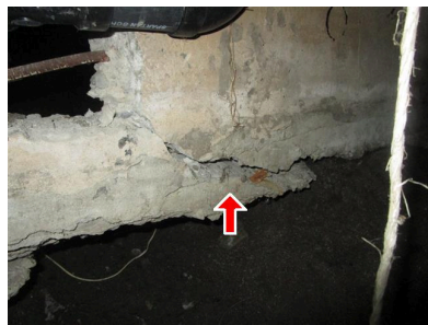
4.10 Item 1(Picture) below master bathroom
