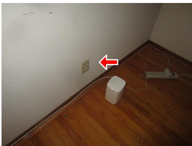
6.6 Item 5(Picture) south bedroom
