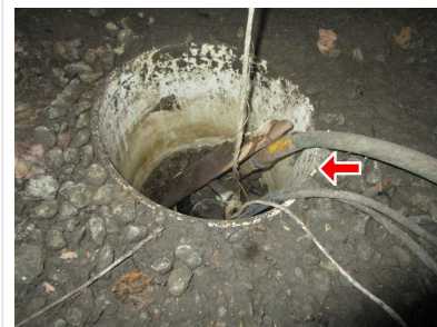
7.11 Item 3(Picture) improper installation
