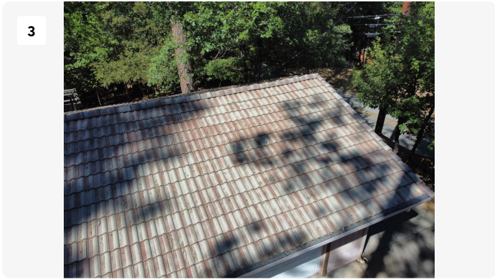
Project: 21919 Fallview Dr, Sonora, CA 95370, USA Date: Aug 14, 2026, 3:57 PM Creator: Steven Alvarez Tags: Roof Debris - Clean, Discontinued - Roma Tile
