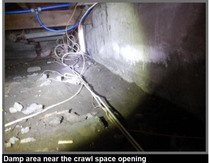
Damp area near the crawl space opening
