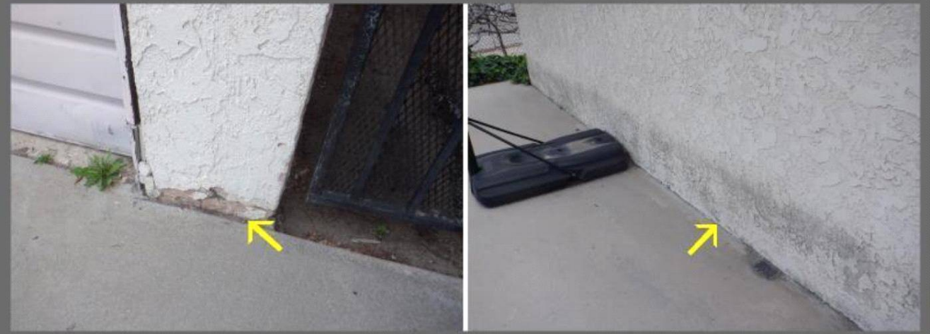
Deterioration & splatter marks
