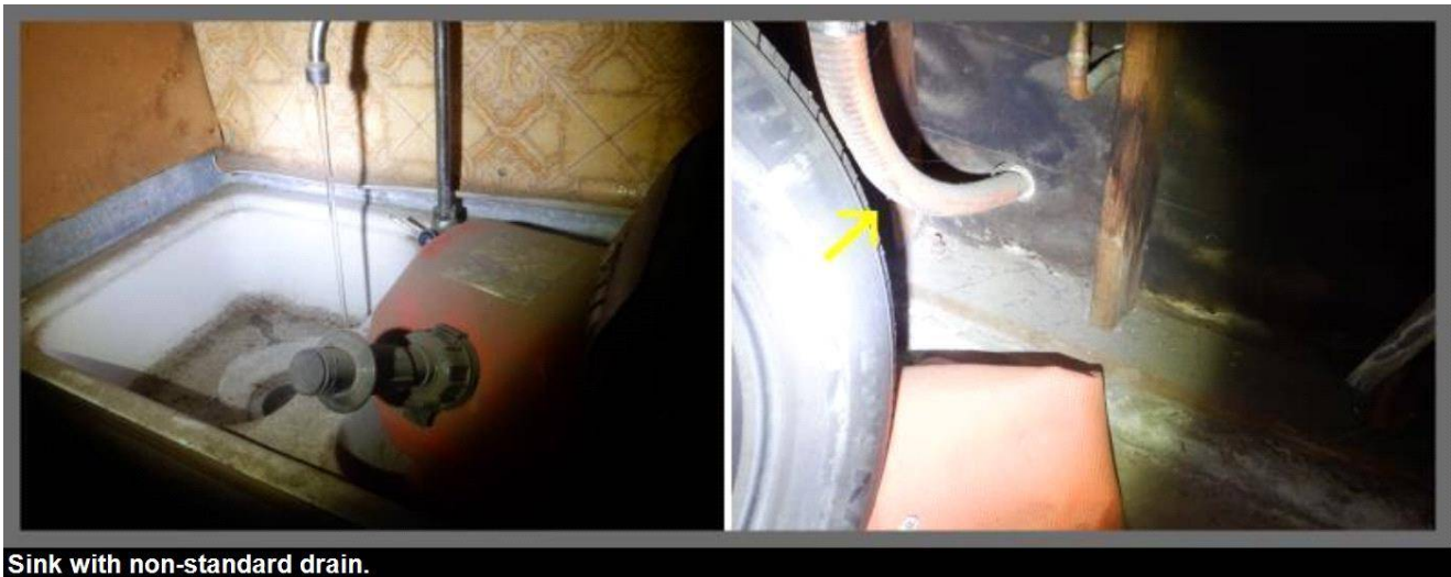
Sink with non-standard drain.
