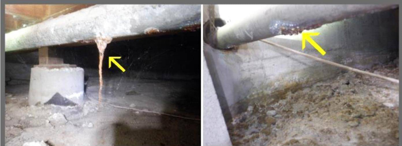
Rust blistering now leaking
