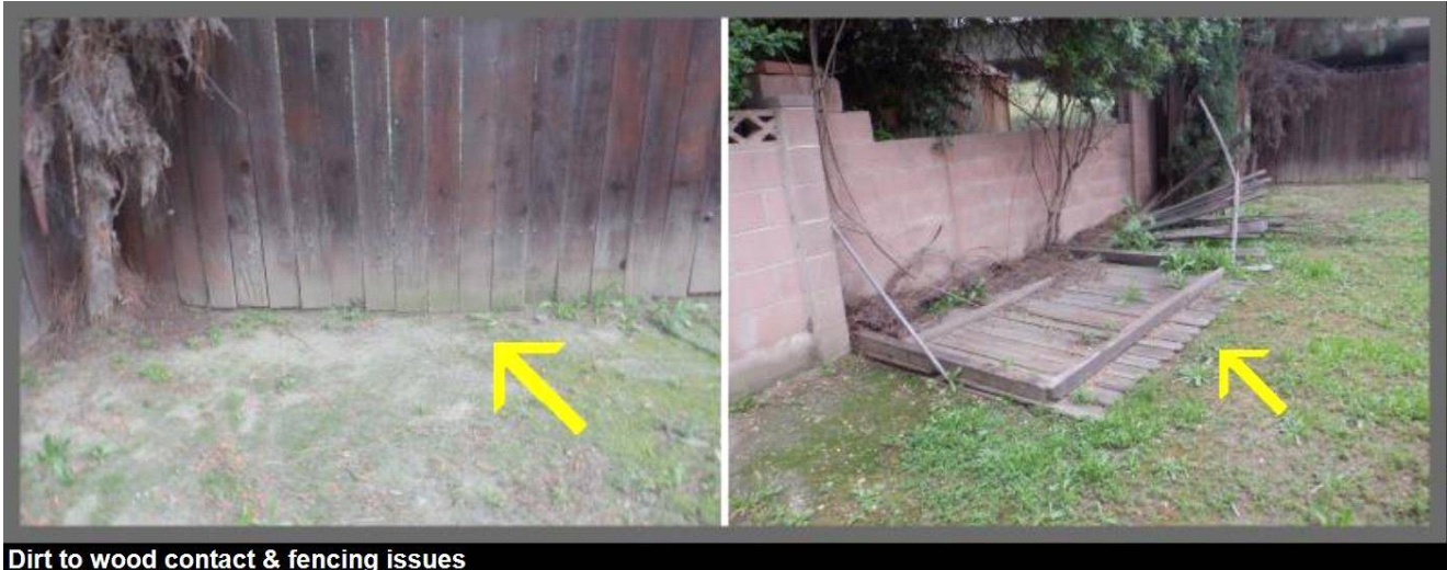
Dirt to wood contact & fencing issues
