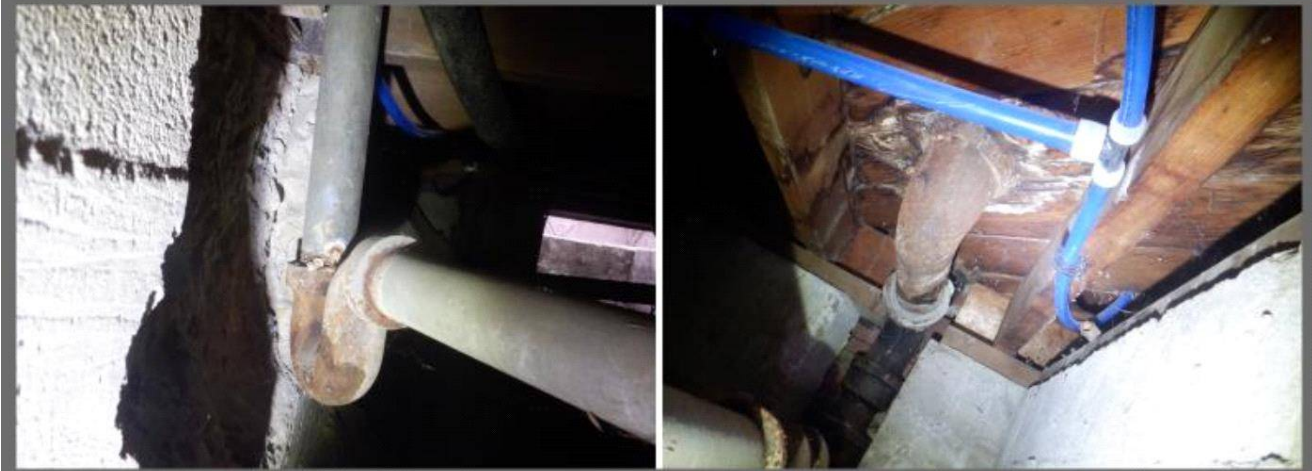
Galvanized steel & Cast iron piping
