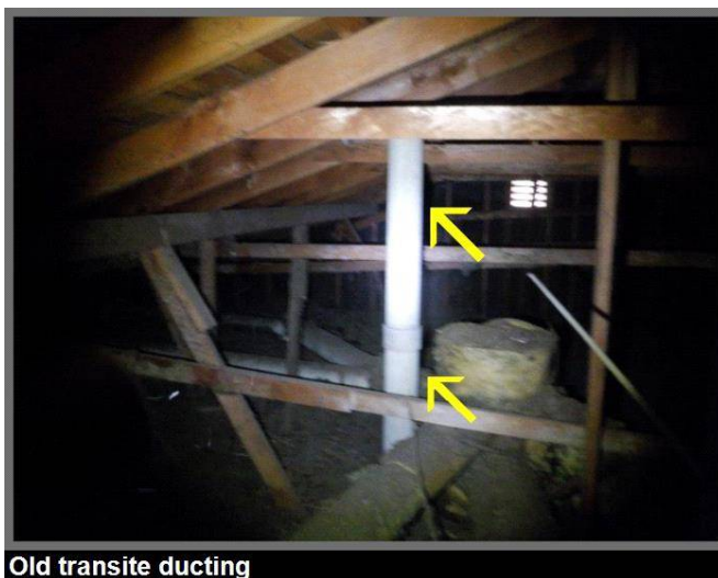
Old transite ducting
