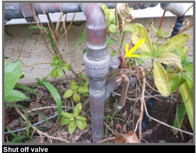
Shut off valve
