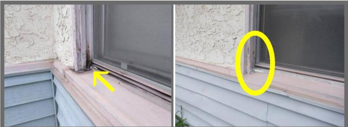
wood damage to window frames
