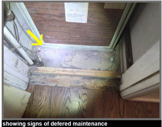
showing signs of defered maintenance
