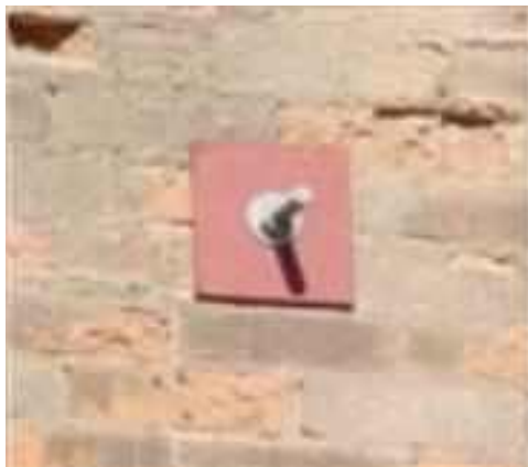
A steel plate with anchor bolts.
