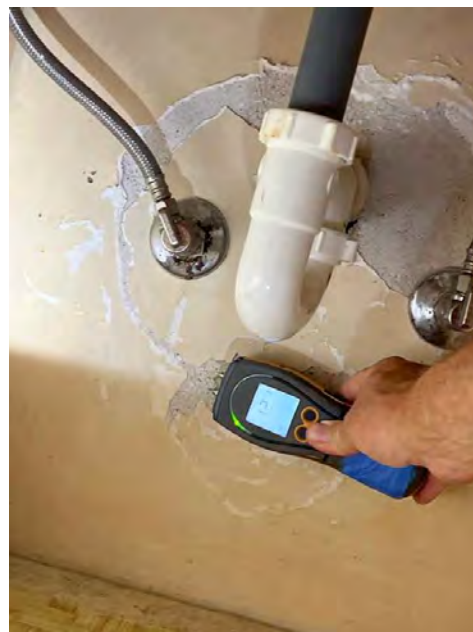
Upstairs Hall Bathroom Moisture Meter Dry Reading
