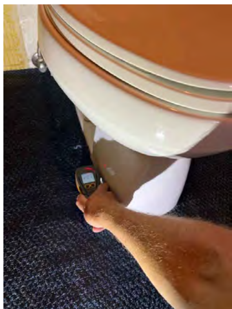
Master Bathroom Moisture Meter Wet Reading
