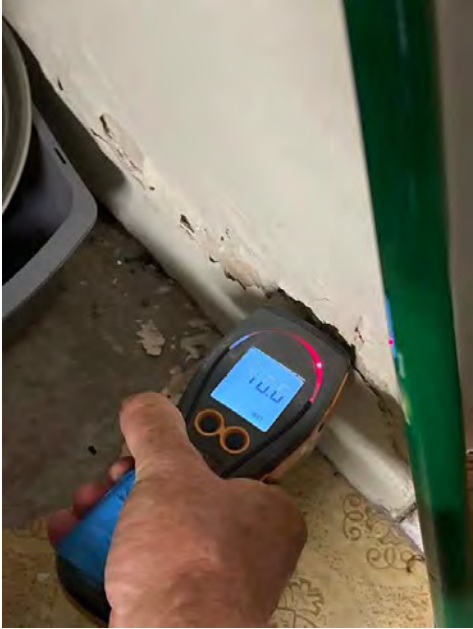
Laundry Room Moisture Meter Wet Reading
