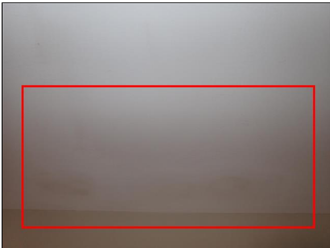
3.1 Item 1(Picture) Kitchen ceiling.
