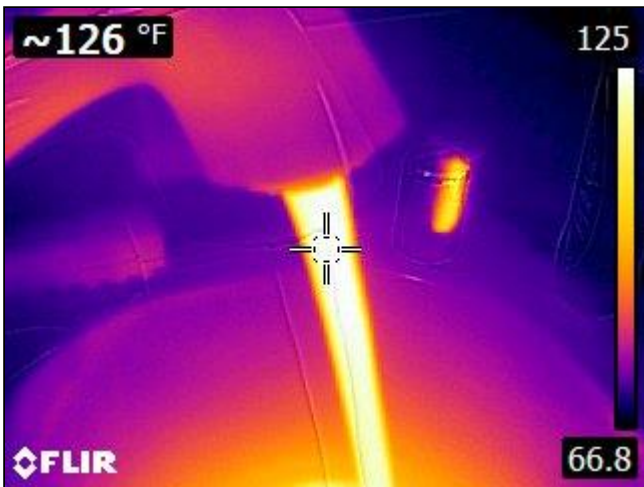
2.5 Item 1(Picture) Thermal image of water heater producing hot water.
