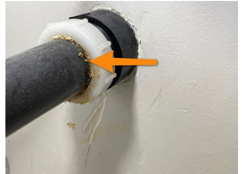
Example Noted at Hall Bathroom
