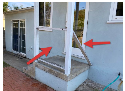
Example Noted at Backyard
