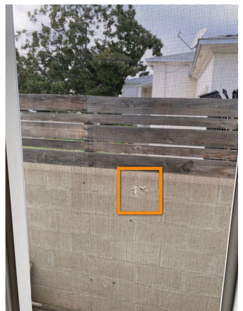
Example Noted at Master Bedroom
