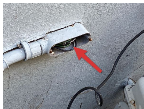
Example Noted at Left Side Yard
