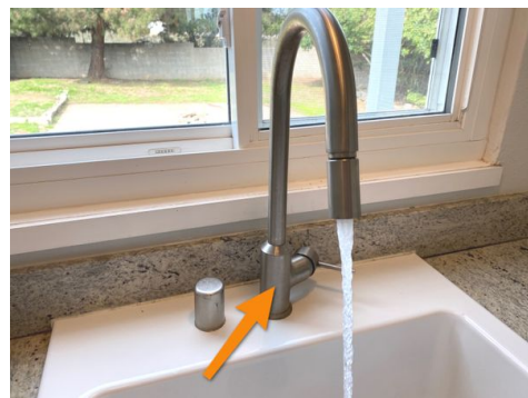
Example Noted at Kitchen
