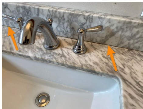
Example Noted at Hall Bathroom
