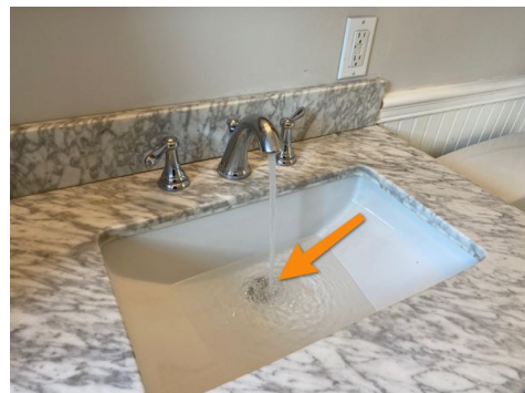
Example Noted at Hall Bathroom
