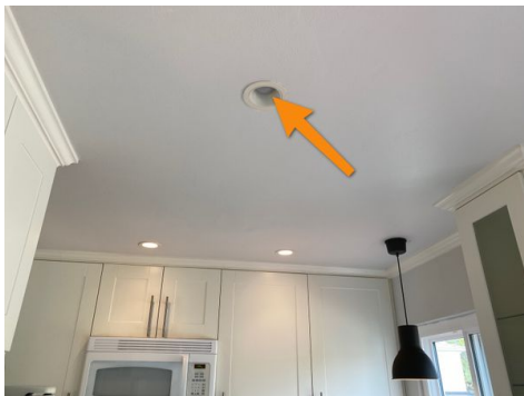
Example Noted at Kitchen
