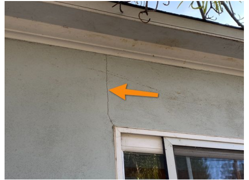
Example Noted at Backyard
