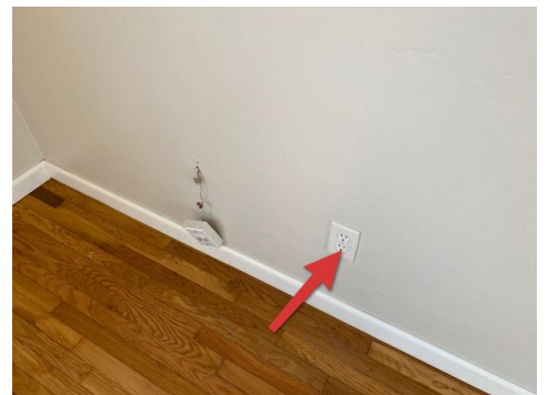
Example Noted at Master Bedroom
