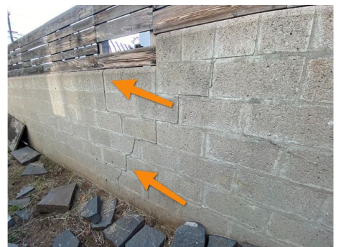
Example Noted at Left Side Yard
