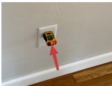
Example Noted at Master Bedroom
