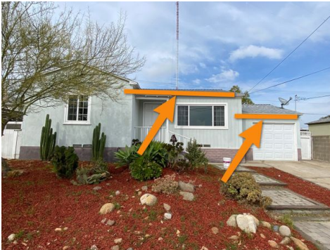
Example Noted at Front Yard
