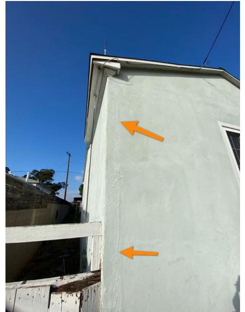
Example Noted at Front Yard
