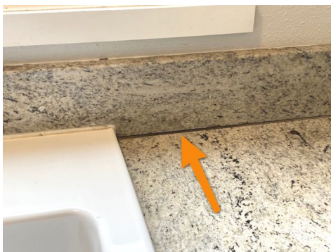
Example Noted at Kitchen
