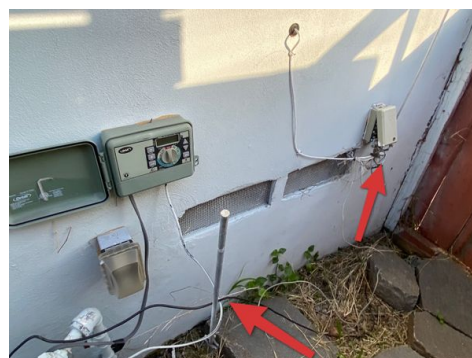
Example Noted at Left Side Yard
