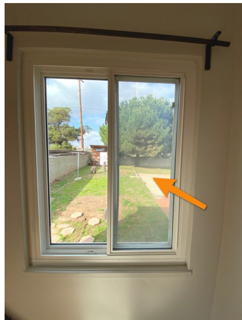
Example Noted at Bedroom #2
