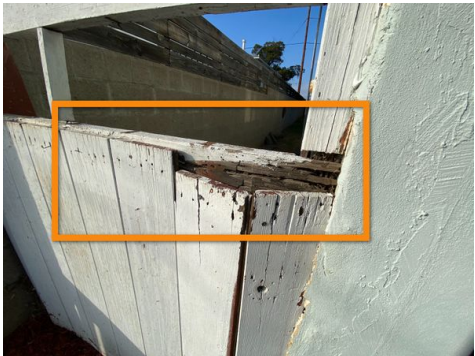
Example Noted at Left Side Yard
