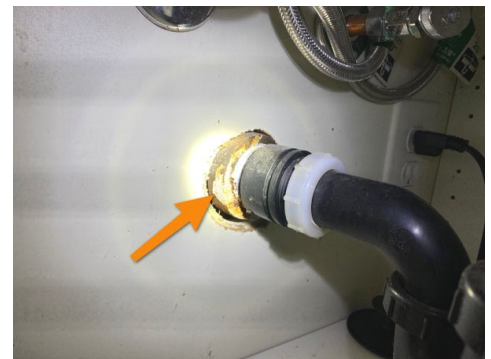
Example Noted at Kitchen
