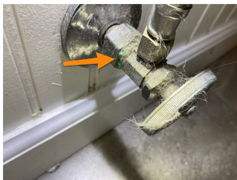
Example Noted at Hall Bathroom toilet
