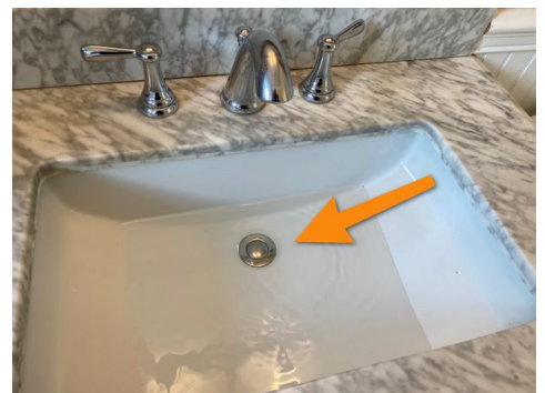
Example Noted at Hall Bathroom
