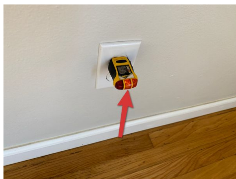
Example Noted at Bedroom #2
