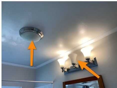
Example Noted at Hall Bathroom
