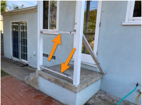
Example Noted at Backyard
