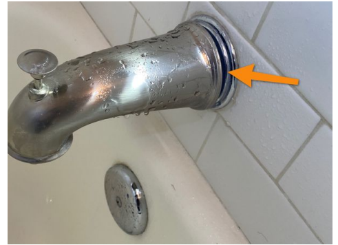
Example Noted at Hall Bathroom
