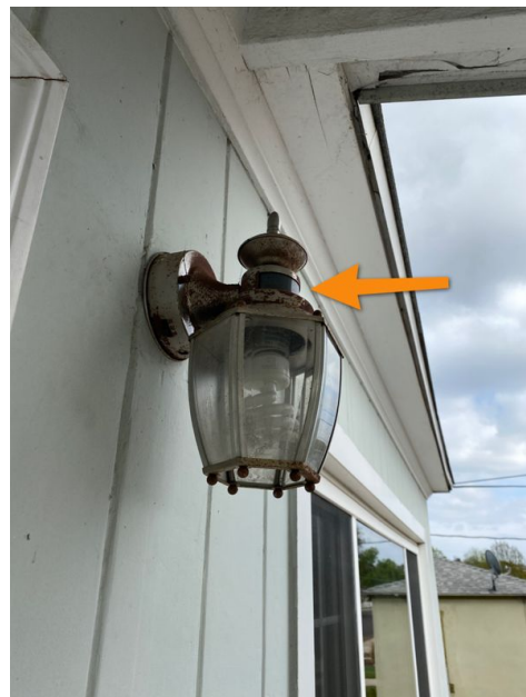
Example Noted at Front Yard
