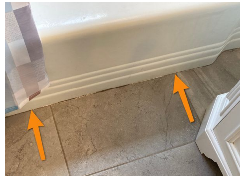
Example Noted at Hall Bathroom
