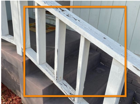
Example Noted at Front Yard
