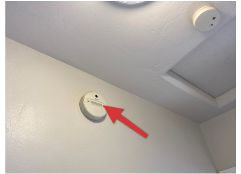
Example Noted at hallway
