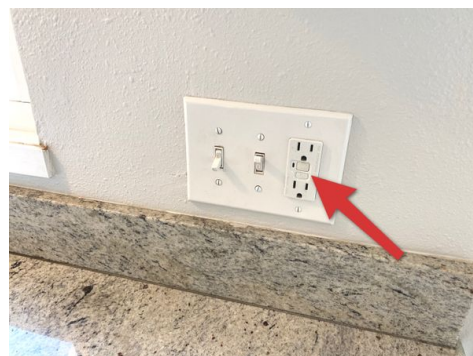
Example Noted at Kitchen
