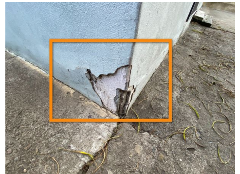
Example Noted at Backyard
