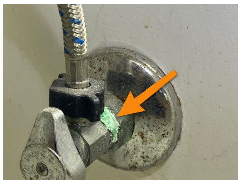
Example Noted at Hall Bathroom
