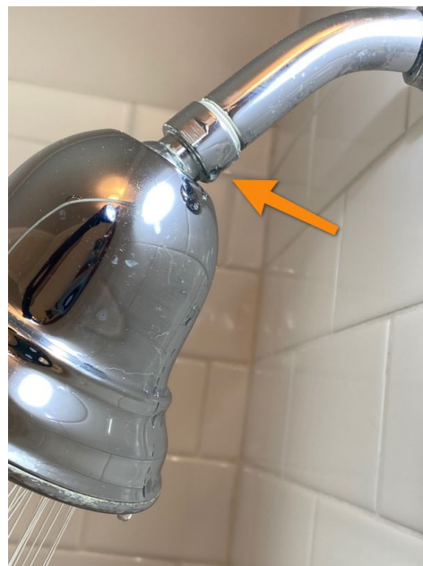
Example Noted at Hall Bathroom
