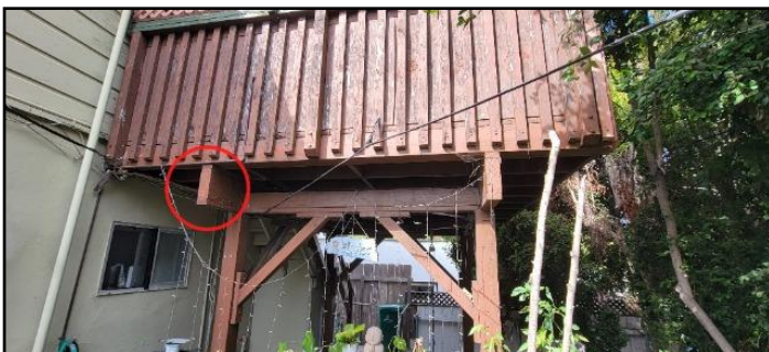
Insect damage at beam
