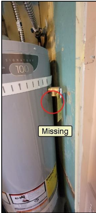
TPR discharge issue
