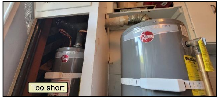
TPR discharge issue
