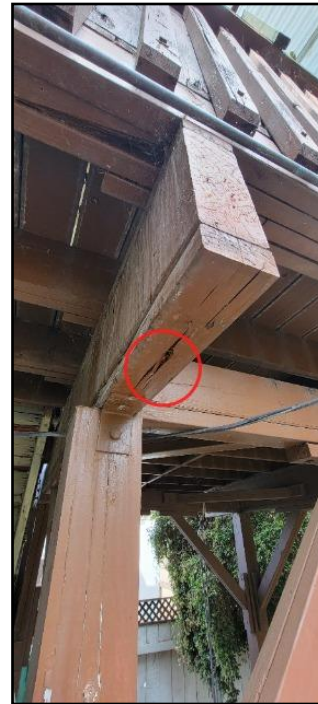
Termite damage here
