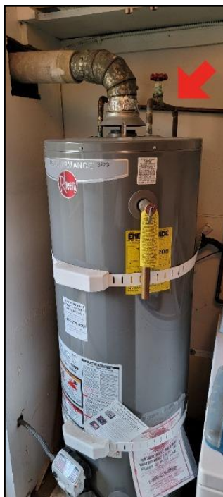
Rigid water supply lines
