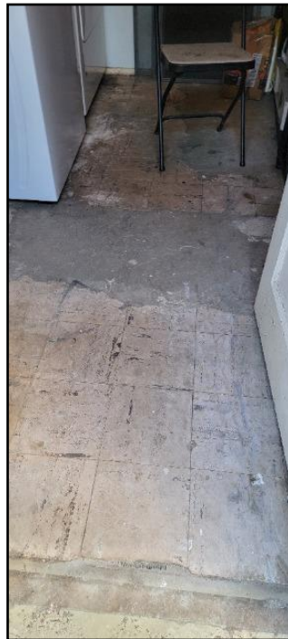
Possible asbestos (not tested)
