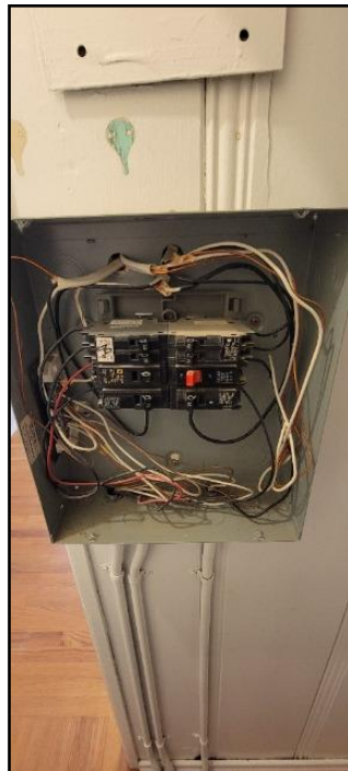
Possible unapproved breakers in this panel
