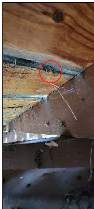
Fungus damage in deck boards
