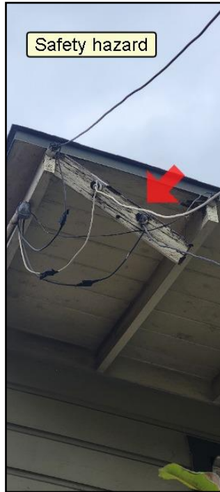
Wires not anchored correctly
