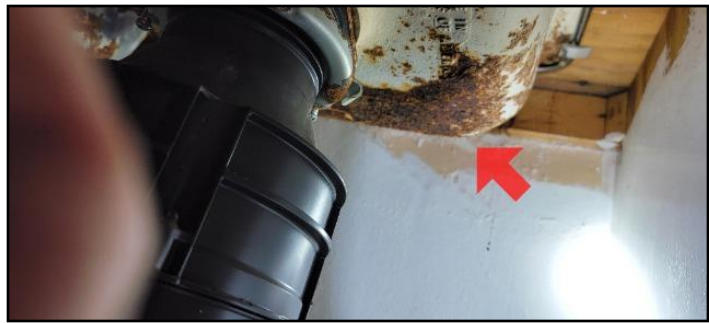
Rust under sink
