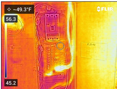
No abnormal heat in electric panels
