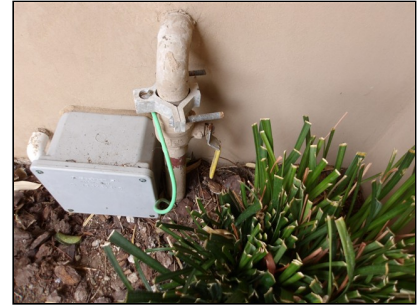
Multiple water shut off valves
