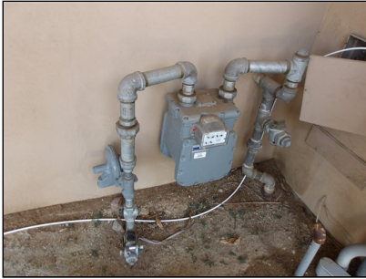
Gas front exterior
