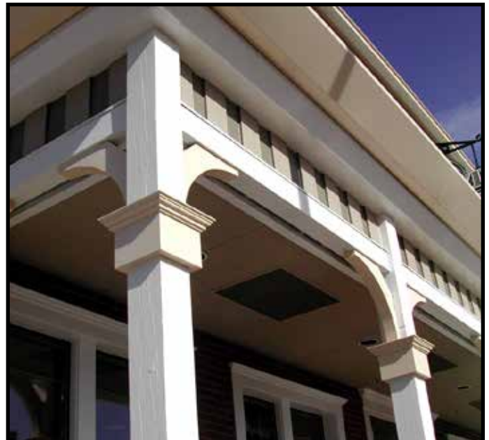
Appropriately sized and functional column
